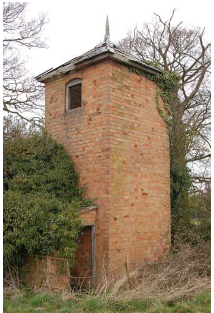
A small red brick, 19th century, hydraulic pump building in Hindlip. Photograph © Worcestershire County Council.
