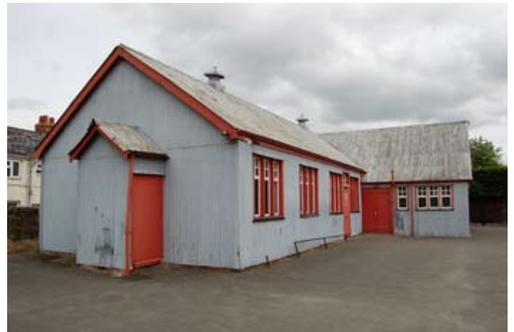
Early 20th century corrugated iron parish hall in Kempsey. Photograph © Worcestershire County Council.
