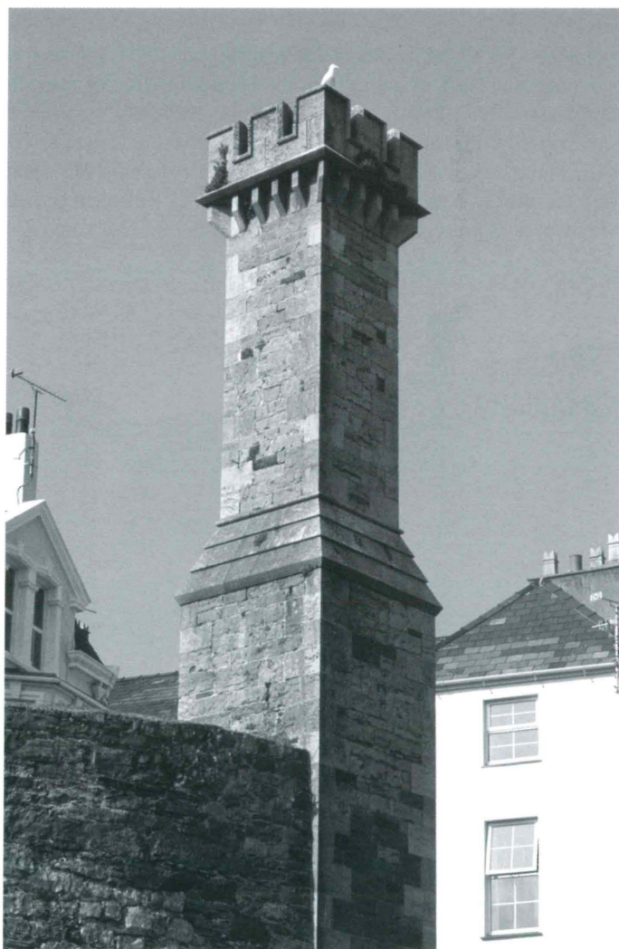
Fig. 11. Boiler house stack on the sea wall, part of the former hot baths and built by 1828, probably by Hansom and Welch, architects of York.
