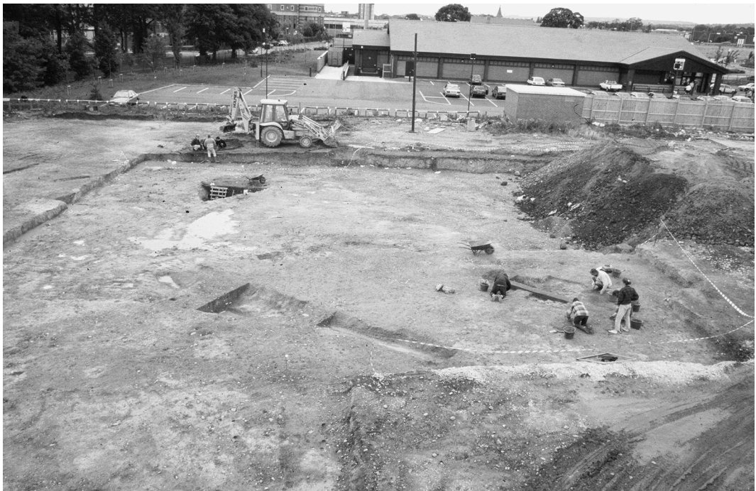
Fig. 2. General view of the 1994 excavations in Area 1 with work proceeding in the area of the corn-drying kiln.
