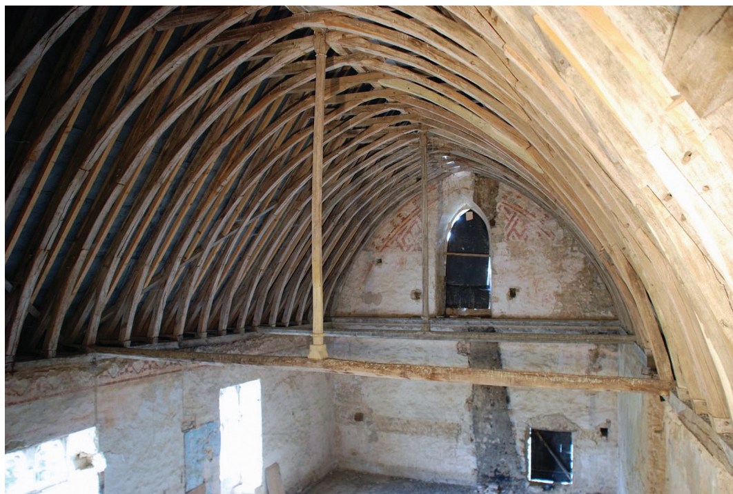
Fig. 16. Asnières-sur-Vègre (Sarthe). The eastern upper hall with its carpentry of 1293–95. This is a very good example showing clearly the how the delicate tie beam, whose function is to prevent the rafters from spreading, is supported by the fine king-post; they are thus both in tension. Vestiges of the once elaborate mural decoration is evident in the plasterwork. Photograph: J. Mastrolorenzo.
