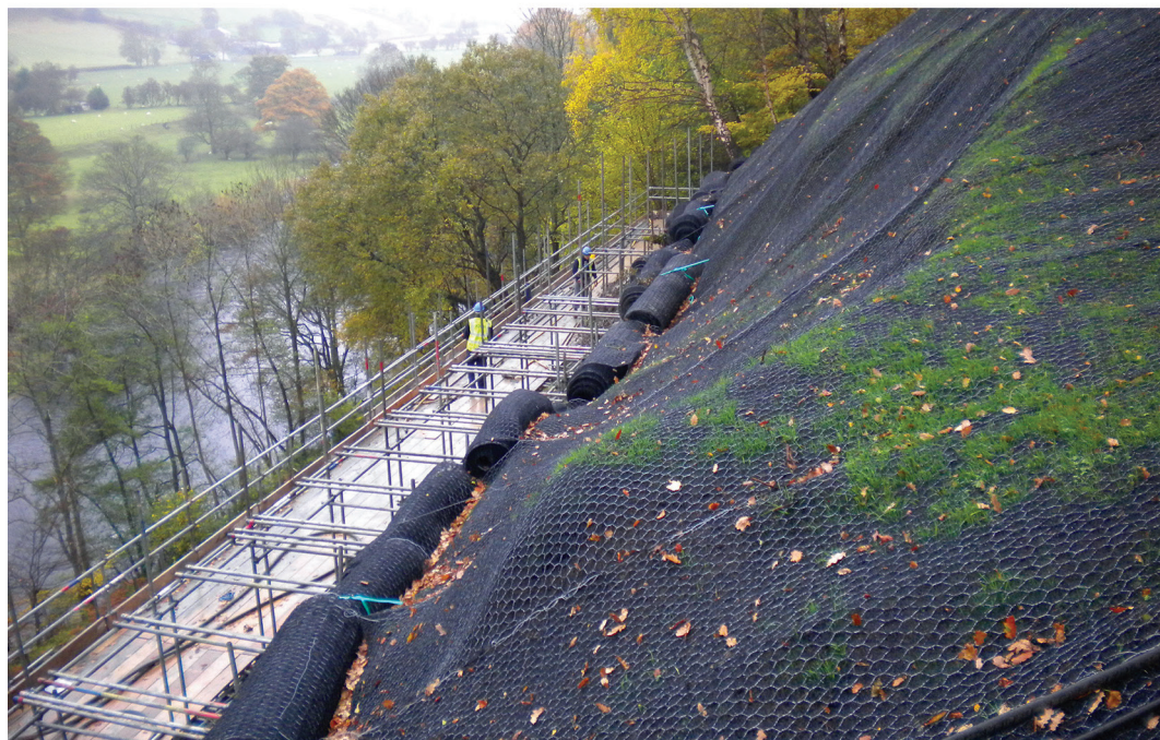
Fig. 7. Owain Glyndŵr's Mount, Glyndyfrdwy, after ( above ) and during ( below ) conservation. © Crown copyright: Cadw – Welsh Government.
