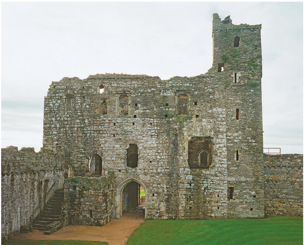
Fig. 5. Rear elevation of the great gatehouse at Kidwelly Castle. © Crown copyright (2017) Welsh Government.
