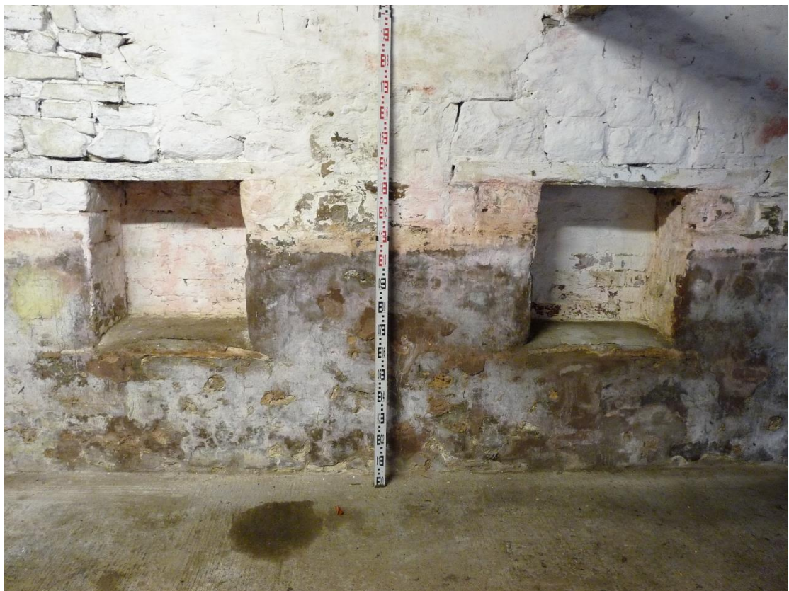
Plate 16: blocked feedholes on north wall (east end) of Building 2 from the north
