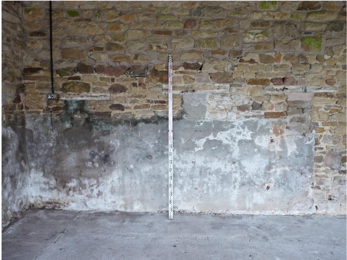
Plate 13: blocked vents on the north wall (west bay) of Building 1
