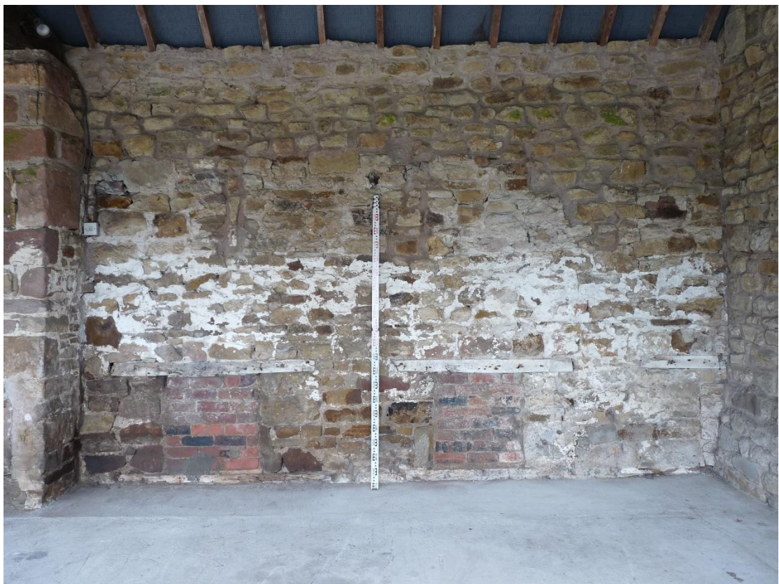
Plate 12: blocked feed-holes on north wall (east bay) of Building 1
