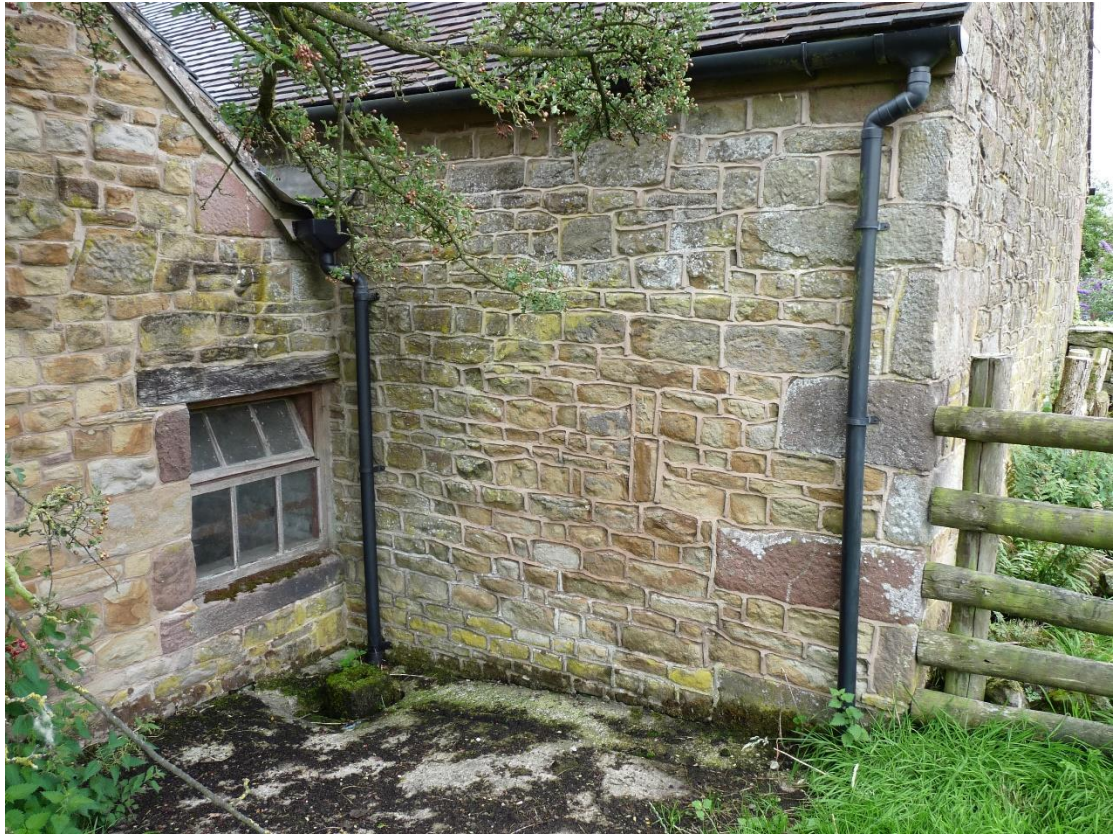
Plate 5: external junction between Buildings 1 and 2, from the north-west, with blocked breather on north wall of Building 1
