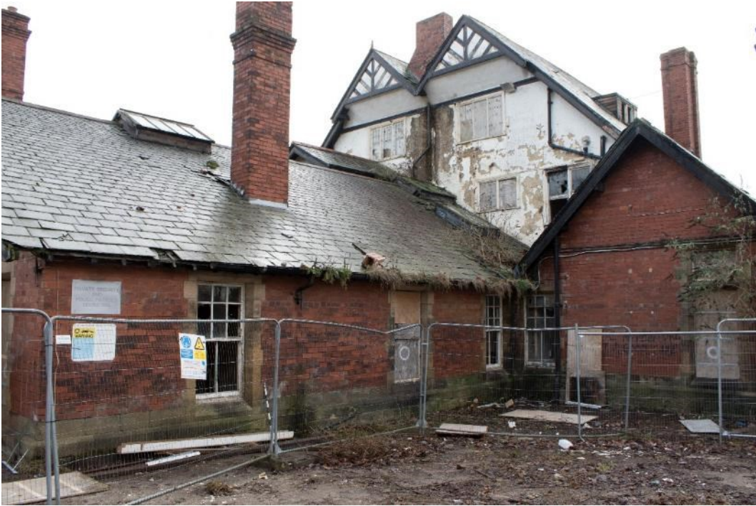
Photo 95: West elevation of north block and north elevation of central block, facing south (1796_095.TIF)
