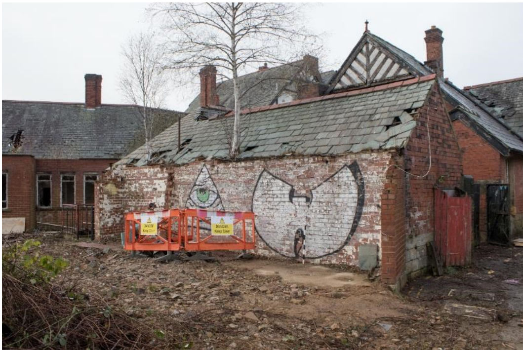
Photo 84: Partially demolished extension to the east of the service range, facing west (1796_084.TIF)
