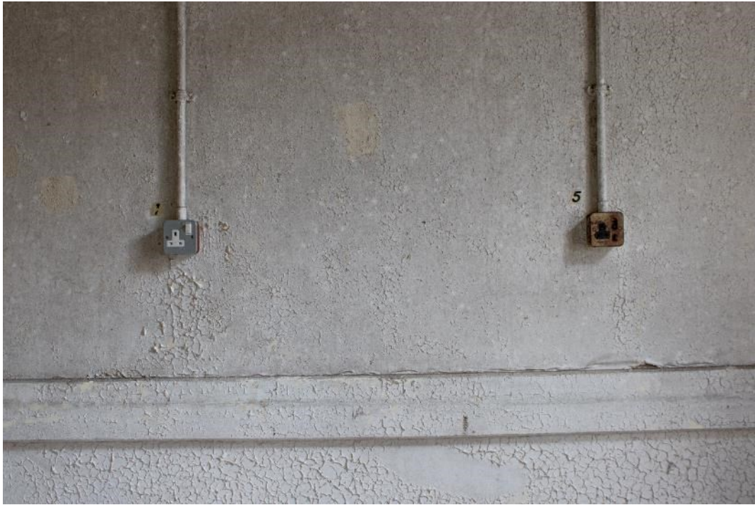
Photo 135: Room 6 power sockets, facing north-west (1796_135.TIF)
