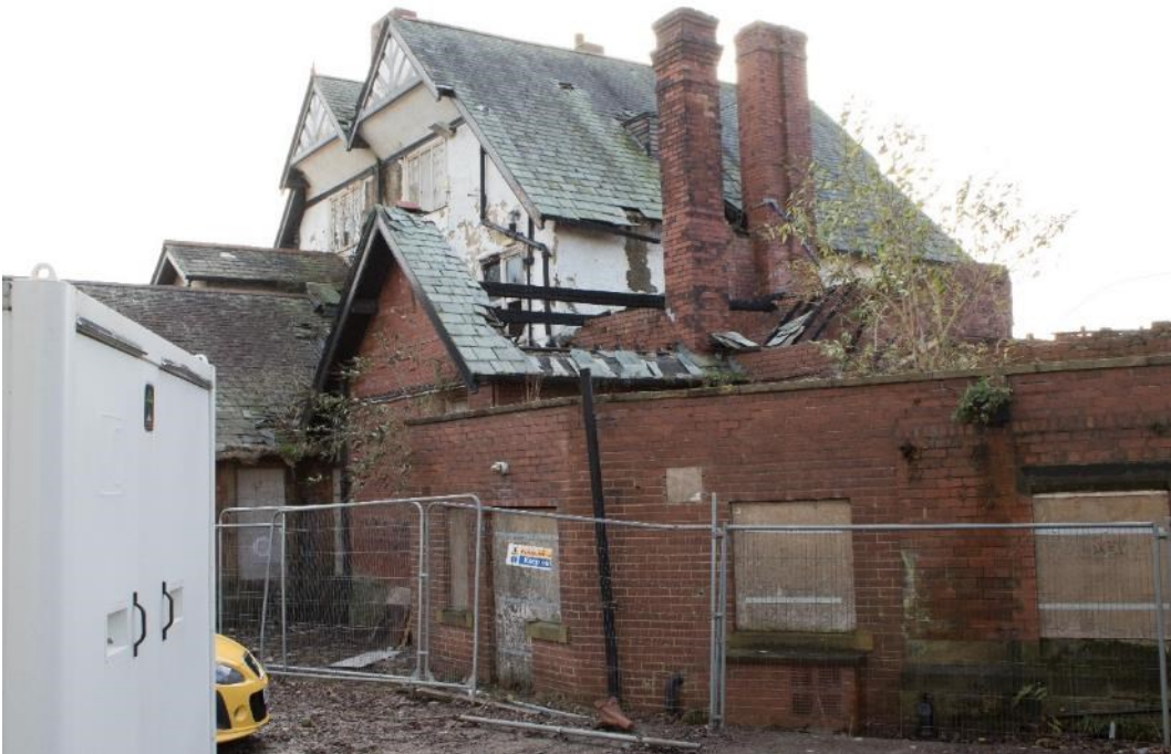
Photo 56: Rear of the west wing, wash block and central block, facing south-east (1796_056.TIF)
