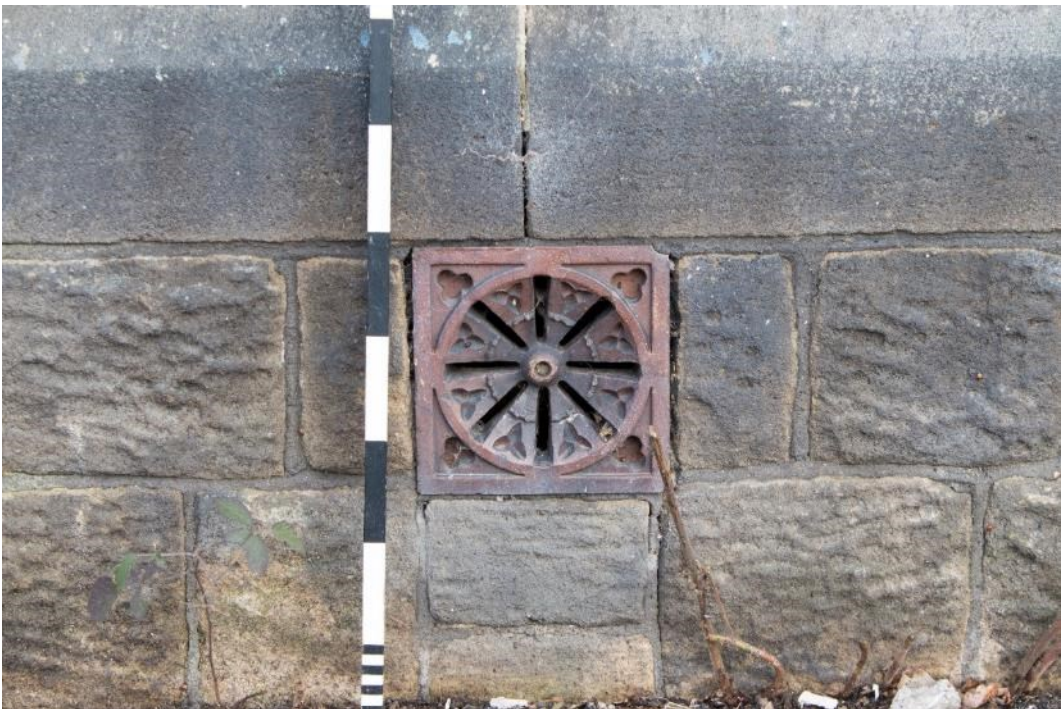
Photo 26: Ventilation grill, facing north-east (1796_026.TIF)
