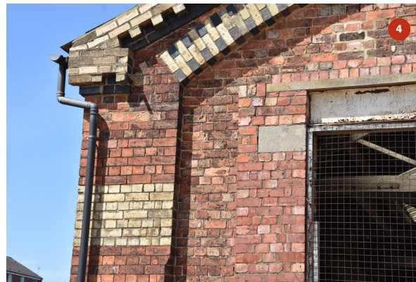
Detail of south elevation showing polychromatic brickwork and padstone supporting the steel lintel to the enlarged opening
