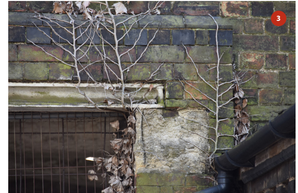
Detail of north elevation showing the west support to the lintel over the wagon entry opening
