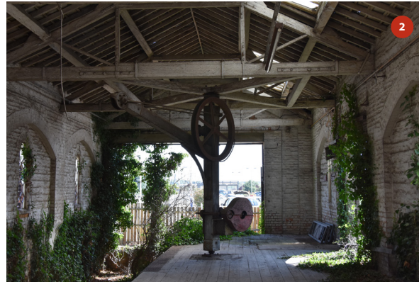
South elevation and jib crane
