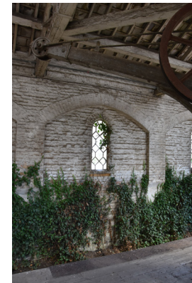
Bay 5 and southern jib crane
