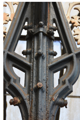
Detail of bolts and strapping joining brackets together around central column (close up of photo 4)
