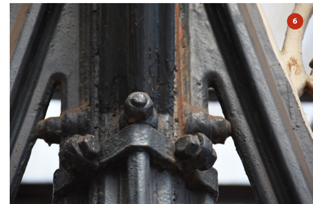
Detail of local iron strapping joining brackets together (close up of photo 5)
