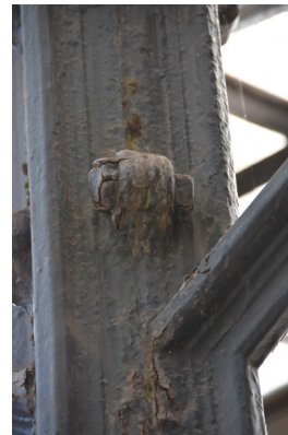
Detail of bolts joining brackets together around central column (close up of photo 4)
