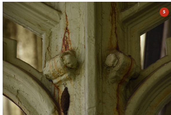
Detail of bolts joining brackets together around central column (close up of photo 4)
