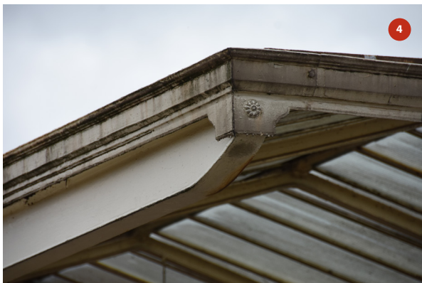
Detail of end bay of northern end of platform 1 canopy (close up of photo 4)
