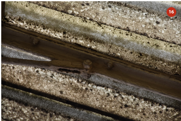
Detail of connection between top chord of tied rafter and horizontal tie member
