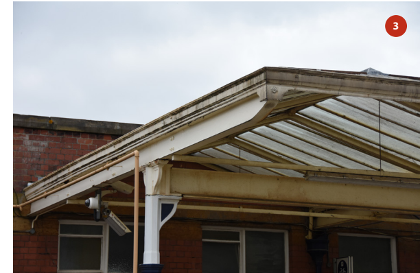
Detail of end bay of northern end of platform 1 canopy (close up of photo 2)
