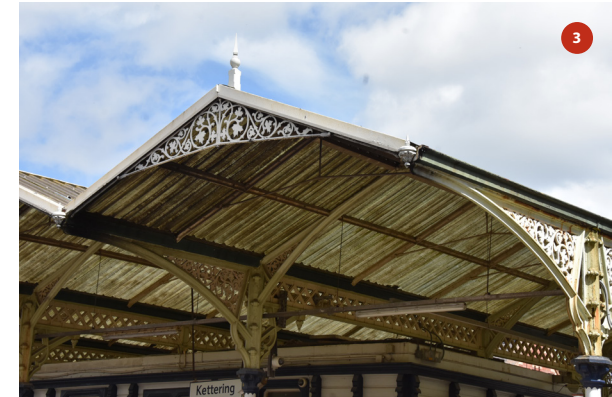
Southern bay of platform 3 canopy seen from the southern end of platform 4
