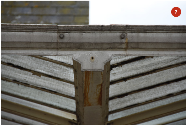
Detail of missing end detail taken from platform 2
