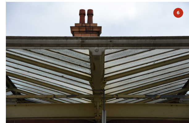
Detail of elevation of platform 1 canopy, seen from middle of platform 2 (close up of photo 5)
