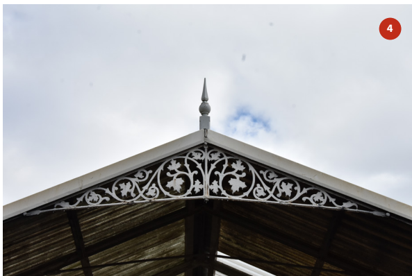
Detail of southern end bay of platform 3 canopy seen from the southern end of platform 4
