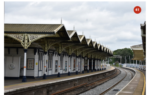
Platform 2 canopy seen from the southern end of platform 1 (close up of photo 40)
