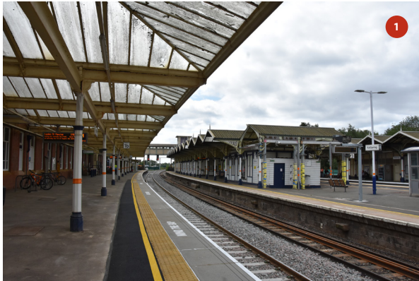
Platform 2 canopy looking north-west from the southern end of the canopy on platform 1
