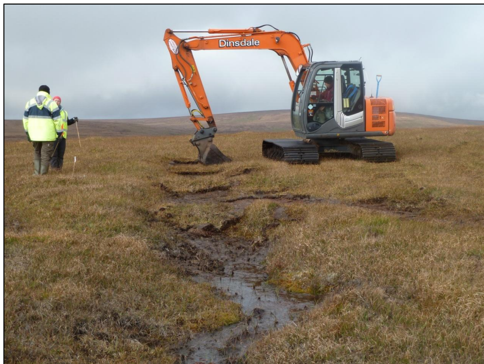
Plate 3 Erosion gully with multiple blocks.
