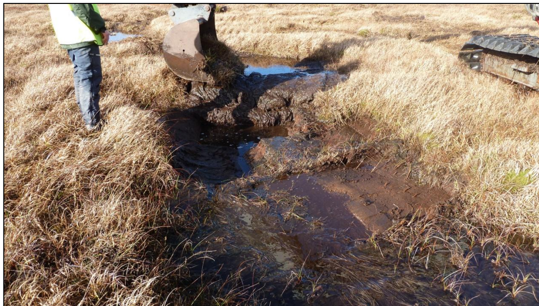
Plate 5 Erosion gully during block construction (note removal of peat island in Plate 4 and reprofiling of gully sides).
