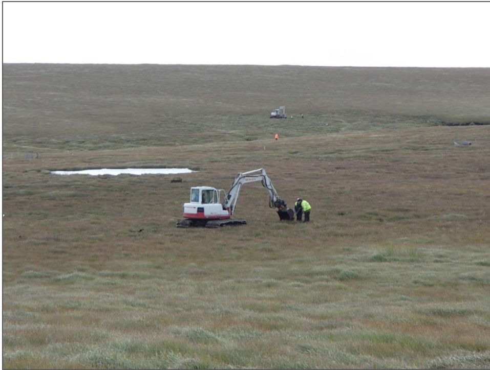
Plate 5 Restoration work on the north side of the pond in area 1, looking south towards restoration work in Area 2.
