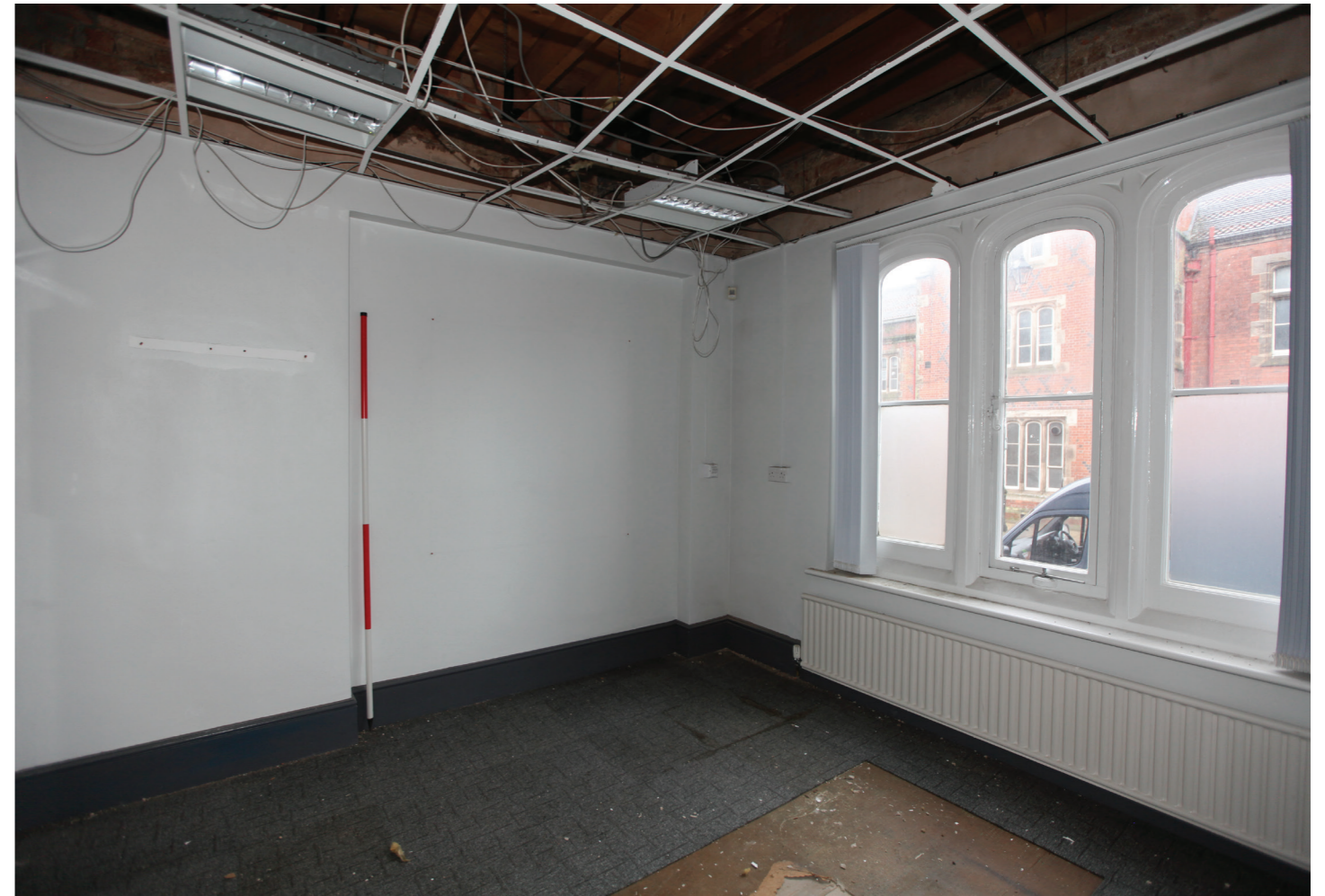
Room G2 - G_006.jpg - No. 1 Winton Square. Former Dining Room, looking towards the stairwell wall, with alcove, probably the enlarged location of the former doorway. It is possible that when the extension was built the original doorway into the Dining Room was simply widened to create a more open and spacious link with the staircase hall to walk through. There are no indications that the corridor wall to the left of this photo was created until recently (late 20th century).
