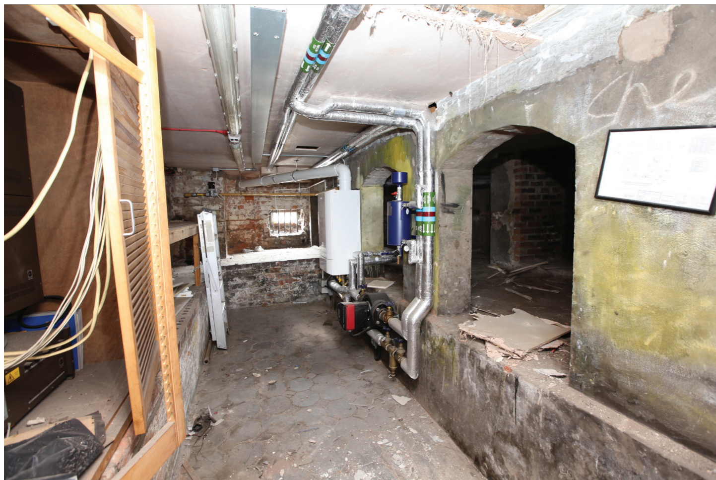
Room B18 - B_038.jpg - BASEMENT - Heated space with ornate tiled floor and baulks around the perimeter. Brick-arched dividing wall provides support for a timber floor above. This space was probably heated to provide secondary underfloor 'warm air' heating for the large Living Room above.
