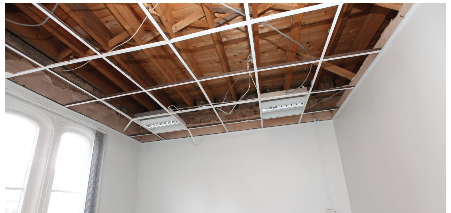
Room G2 - G_007.jpg - No. 1 Winton Square. Inserted modern ceiling & joists to ground floor. Modern partition to the right.
