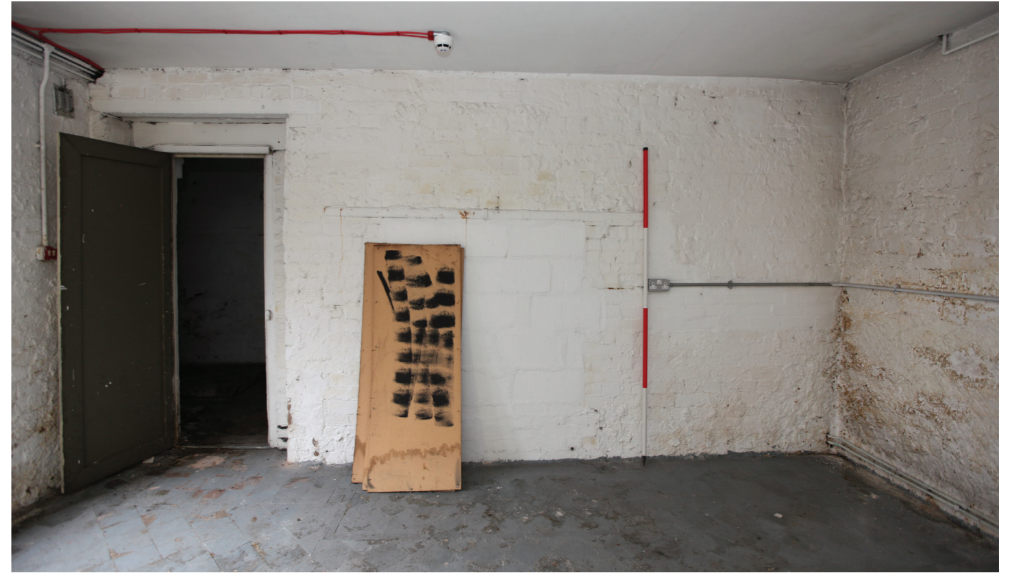
Room B4 - B_019.jpg - The former kitchen to No. 1 Winton Square. The door to the left led to the garden via a flight of steps but was retained when the extension was added and now leads to the coal cellar and storage areas. The former kitchen range was removed and the hearth blocked up, central to this wall. Red clay tiled floor in-situ throughout this space. Modern plasterboard soffit.
