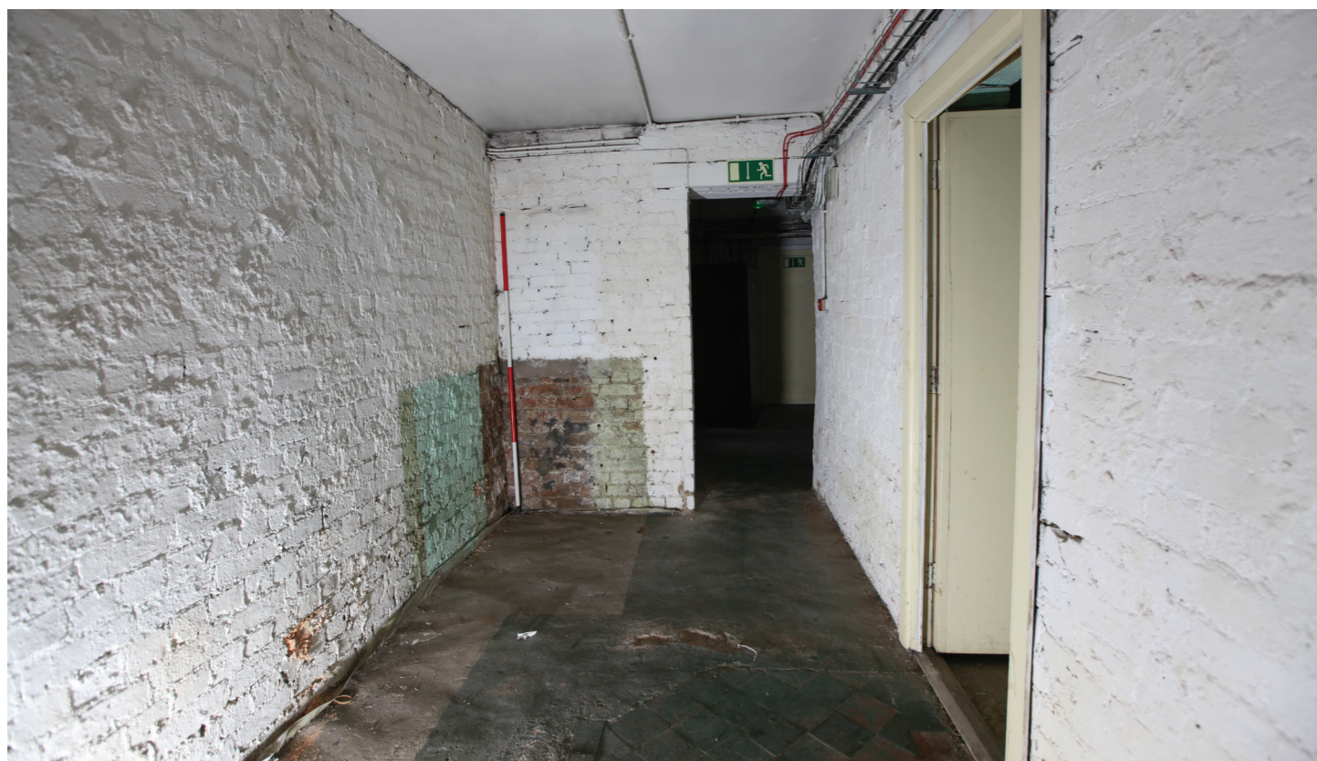
Room B5 - B_017.jpg - Former stairwell to No. 1 Winton Square. The doorway in the distance is a modern alteration. The footprint of the staircase and the direction of the rise can be seen in the floor detail, with concrete for the base of the stair and tiles elsewhere.
