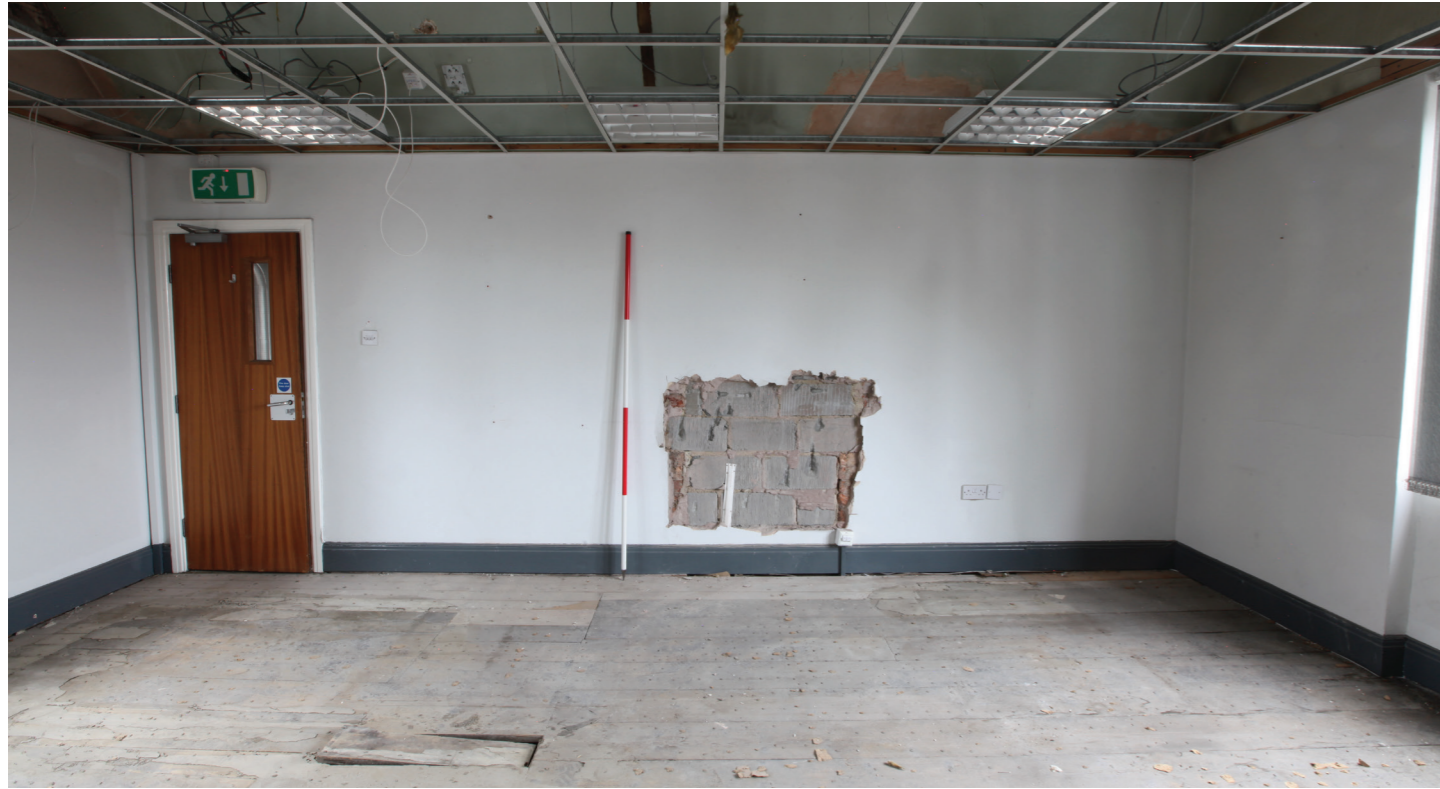
Room F12 - F_001.jpg - Internal wall to first floor pair of bedrooms (No. 3). The 'breezblock' panel reveals a former doorway which entered the second bedroom off the stairwell. The current arrangement has removed this access, indicating that the staircase may have been turned.
