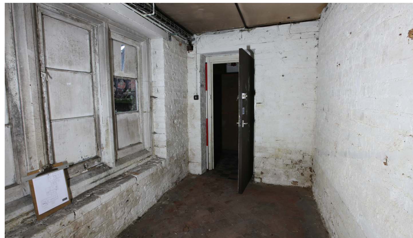
Room B7 - B_014.jpg - Former probable pantry (unheated space). The brick partition to the left is the original one dividing the scullery from the pantry on plan. Windows provide plenty of light for working at this semi-basement level. Red clay tiled floor in-situ.
