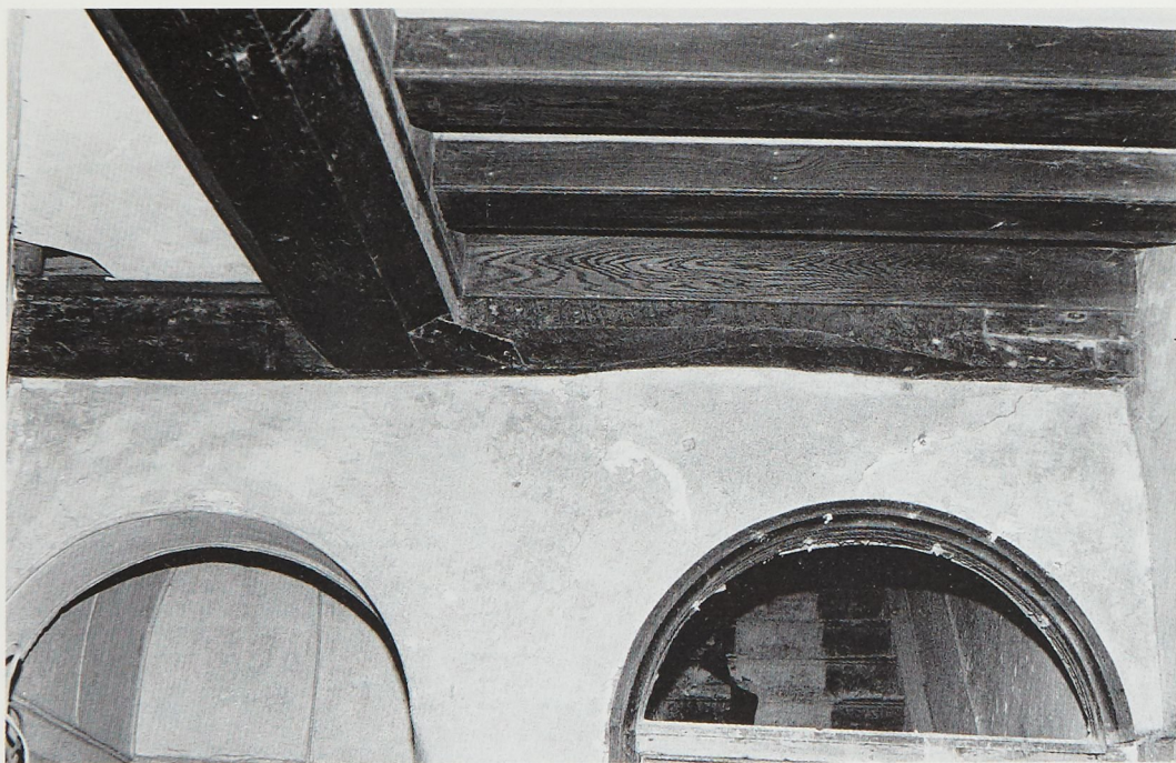
Plate XVIII Extension of central room transverse joist showing position of former chamfer stop and modern softwood beam.
