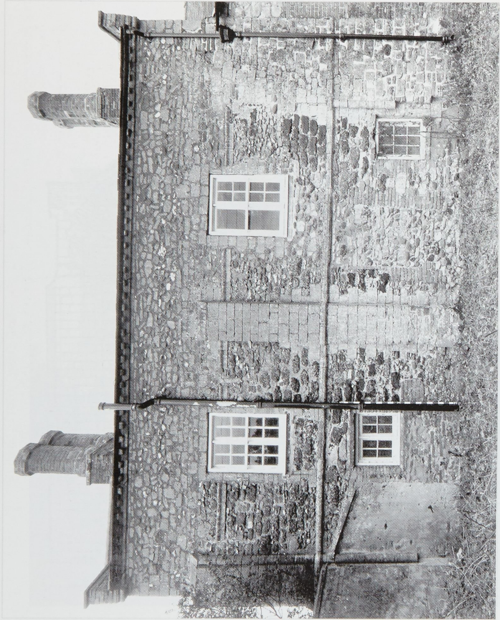
Plate 2. The north wall of Winnold House The buttresses and string courses remain largely intact, although only the lower external jambs of one upper window (upper left) remain in situ . David Stevens 1993.
