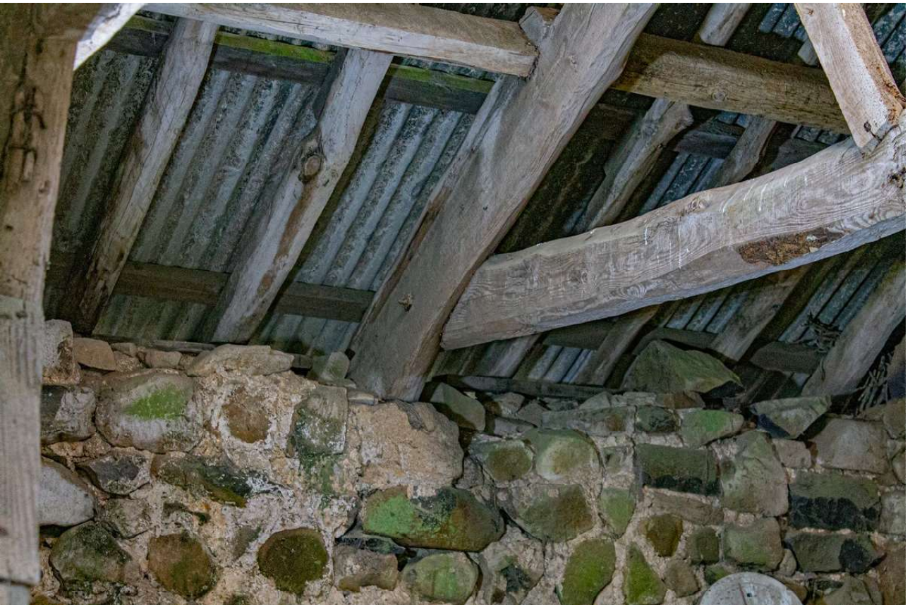
Plate 54 (51): Barn B1, Building B (Barn), detail of the rafter of the timber roof truss resting over the north-west wall and showing the bolting of the tie beam, from the south
