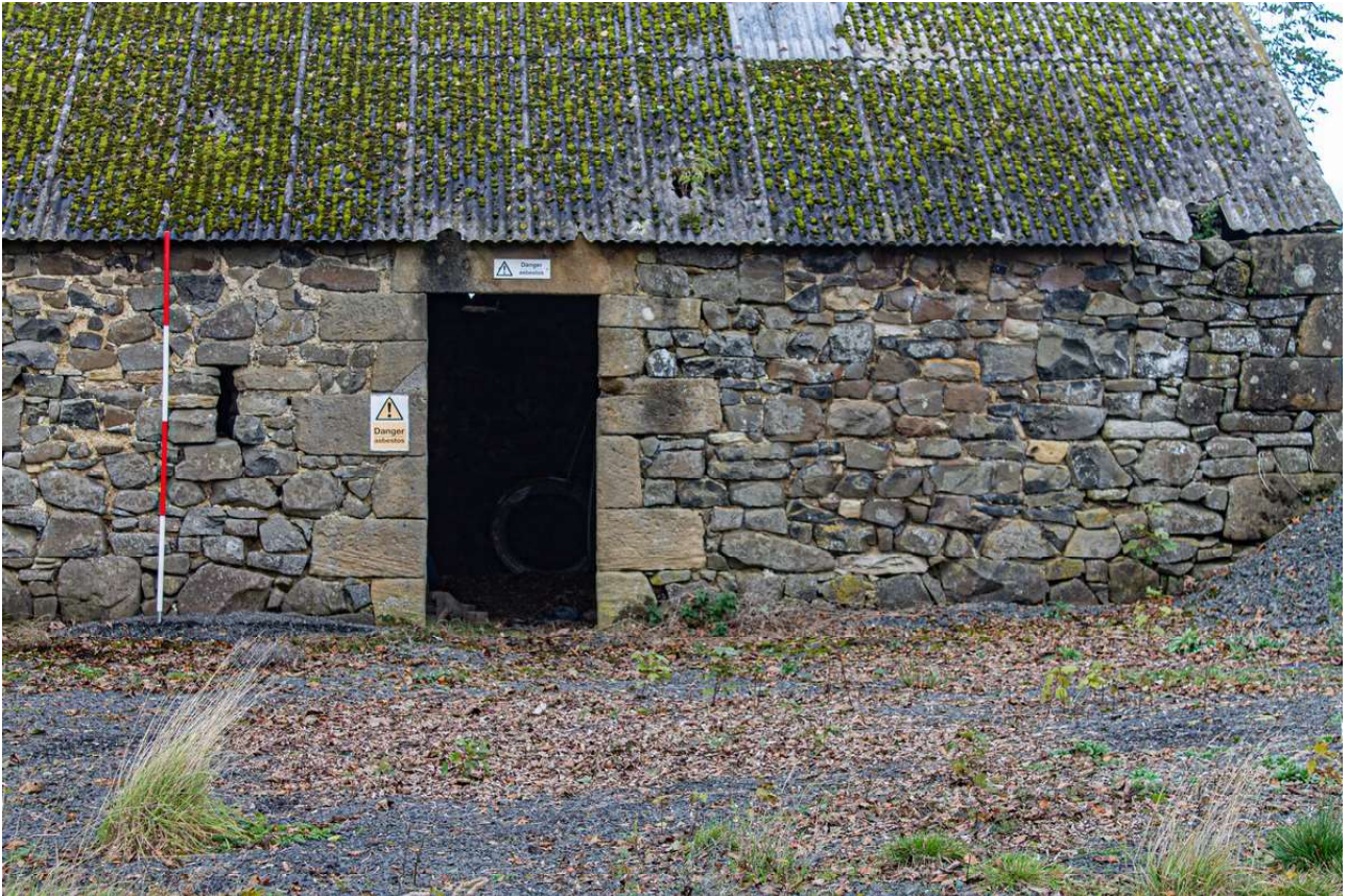
Plate 31 (31): Building B (Barn), detail of the entrance into Barn B1 and the adjacent slit window in the north-east end of the south-east elevation, from the south-east
