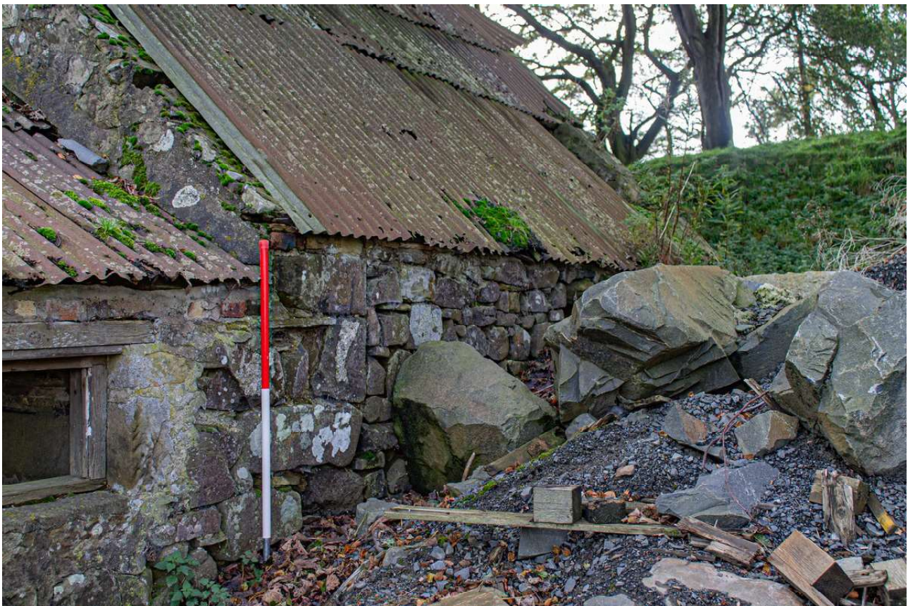
Plate 44 (46): Building B (Barn), general view of the north-west elevation of Barn B5, from the north
