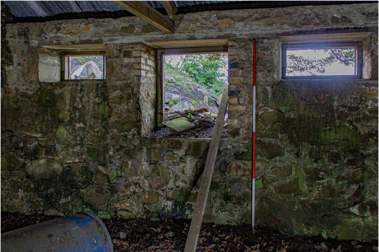
Plate 71 (71): Building B (Barn), Barn B4, detail of the inserted openings in the north-west wall, from the SSE
