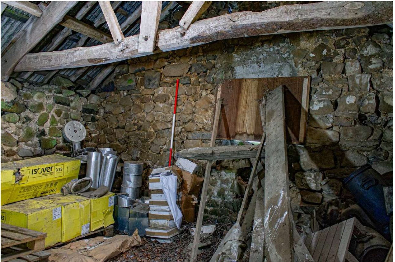
Plate 50 (49): Building B (Barn), Barn B1, general view showing the boarded window in the north-east elevation, from the south
