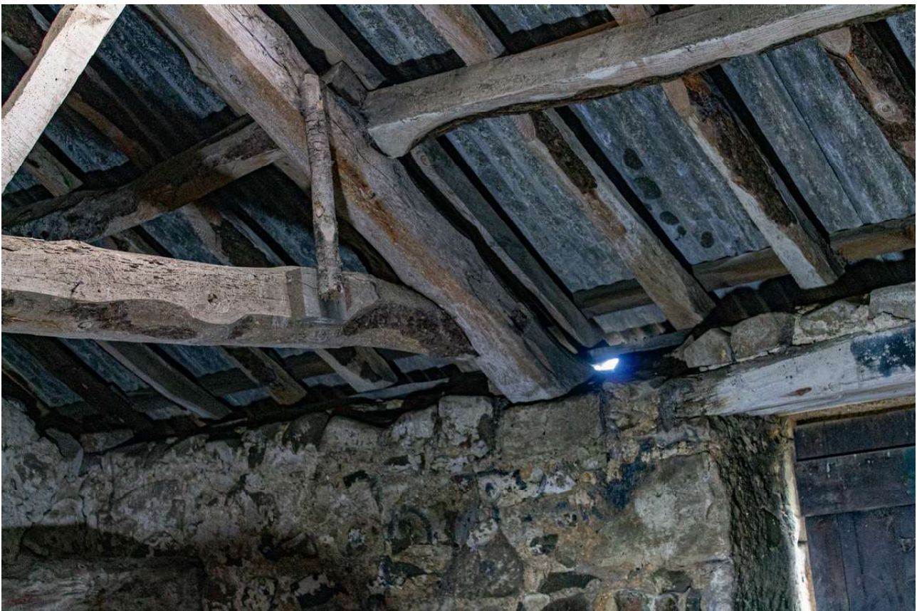
Plate 64 (61): Building B (Barn), Barn B2, detail of the rafter of the north-east timber roof truss as it sits over the south-east wallhead, from the west
