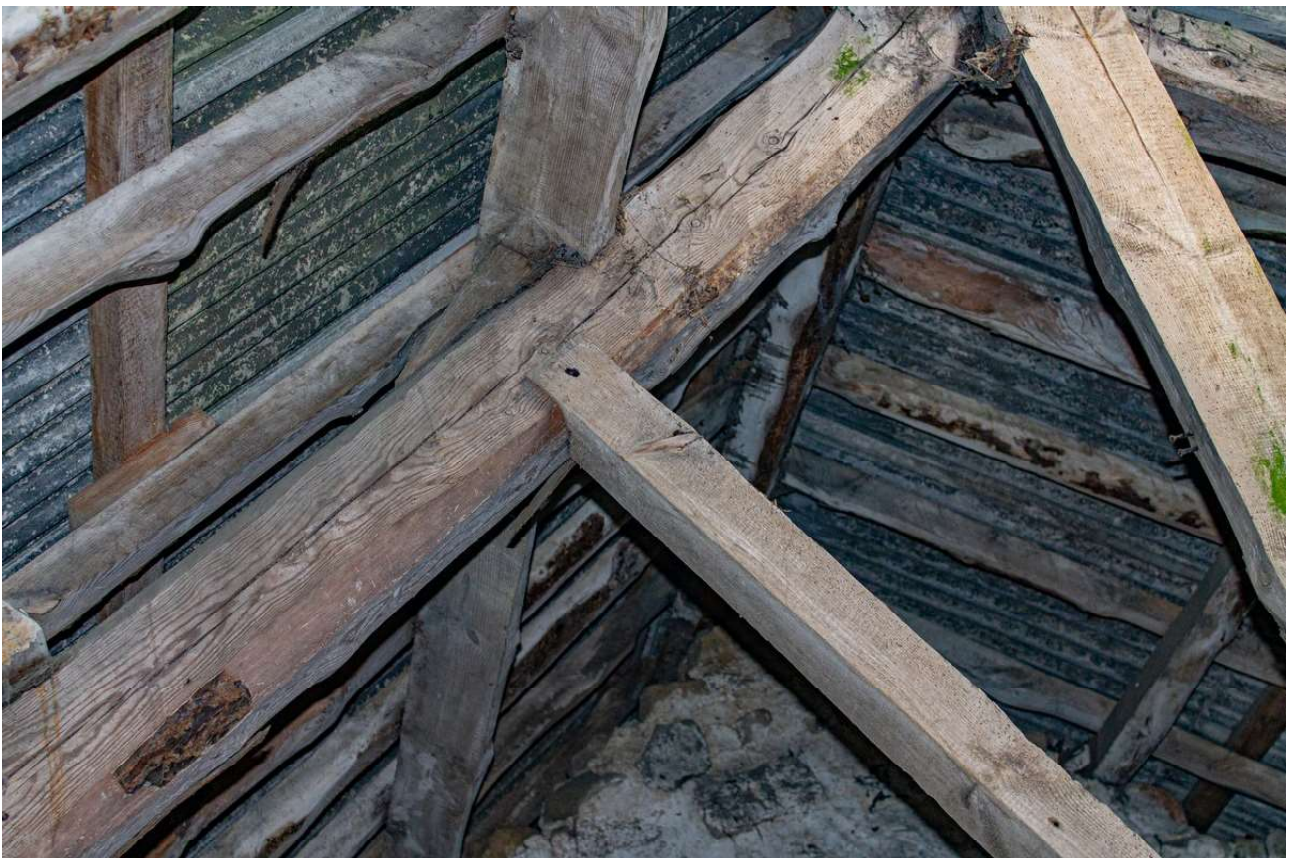
Plate 66 (64): Building B (Barn), Barn B2, detail of the strut slotted into the rafter of the north-east timber roof truss on north-west side, from the south-west
