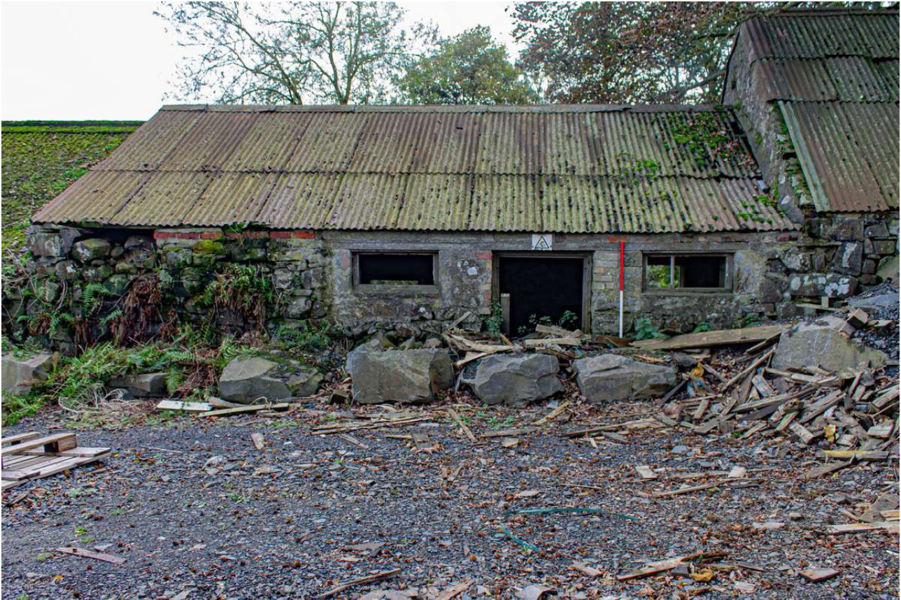
Plate 41 (43): Building B (Barn), general view of the south-west side of the north-west elevation showing the inserted windows in Barn B4, from the north-west
