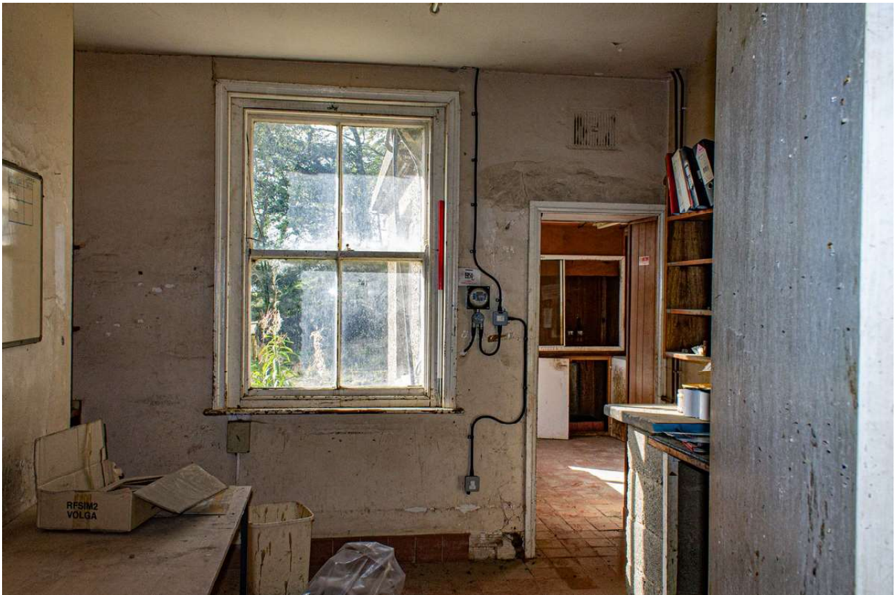
Plate 24 (24): Building A (Cottage), general view of the south-west elevation of Room A6, from the north-east
