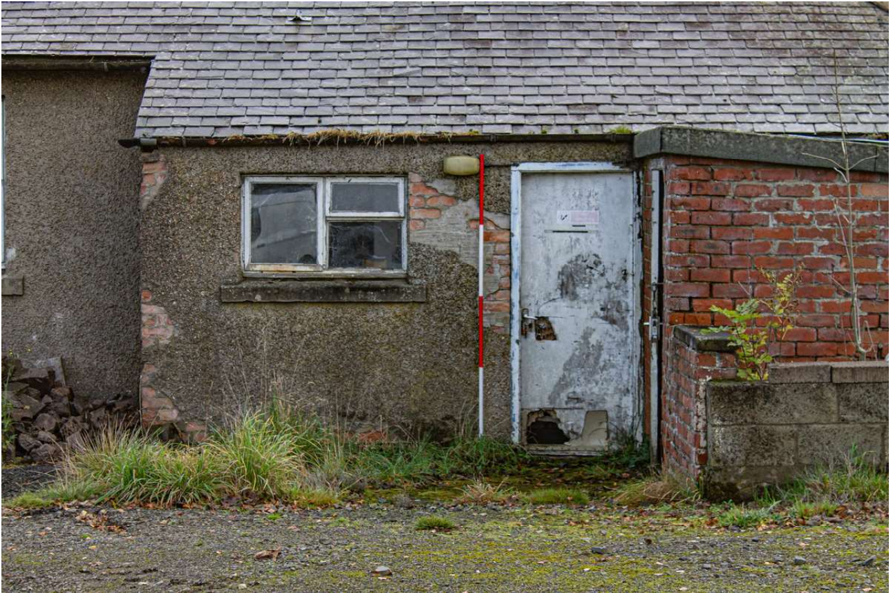
Plate 7 (02): Building A (Cottage), detail of the back door and adjacent window in the north-west elevation, from the north-west
