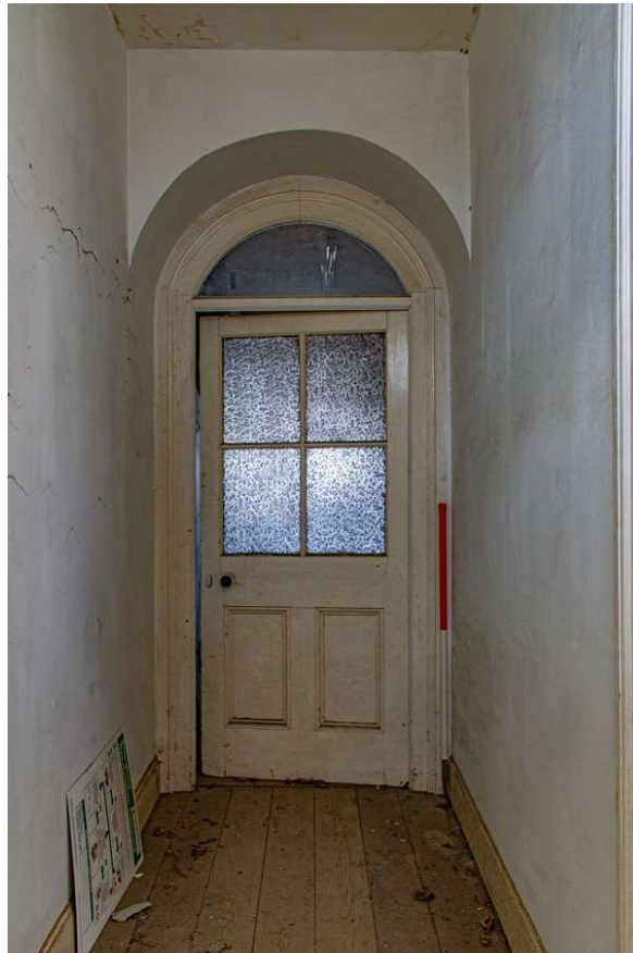
Plate 15 (15): Building A (Cottage), detail of central doorway between Rooms A1a and A1b, from the south-east
