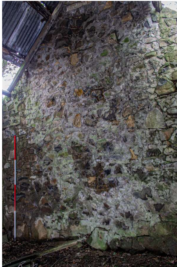
Plate 77 (77): Building B (Barn), general view of the south-west elevation from the NNE
