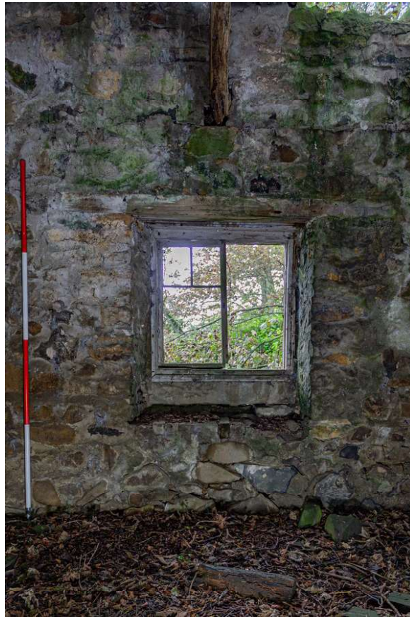
Plate 75 (75): Building B (Barn), Barn B5, detail of the window in the south-east elevation, from the north-west
