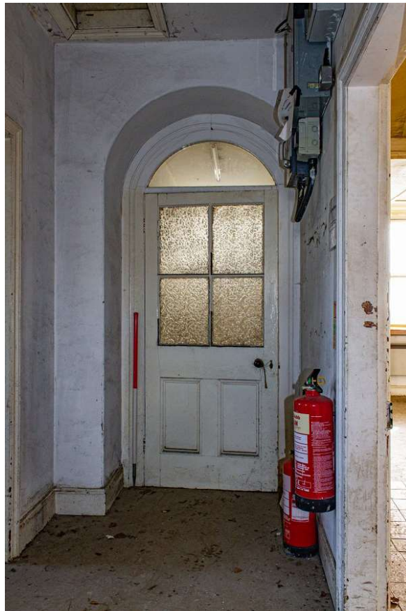
Plate 16 (16): Building A (Cottage), detail of central doorway between Rooms A1a and A1b, from the north-west
