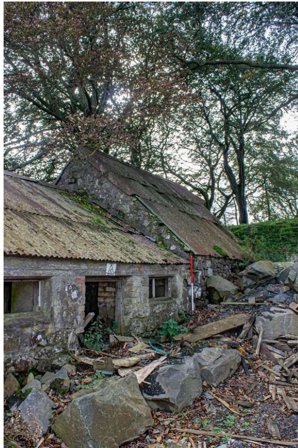
Plate 43 (45): Building B (Barn), general view of the south-west end of the north-west elevation, from the north
