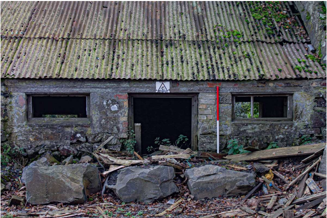
Plate 42 (44): Building B (Barn), detail of the inserted windows in Barn B4, from the north-west
