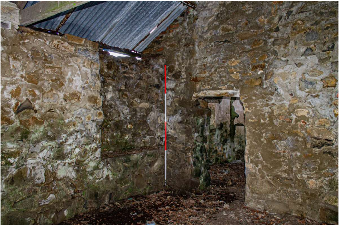
Plate 70 (72): Building B (Barn), Barn B4, detail of the north corner showing the rubble-blocked opening (left) and the doorway through to Barn B3 (right), from the south
