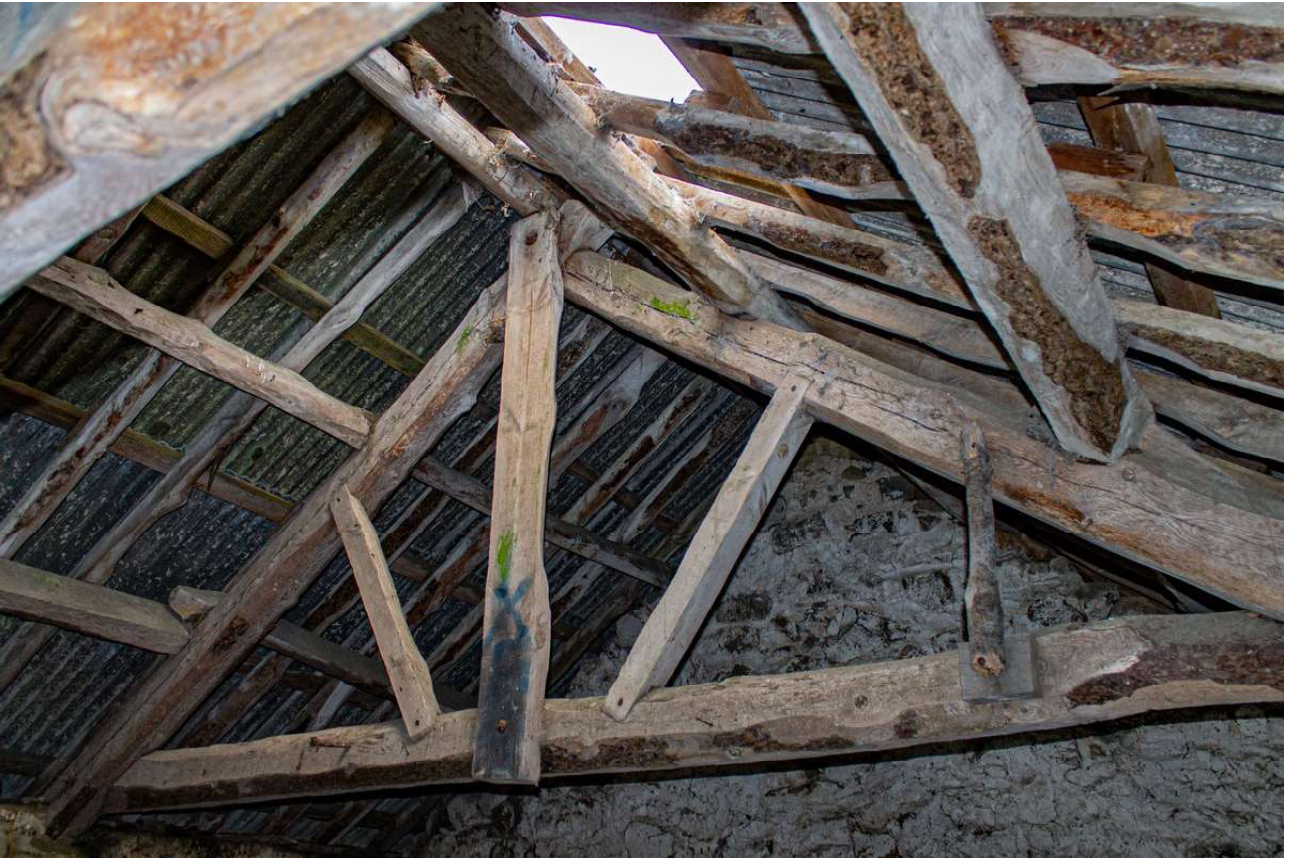
Plate 61 (66): Building B (Barn), Barn B2, general view of the north-east timber roof truss from the SSW
