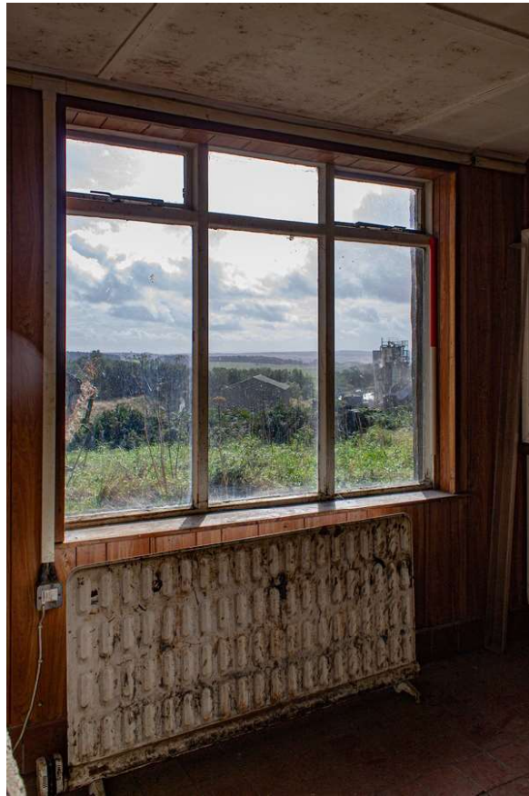
Plate 25 (25): Building A (Cottage), detail of window in the south-east elevation of Room A7, from the north
