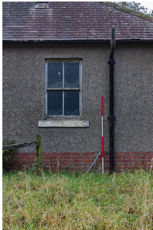
Plate 10 (05): Building A (Cottage), detail of the sash window in the north-west side of the north-east elevation, from the north-east
