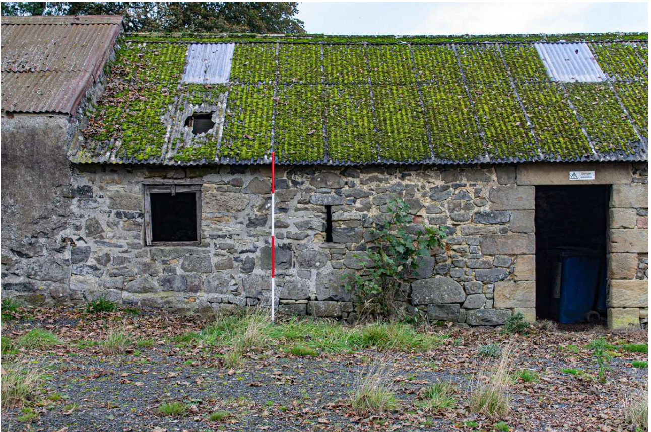
Plate 32 (32): Building B (Barn), detail of the door through to Barn B2 and the adjacent window and slit window in the north-east side of the south-east elevation, from the south-east
