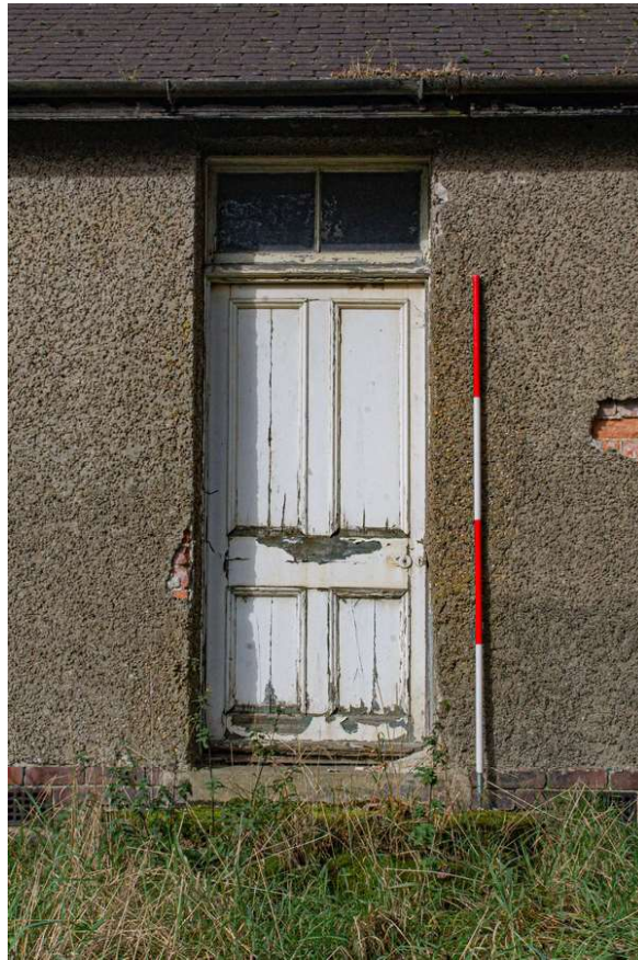
Plate 5 (07): Building A (Cottage), detail of the main entrance in the centre of the south-east elevation, from the south-east
