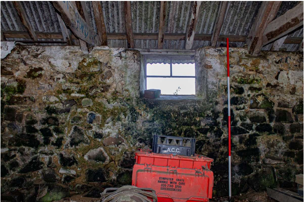
Plate 56 (55): Building B (Barn), Barn B2, detail of inserted window in the north-west elevation, from the south-east
