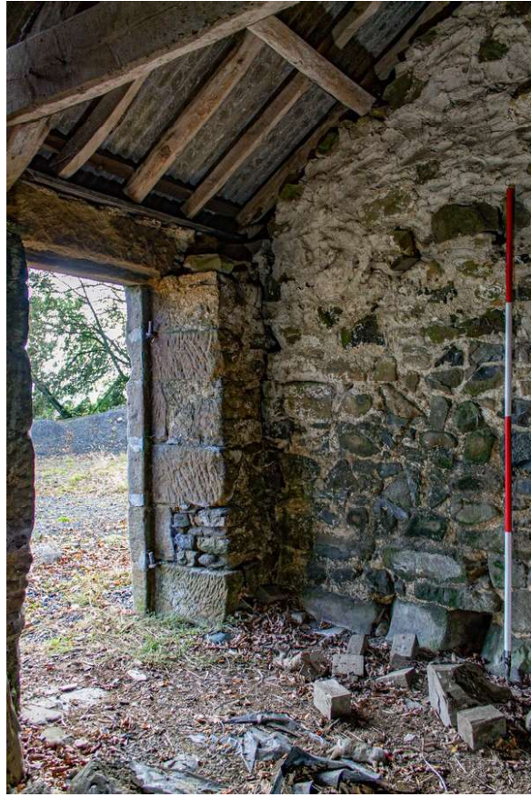
Plate 49 (54): Building B (Barn), Barn B1, general view showing the doorway in the south-east elevation, from the east
