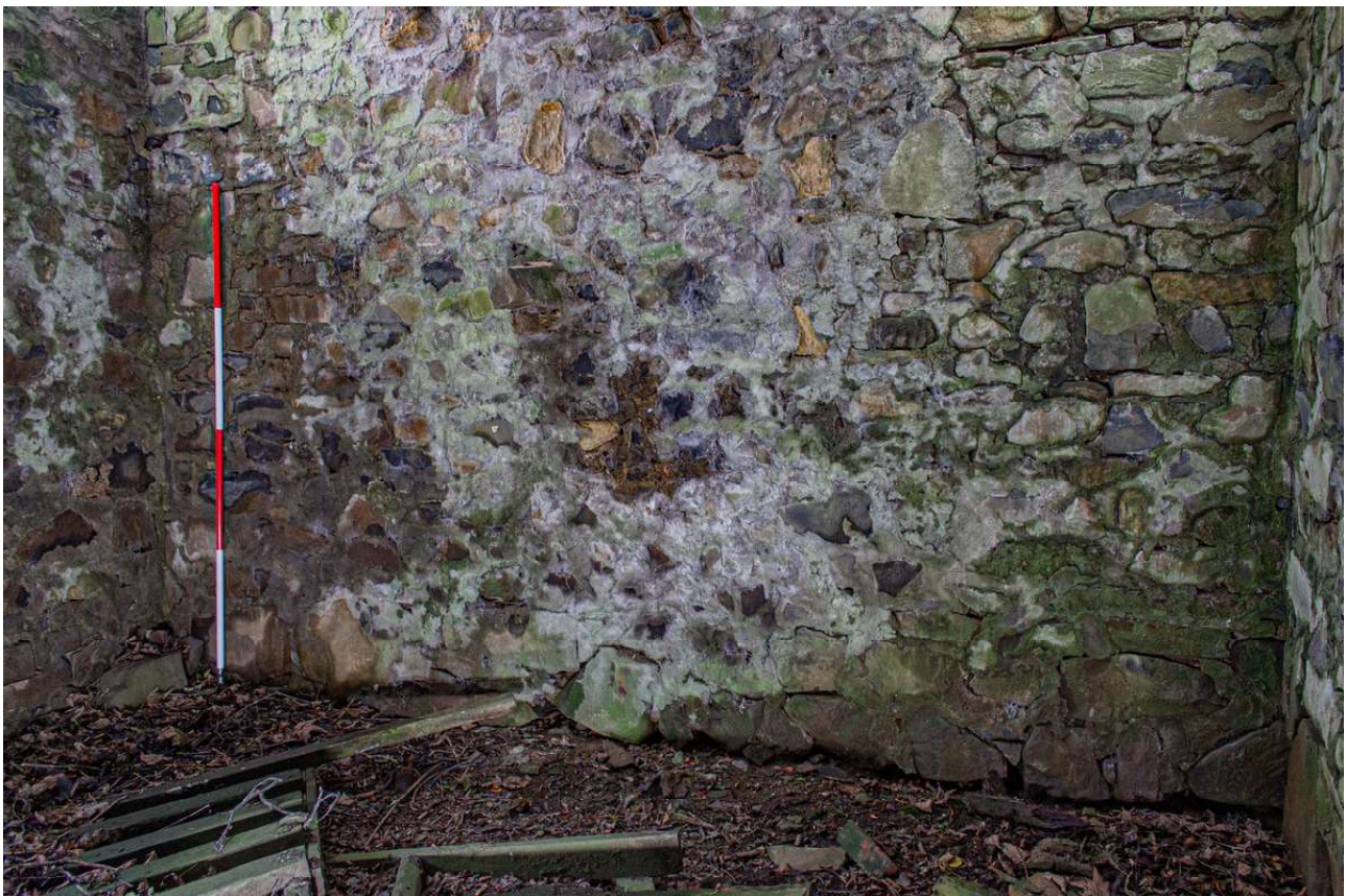
Plate 78 (78): Building B (Barn), detail of the base of the south-west elevation, from the NNE
