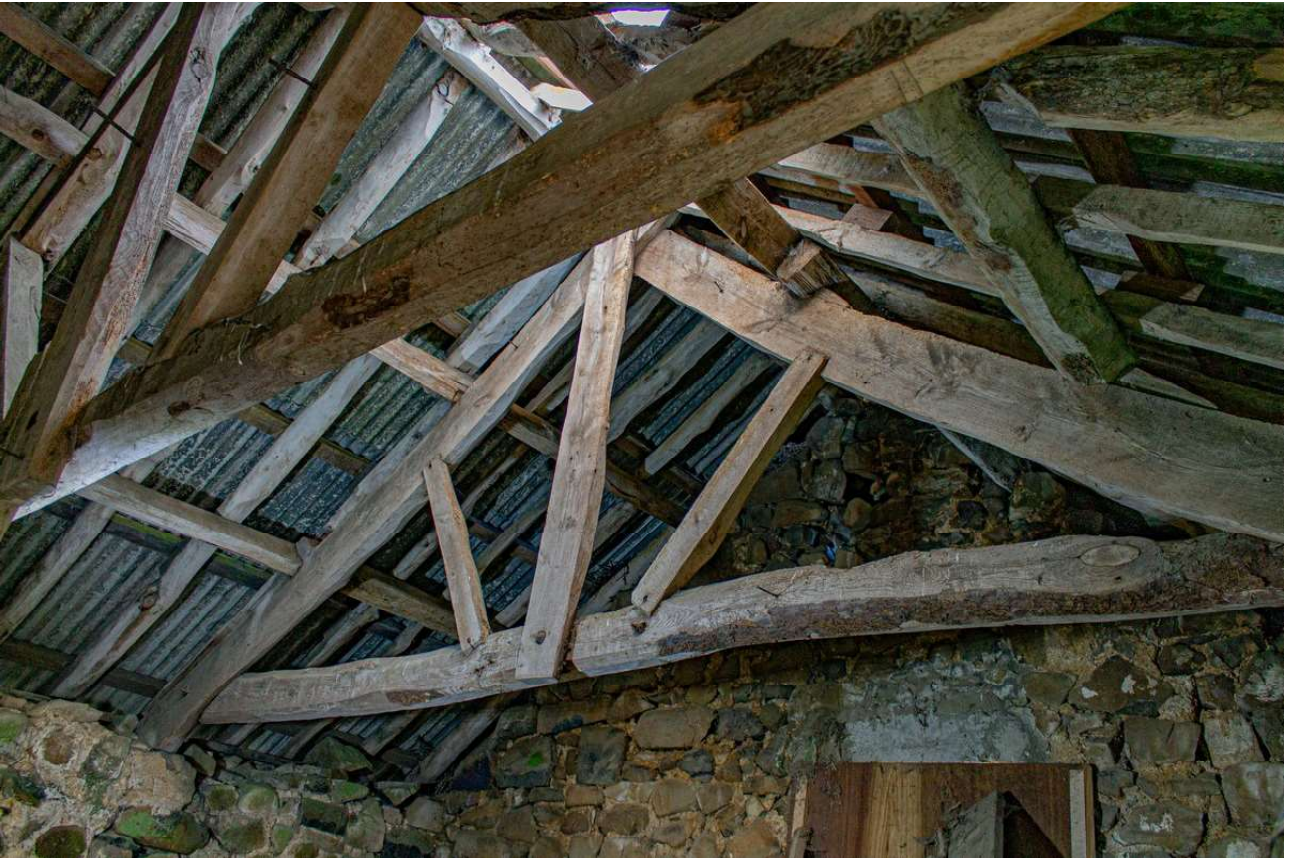
Plate 53 (50): Barn B1, Building B (Barn), general view of the timber roof truss from the south
