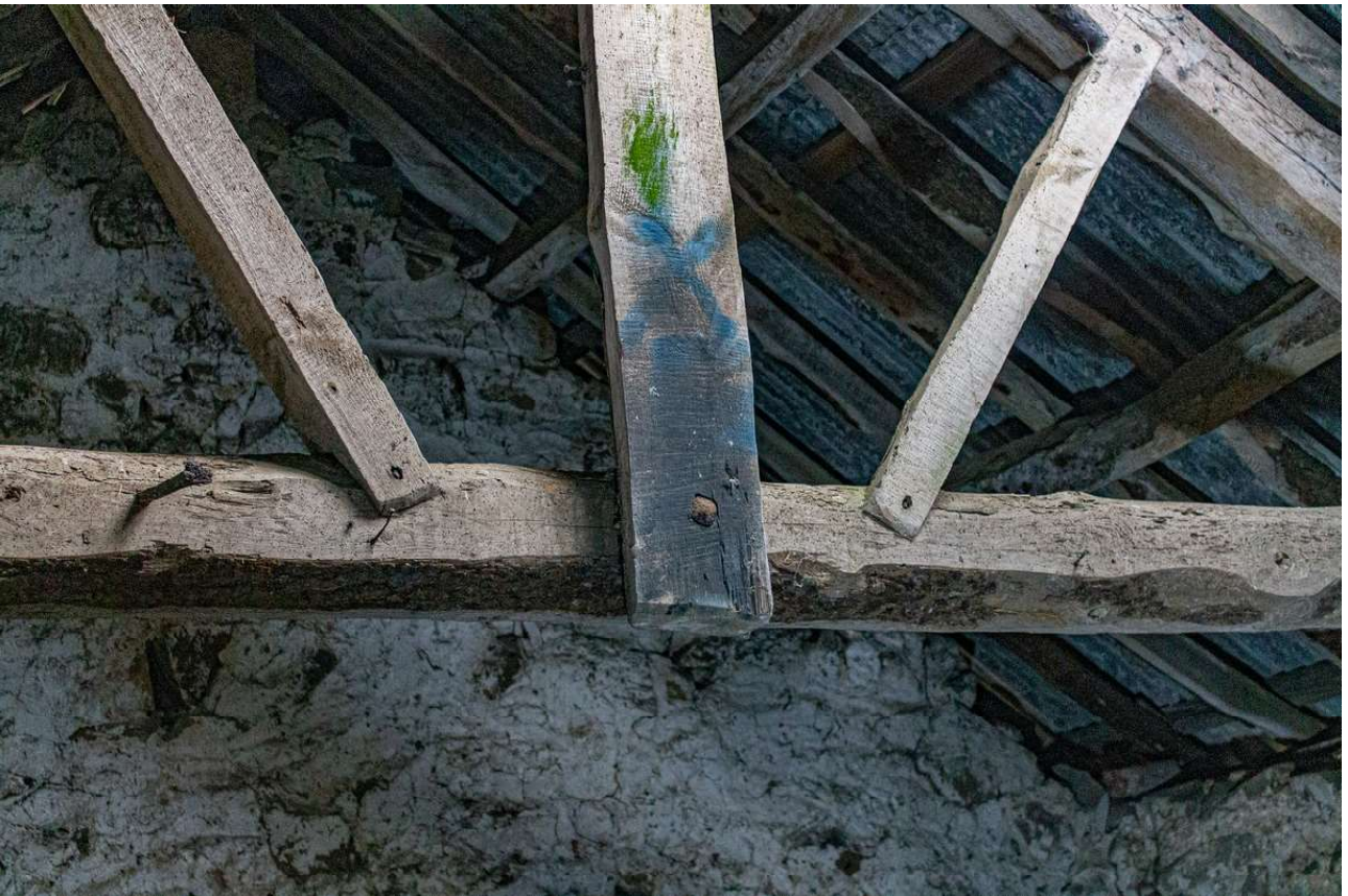
Plate 62 (60): Building B (Barn), Barn B2, detail of the bolt fastening the king post and tie beam in the north-east timber roof truss, from the south-west
