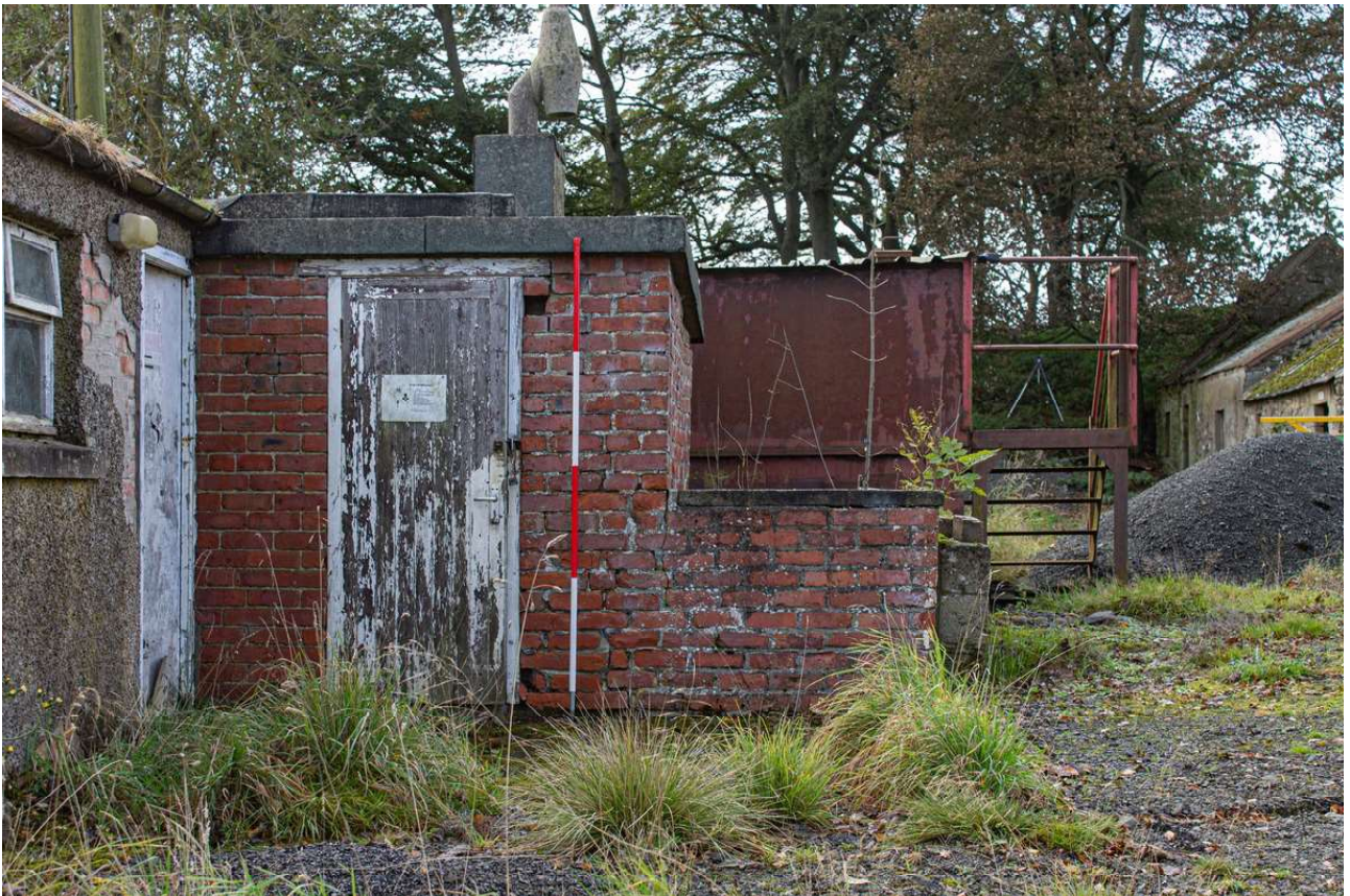
Plate 8 (03): Building A (Cottage), detail of the north-east facing side of the small brick lean-to addition in front of the north-west elevation, from the north-east
