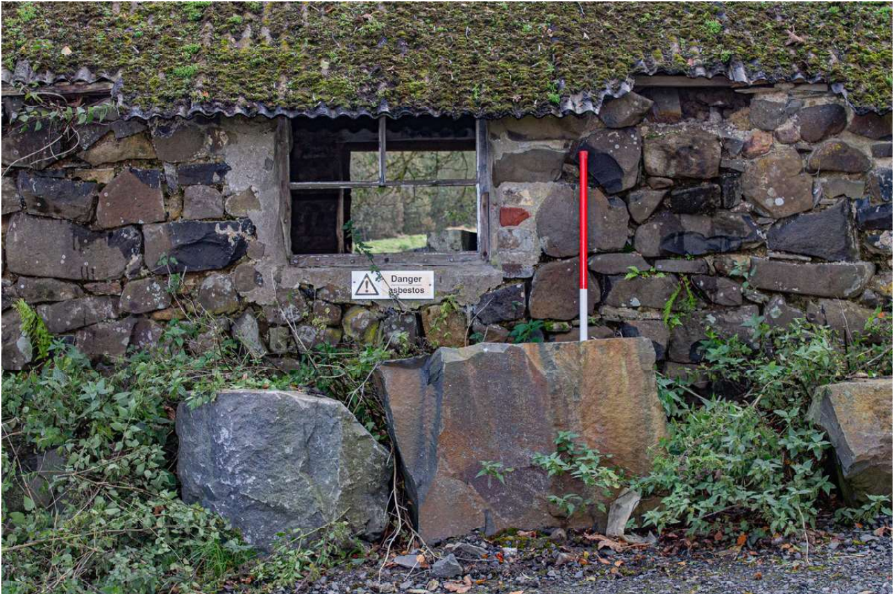
Plate 39 (41): Building B (Barn), detail of the inserted window of Barn B2 in the north-east side of the north-west elevation, from the north-east
