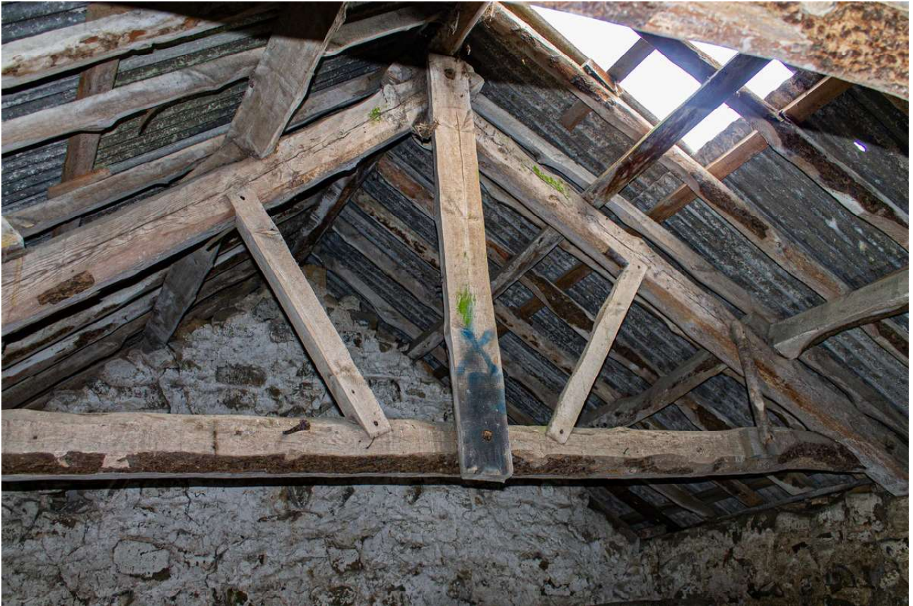
Plate 59 (59): Building B (Barn), Barn B2, general view of the north-east timber roof truss from the west
