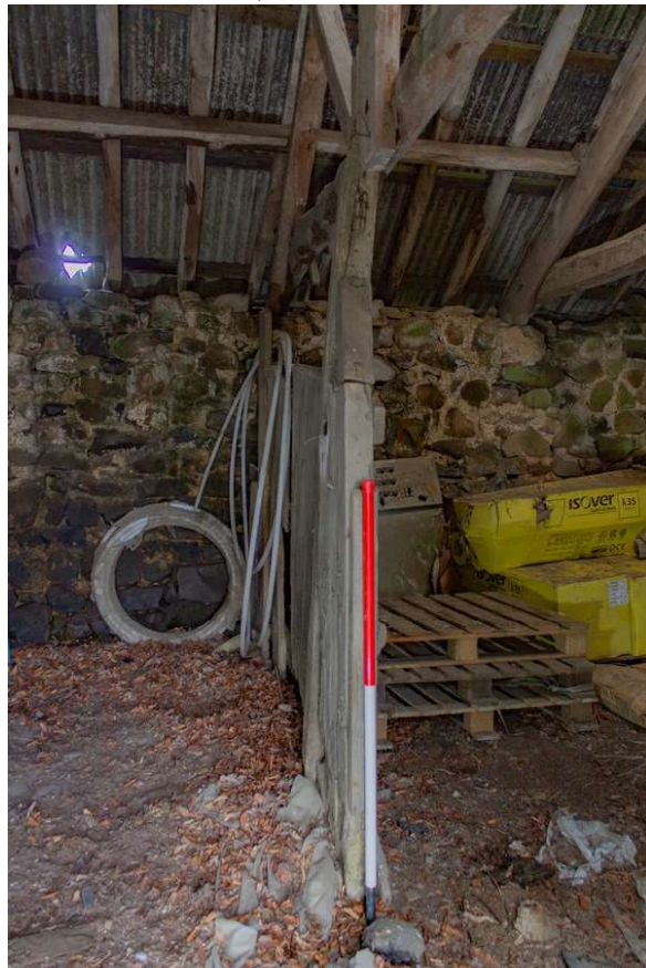
Plate 52 (52): Barn B1, Building B (Barn), detail of the timber partition for the animal pen, from the south-east
