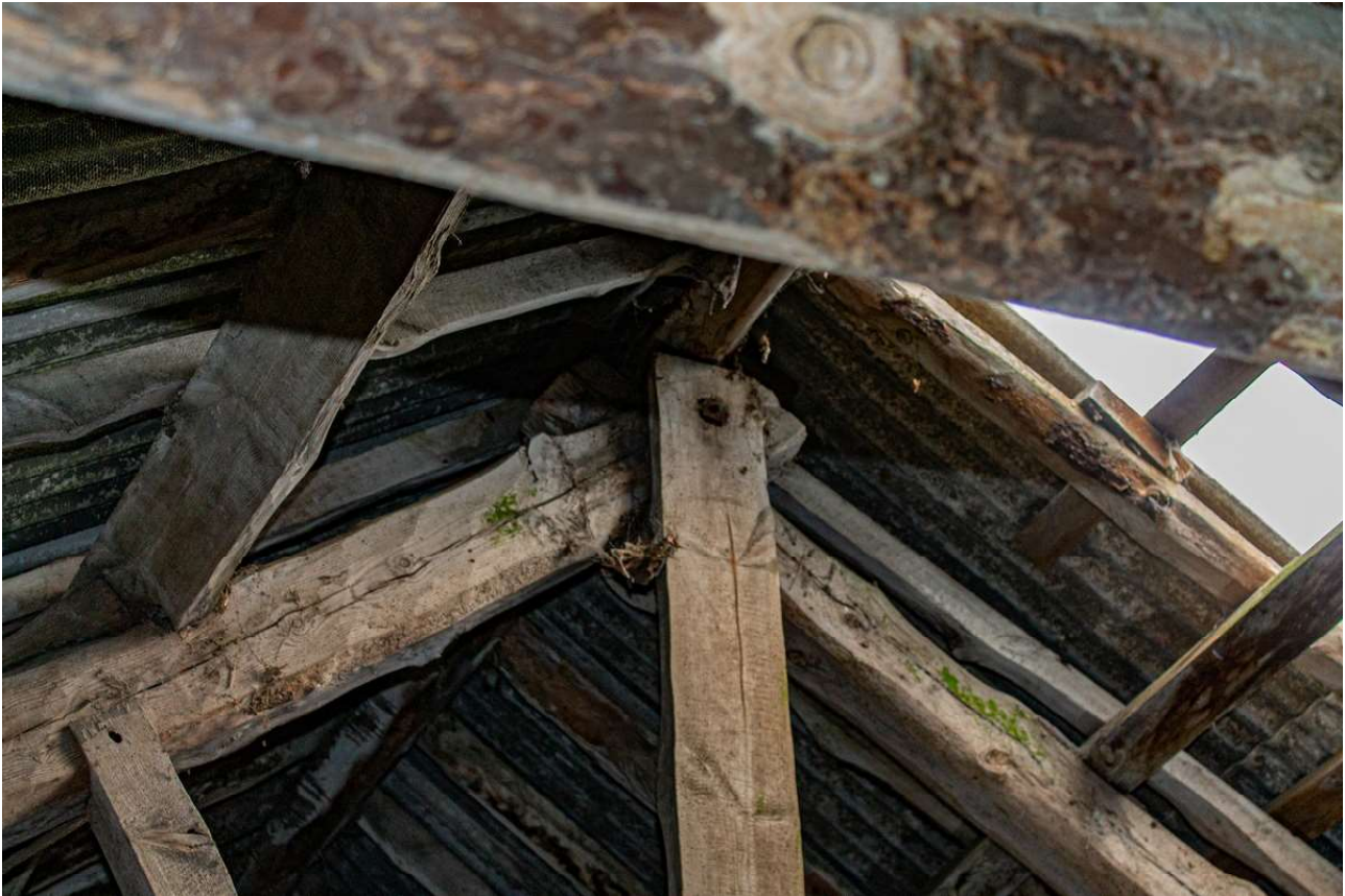
Plate 63 (62): Building B (Barn), Barn B2, detail of the top of the north-east roof truss showing the king post bolted to the rafters, from the south-west
