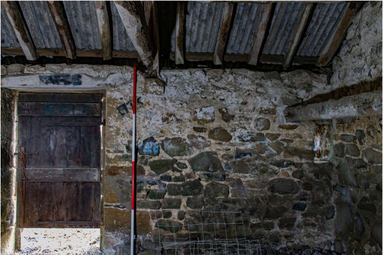
Plate 55 (58): Barn B2, Building B (Barn), general view of the south-west side of the south-east elevation showing the low timber and slit window (to the right) and the main doorway (to the left), from the north-west
