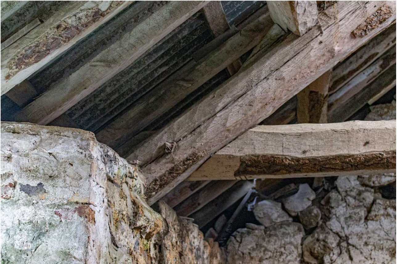
Plate 65 (63): Building B (Barn), Barn B2, detail of rafter of the north-east timber roof truss resting over the north-west wallhead, from the south-west
