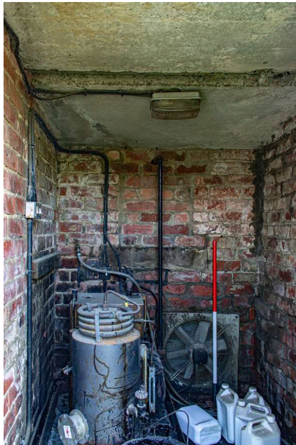
Plate 28 (28): Building A (Cottage), general view of Room A9, coal shed/log store, showing the blocked rear window, from the north-east
