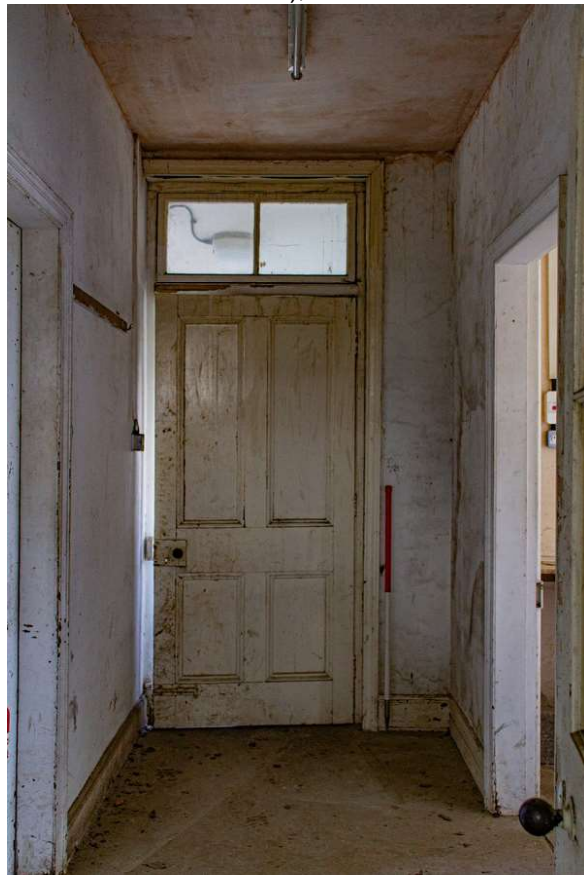
Plate 18 (17): Building A (Cottage), detail of the door in the north-east side of corridor A1b (through to the back passage, Room A8a), from the south-east
