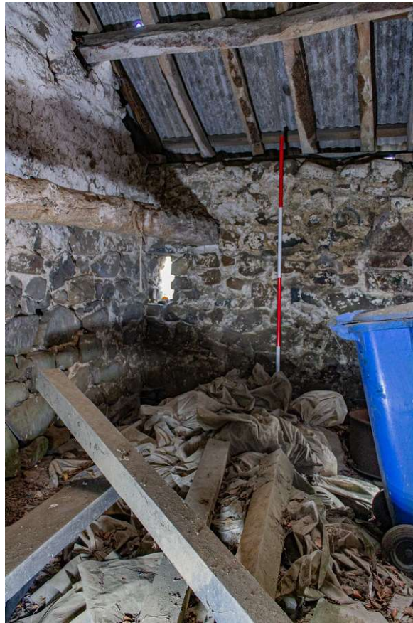
Plate 57 (57): Building B (Barn), Barn B2, detail of the north-east side of the south-east elevation showing the slit window and low timber, from the WNW
