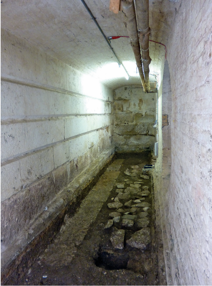
Fig 11 Glaziers Hall, basement wine cellar, looking south. In-situ stone blocks forming part of the 19th century London Bridge visible at ground level and in the south and east wall faces. (Photograph © MOLA)
