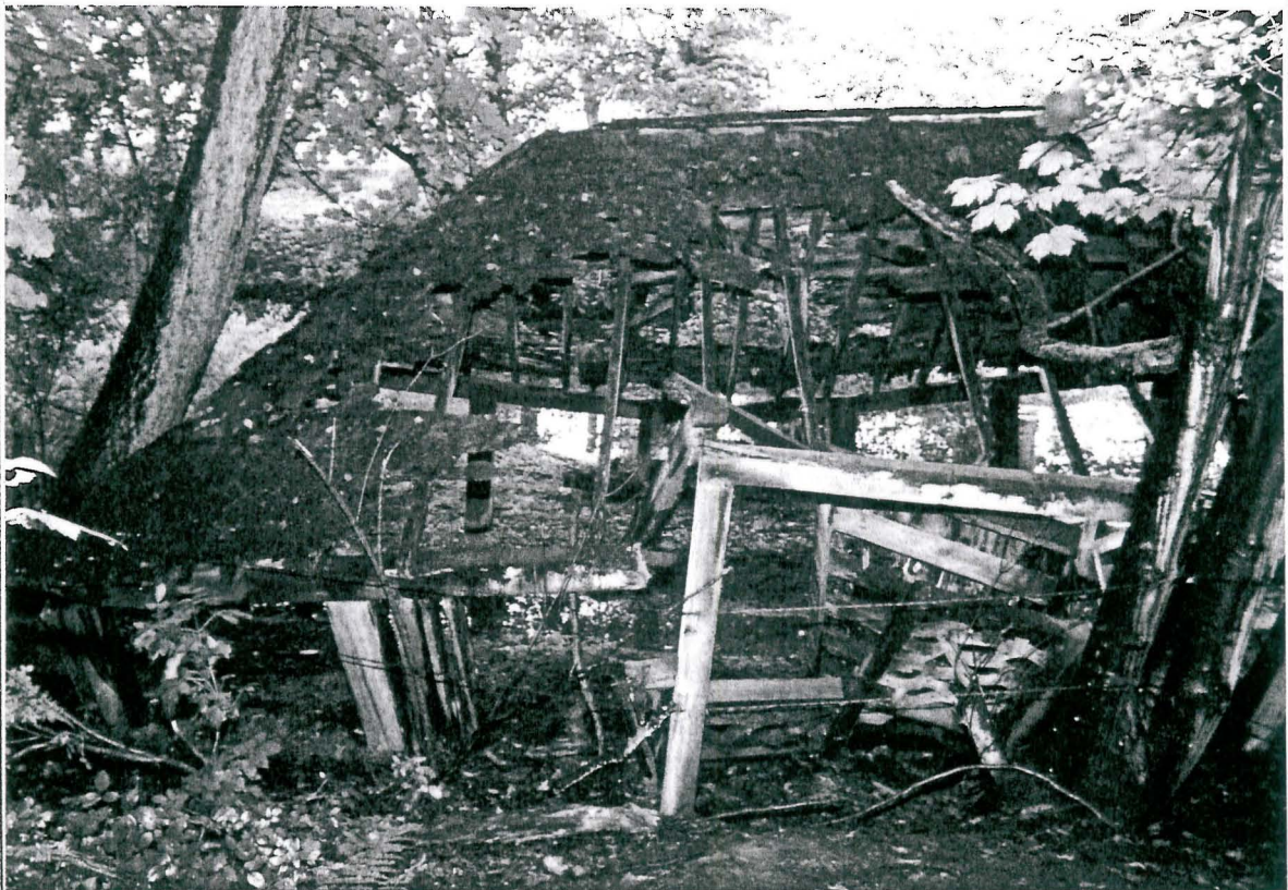
The boathouse from the south, landward side, including the collapsed porch
