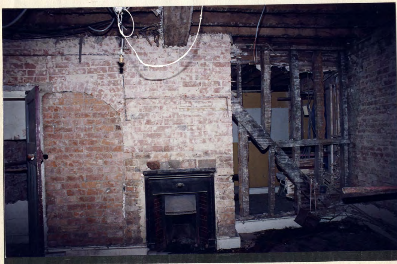
Building E: 1st floor from the north, showing the chimney stack and re-used timbers
