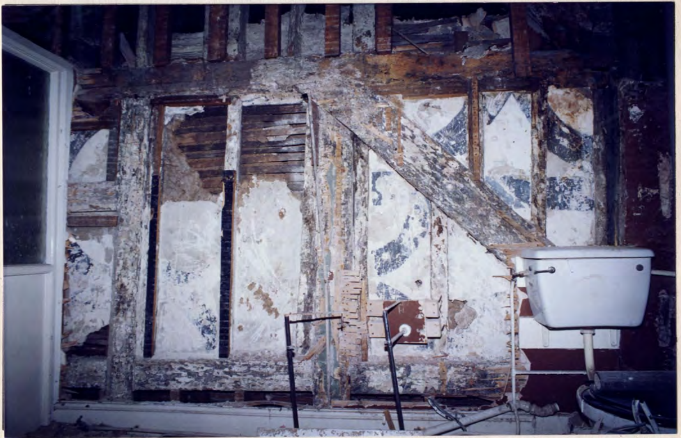
Building A: Intermediate frame, 1st floor, south face, showing wall paintings across blocked doorway
