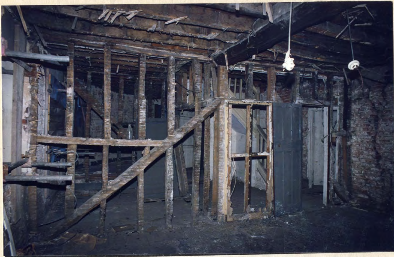
Building D: 2nd floor from the south, showing the poor quality timber dividing frames
