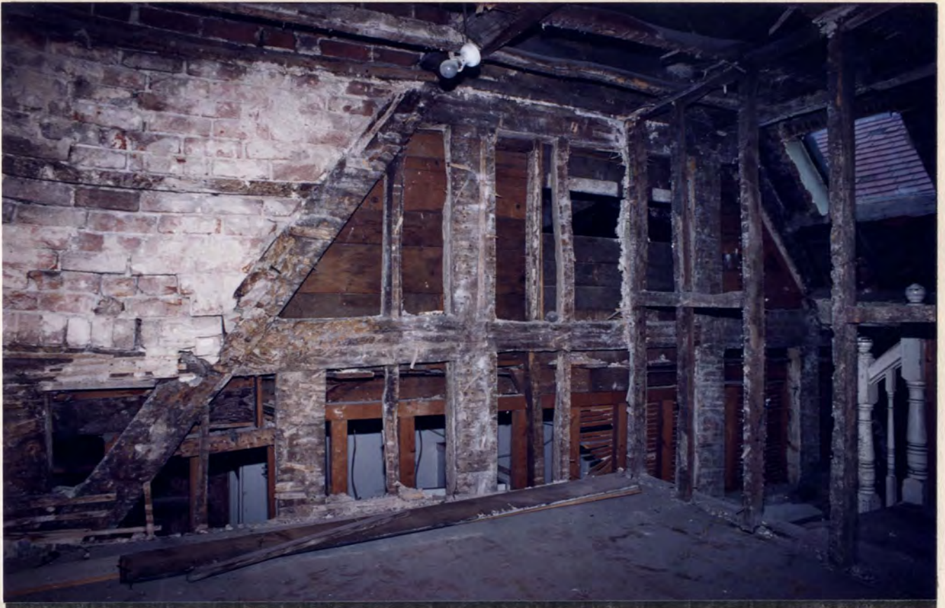
Building A: Intermediate frame, attic floor, south face, showing central opening cut through lower collar
