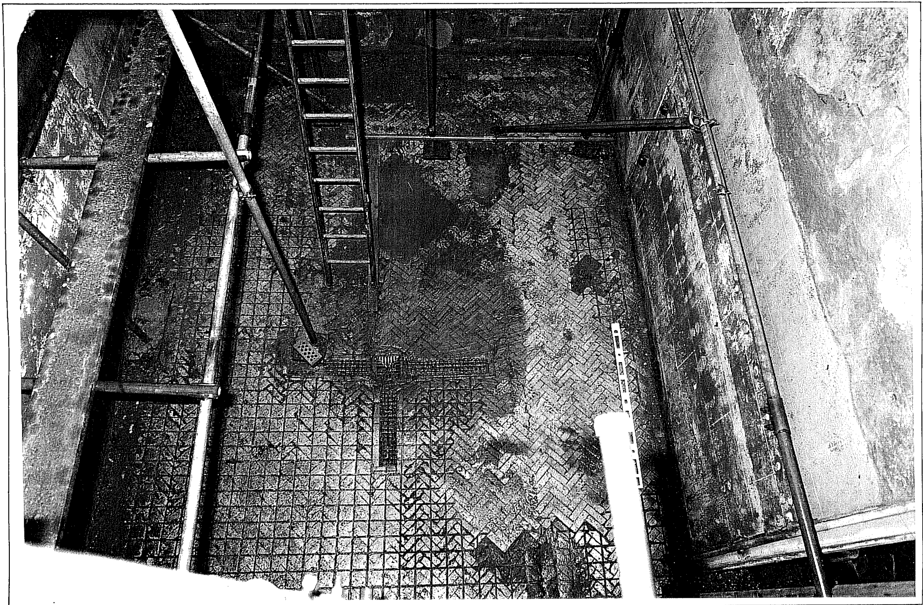
The floor showing the pattern of the clinkers, the iron drain and the concrete patching.
