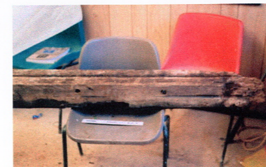
Plate 14, Moulded timber re-used as a lintel from the doorway between Rooms 1 and 2 (showing the good side).
