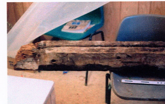
Plate 13, Moulded timber re-used as a lintel from the doorway between Rooms 1 and 2 (showing the good side).
