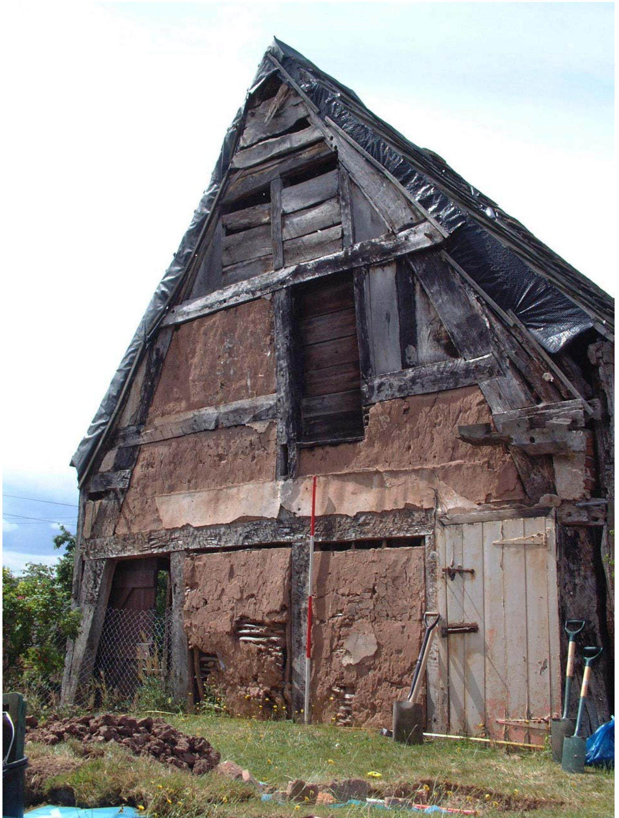
Plate 14: Cruck frame C1 looking south-west. The door is the location of the earlier door between the domestic end and the byre (Scale 2 metres)
