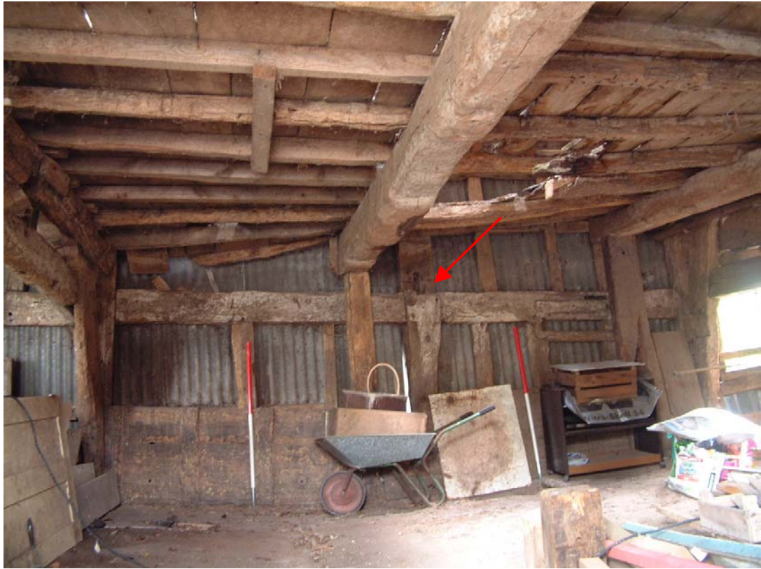
Plate 17: Southern framing of Bay 2. The bridging beam is inserted and originally was tenoned into the central post (arrowed)
