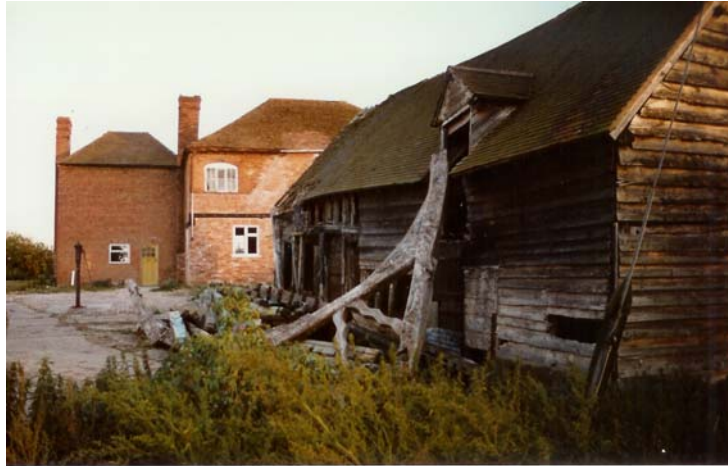
Plate 1: The cruck frame removed during the late-20 th century stands propped against the building (Photograph by courtesy of Mr and Mrs Barnes)
