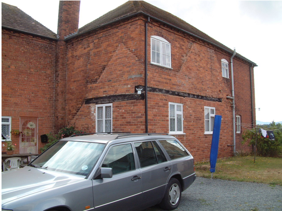
Plate 20: Remaining timber-framing in the external walls of the present farmhouse; also note the shadow lines of the former rooflines.
