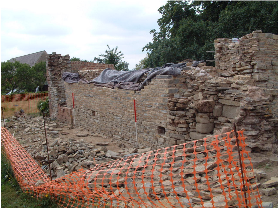
Plate 5: Putlog holes in the lower face of the eastern elevation, scales 1-metre.
