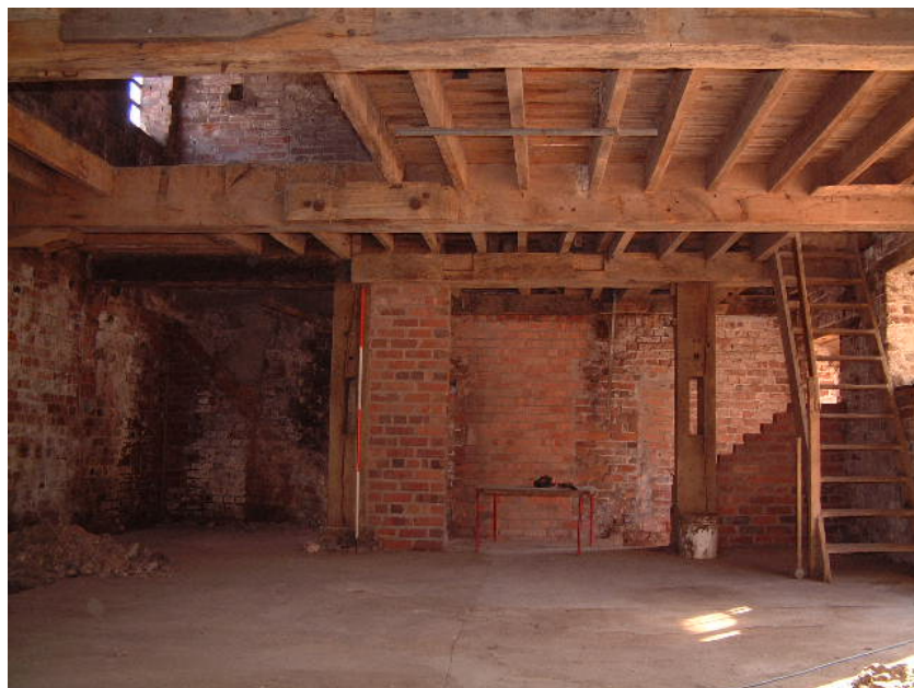
Timbers of the former 'hurst-frame' at the eastern end of the ground floor (scale 2 metres)
