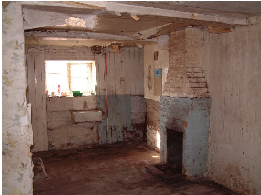
Room lately used as part of cottage in western end bay at ground floor. Possibly, this was an earlier overseers office (scale 2 metres)
