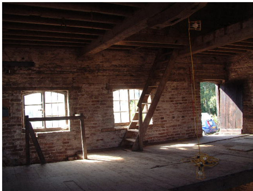
First floor showing steps up and down and loading door (scale 2 metres)
