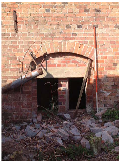
Former door into link building (now gone), which was between the mill and the building lately used as a stable (scale 2 metres)
