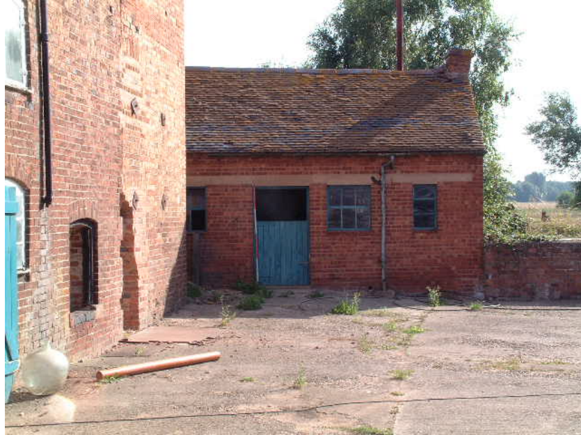
The stable block at the eastern end of the mill (scale 2 metres)
