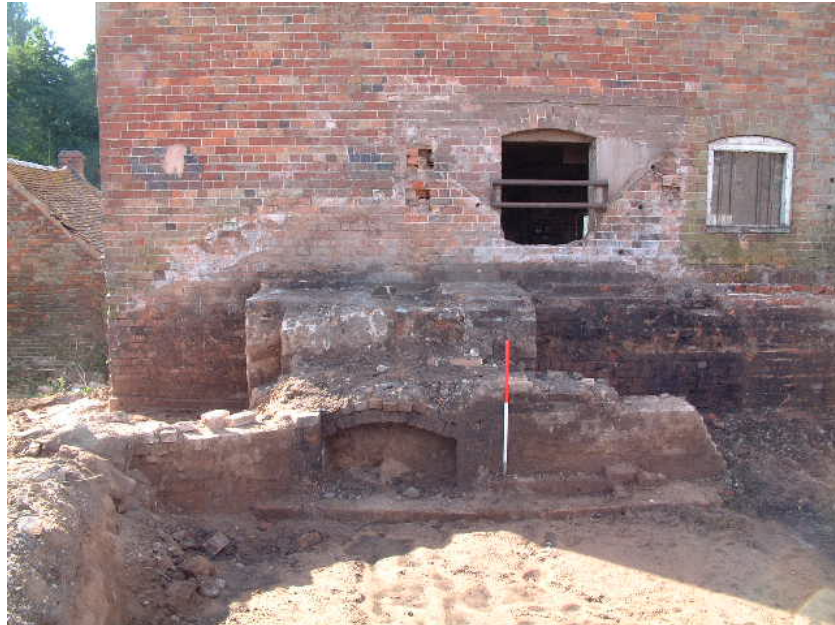
The inlet (penstock) to the rear of the wheel chamber (scale 1 metre)
