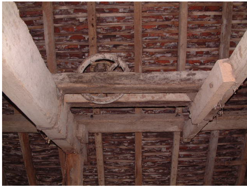
The sack hoist wheel
