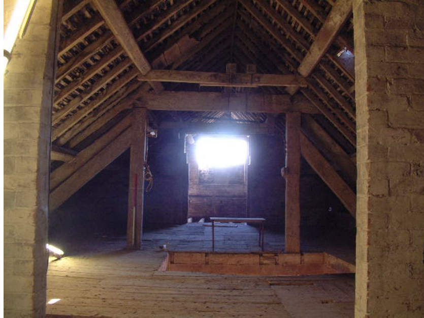
The central truss in the attic floor of the mill (scale 1 metre)
