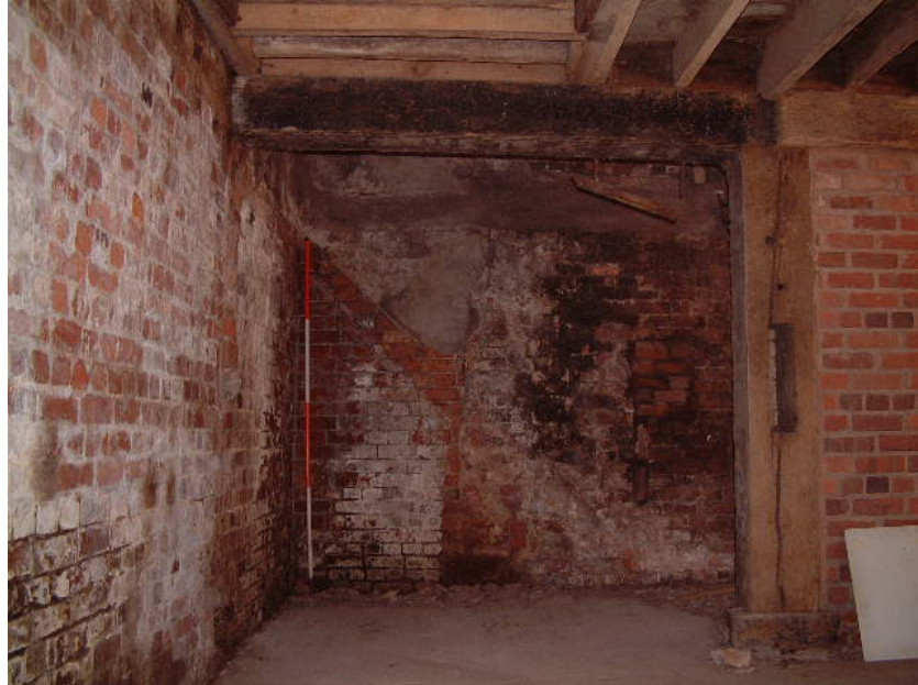
Alterations in the eastern bay for modern grain processing infrastructure (scale 2 metres)
