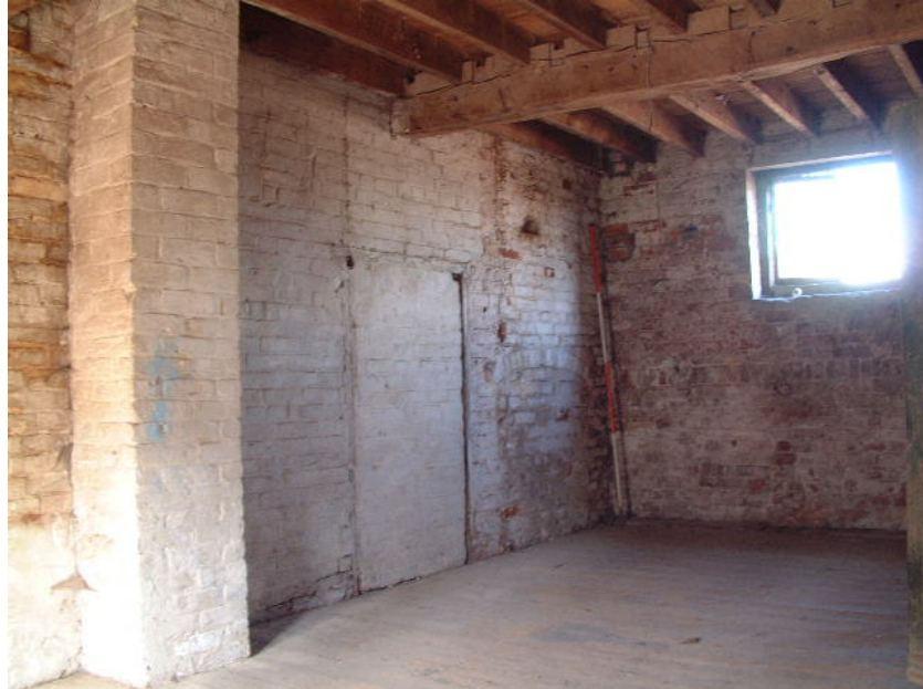
Blocked former window to farmhouse and blocked doorway between farmhouse and mill (scale 2 metres)
