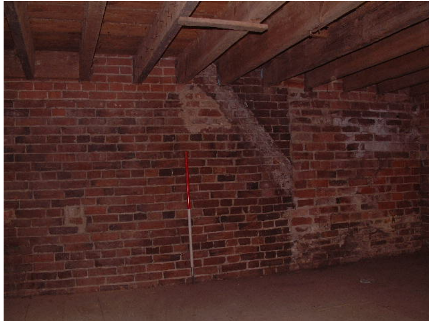
Butt joint of the mill extension to the north and former roofline at 2 nd floor level (scale 1 metre)
