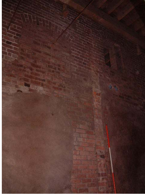
Blocked apertures at first floor level above wheel chamber. Wall scar is a modern feature (scale 2 metres)
