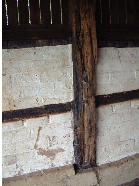
Another re-used timber has a groove to take the bottom end of wattle staves for wattle and daub panelling. The timber would originally have been horizontal (Building 2)
