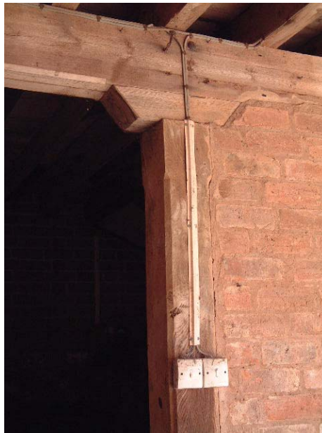
The high quality of carpentry in Building 4B is indicated in the chamfered and stopped post and beam. The wall is a later insertion
