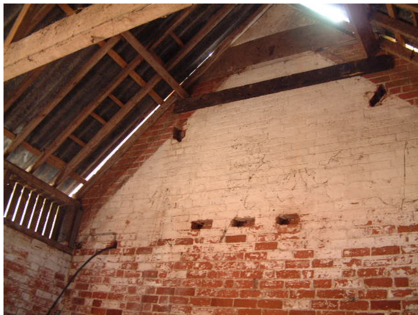
The former roofline of Building 4A is preserved on the gable end of Space 4B, note also the holes in the wall to receive the roof purlins.
