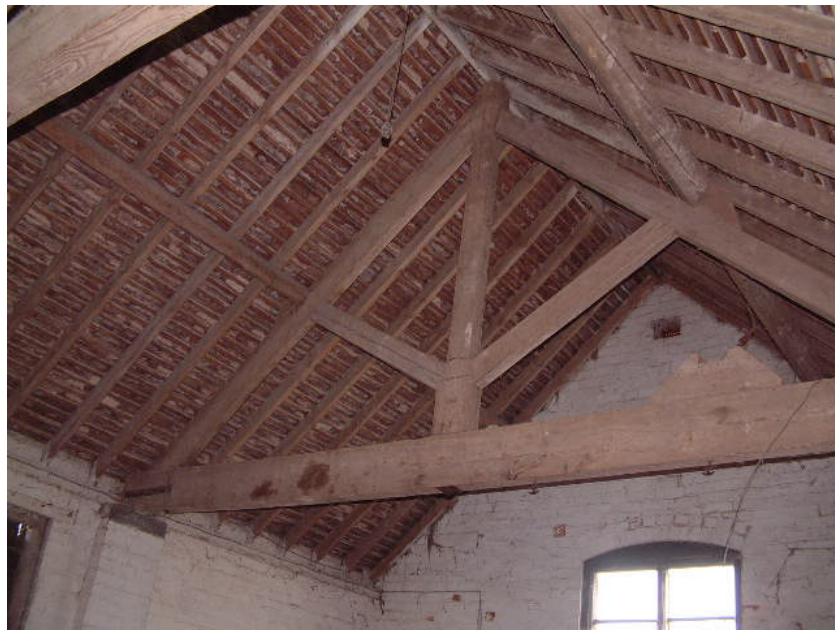
Kingpost roof-trusses in the granary (Building 4B), note the bracket on the tiebeam, which would have acted as a pivot point to haul sacks up and down from the cartshed below
