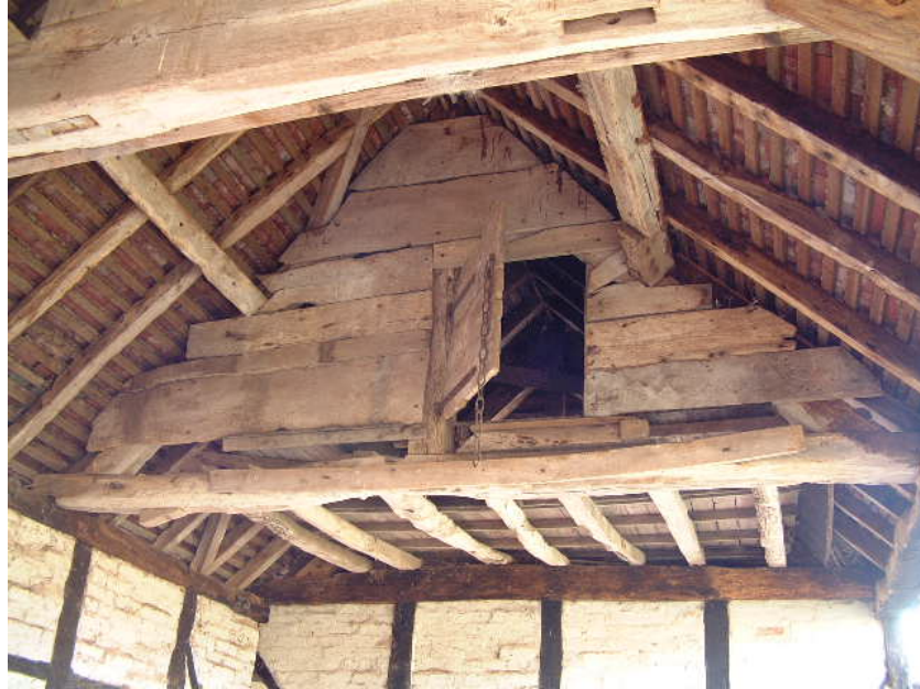
Pigeon loft in the rafters of Building 1, looking south
