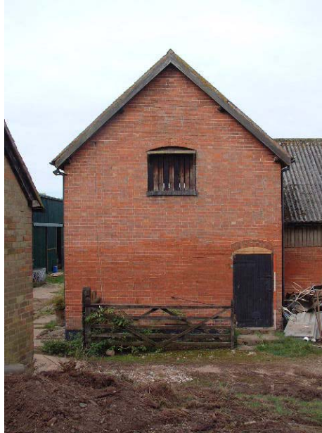
Pitchin- eye and door to the stairs in the eastern gable end of Building 4B (scale 2 metres)
