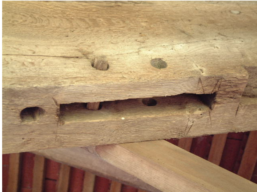
Carpenters scribe marks show that he had made a mistake when marking out for this mortise (Building 2)
