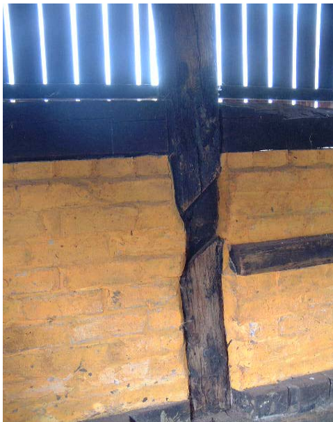
Half-lap joint indicating that this timber in Building 2 is re-used from an earlier timber-framed building, probably to take a sill beam to post tension brace.
