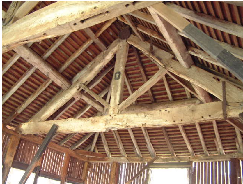
Re-used timbers with empty mortises, stave holes and peg holes in Building 2 truss
