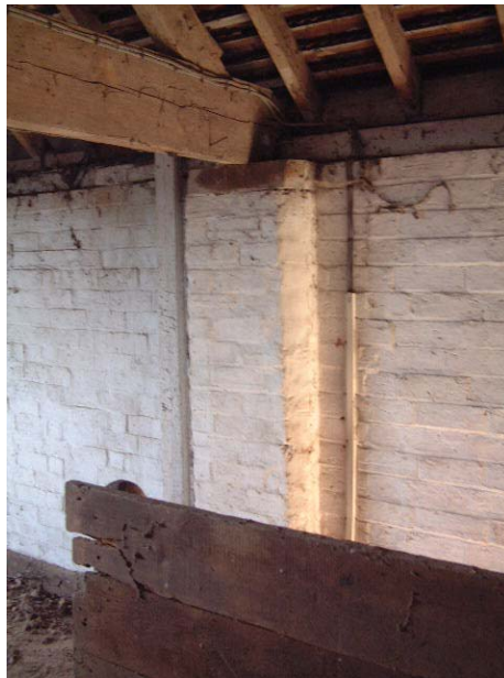
The rounded bricks on the truss support pier at the top of the stairs into the granary. All the other piers have straight edges
