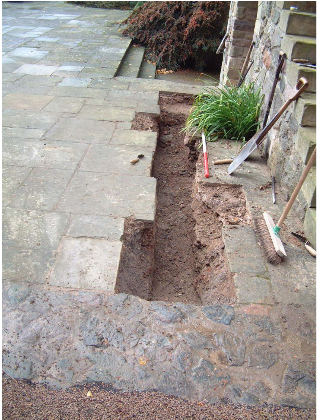
The excavated ducting trench to the south of the former nave wall, now demarcated by modern stone at the edge of the external courtyard. The material below the flags is a make-up layer associated with the levelling of the courtyard in the 1960's (scale 1 metre)
