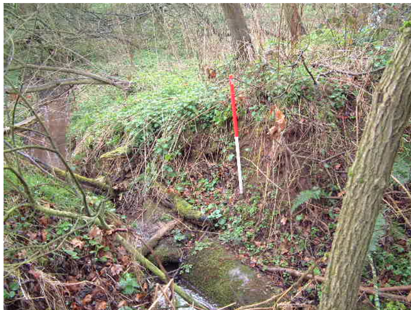
Clay abutment of former footbridge south of the present stream crossing (Looking west; Scale 1 metre)
