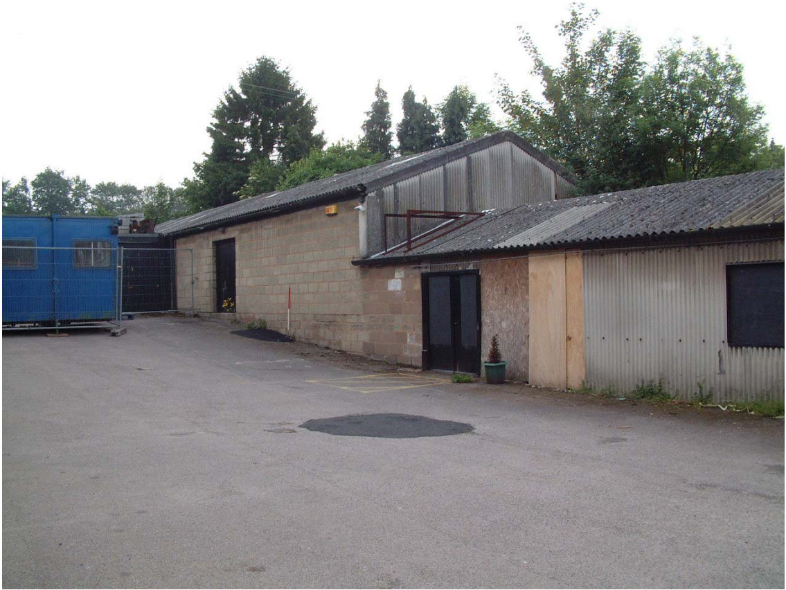
PLATE 3: Modern buildings to the rear of the store looking south-east (scale 1-metre)
