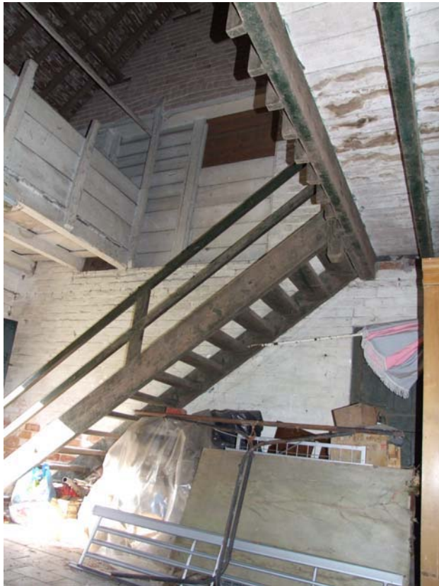
Plate 5: Stairs, landing (right) and bridge (left) in the cart bay of the northern range
