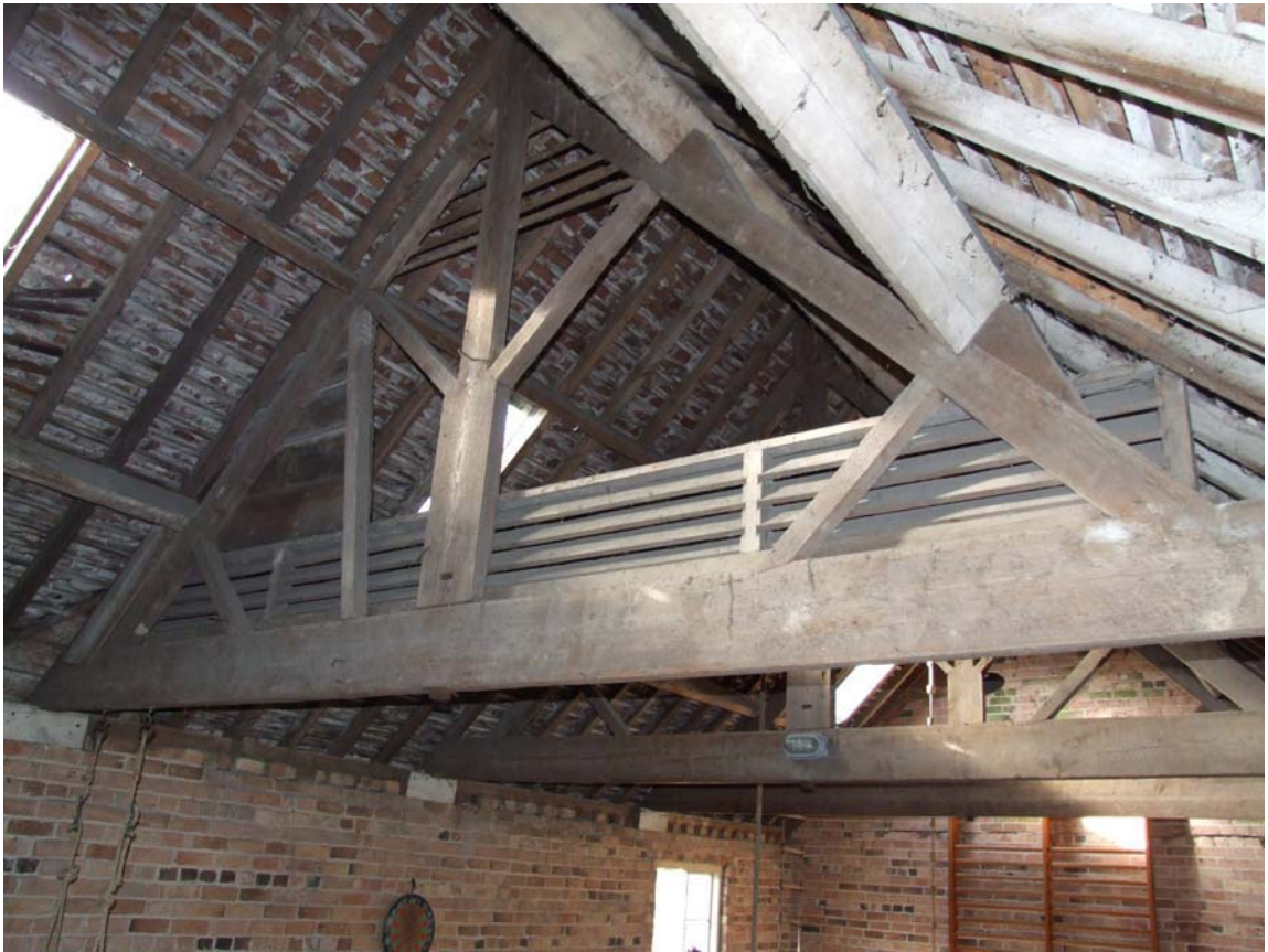
Plate 7: Truss in the northern range, typical of those used elsewhere at the site
