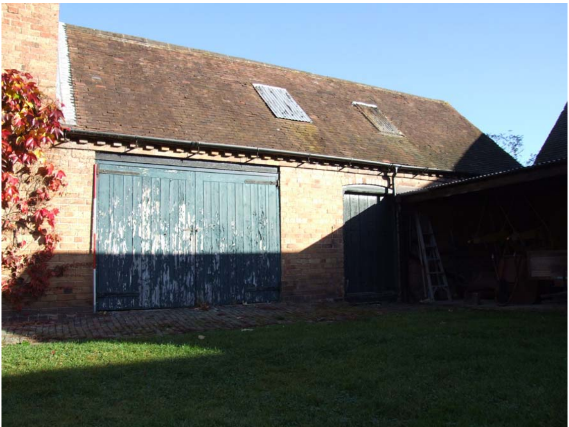
Plate 8: Possible inserted double doors in single storey element of the northern range
