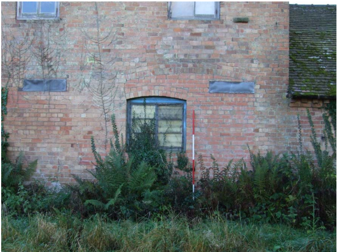
Plate 6: Blocked doorway with later inserted window in the north elevation of the northern range
