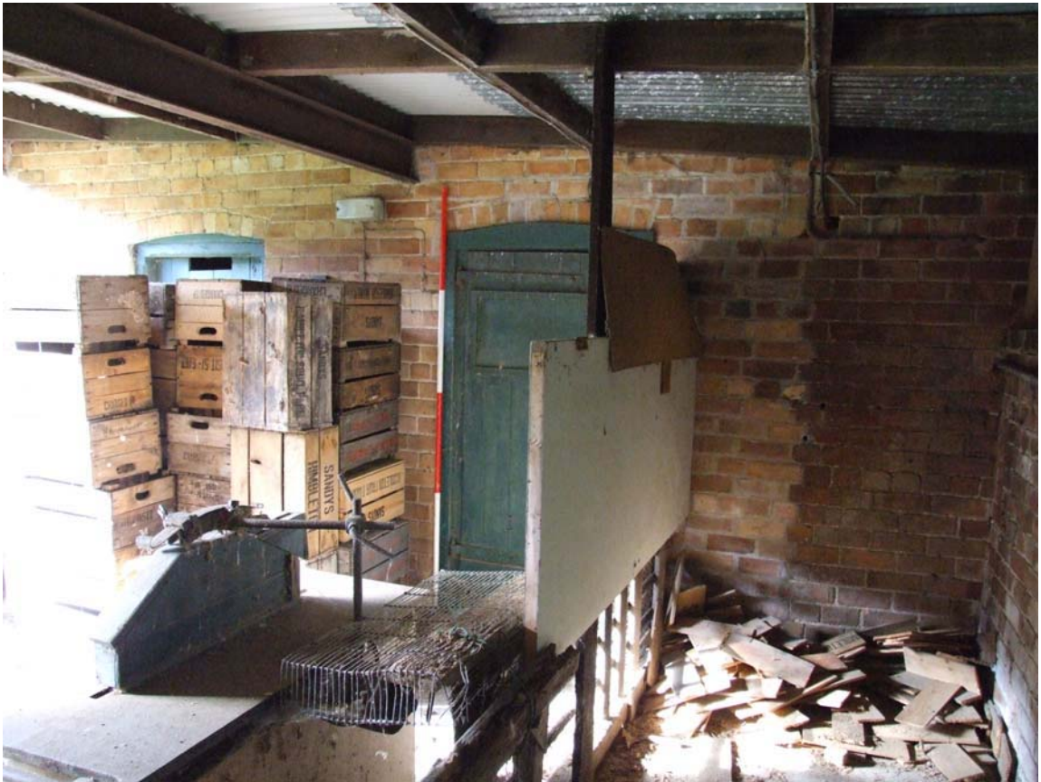
Plate 21: Stable block in the north-west corner of the complex, with later wall (right)
