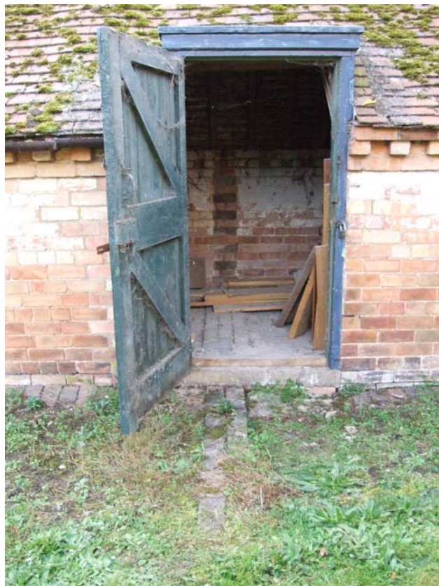
Plate 20: Scar of former wall of pigsty, indicating door is a later insertion
