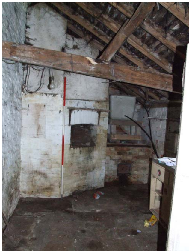
Plate 20: Bread oven and boiler at the western end of the lean-to (scale 2-metres)
