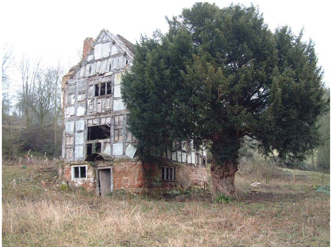
The Old Court and ancient Yew, which is probably contemporary with the build, looking north-east
