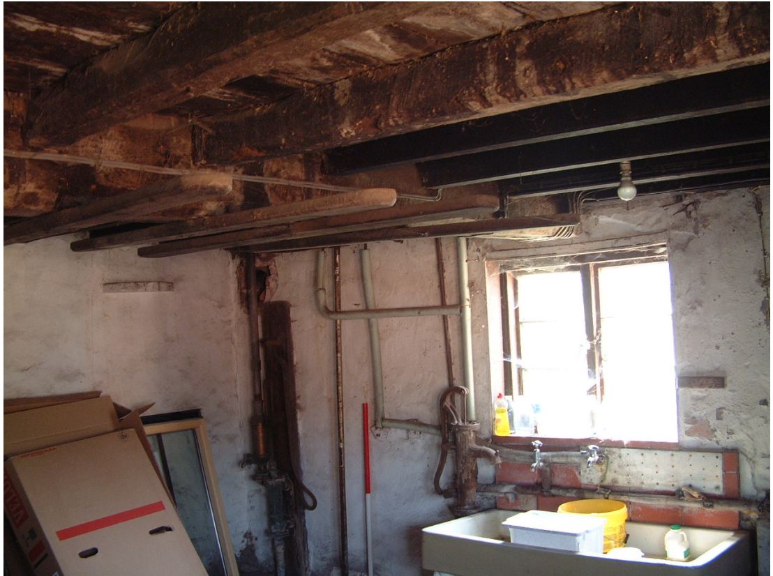
Pump and sink in wash room in the northern cross-wing
