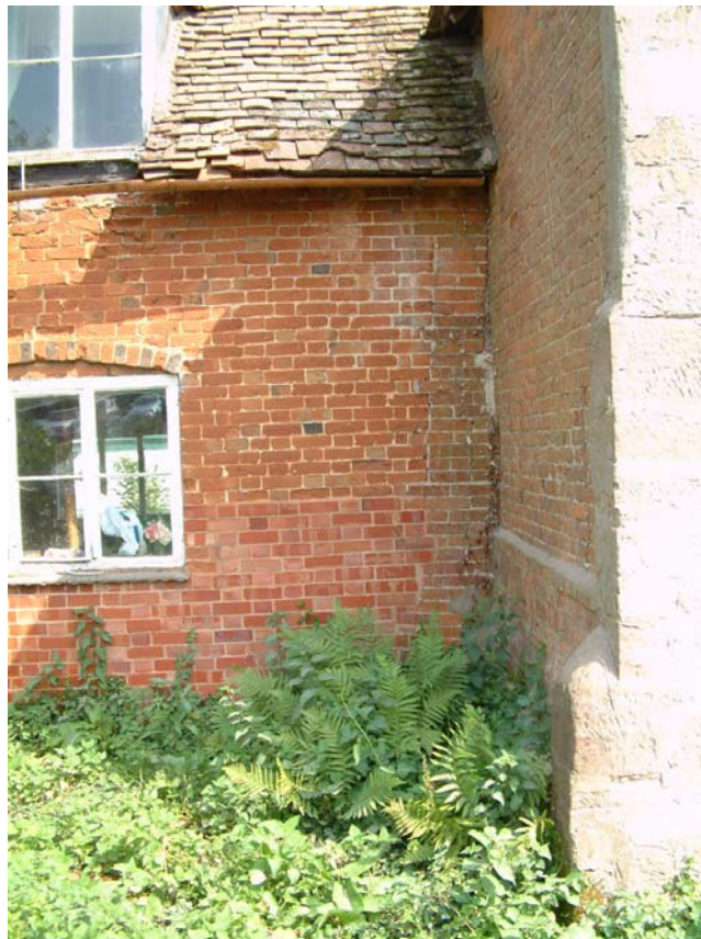
Infill brickwork at corner of hall and the southern cross-wing, looking east
