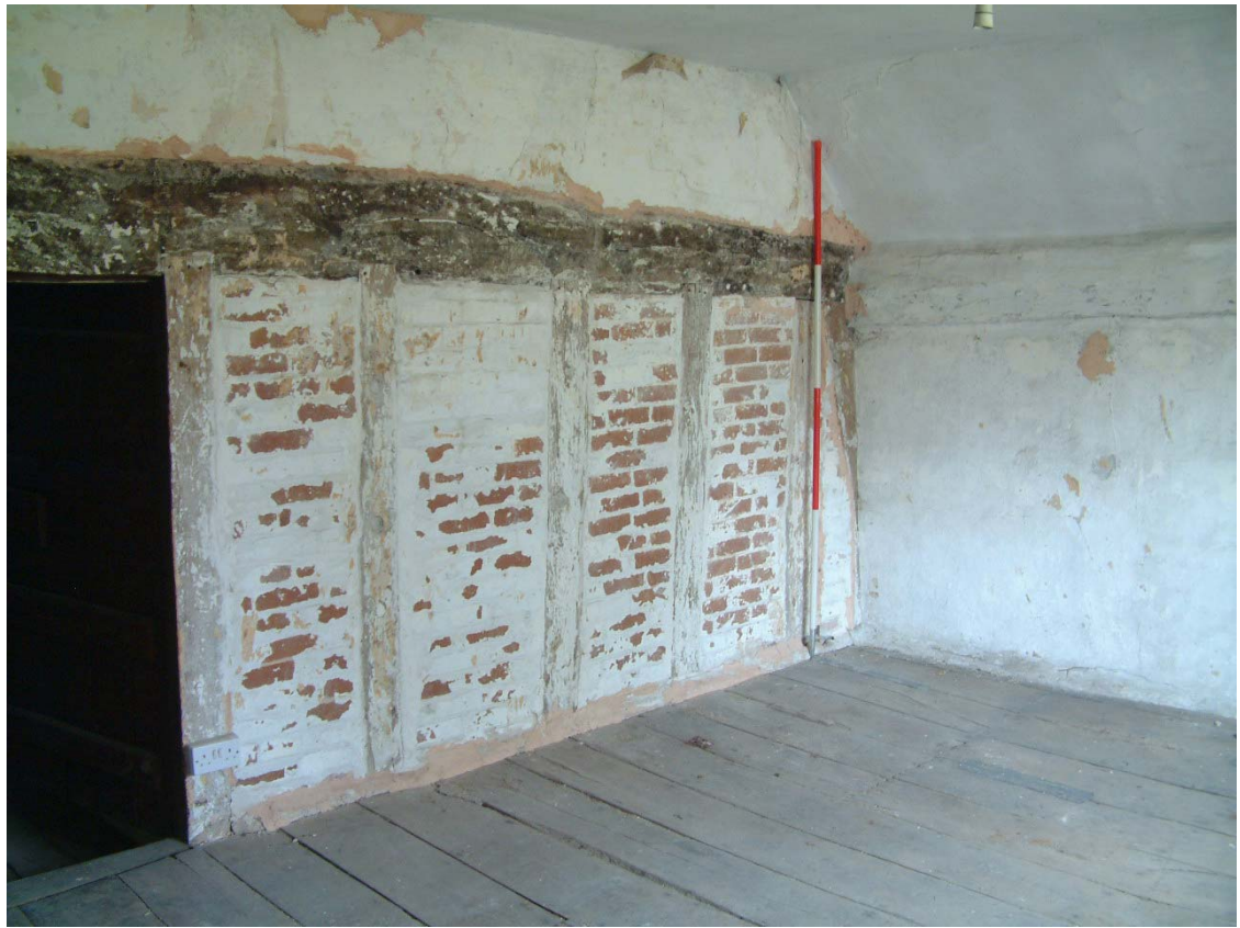
Plate 7: Inserted central partition below the tiebeam of the upper floor of northern cross-wing (Scale 2 metres)
