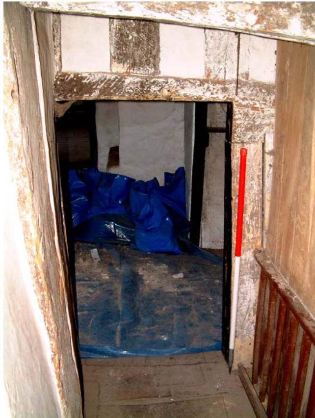
Plate 10: Doorway cut through the tiebeam of the northern framing of the hall (Scale 1 metre)
