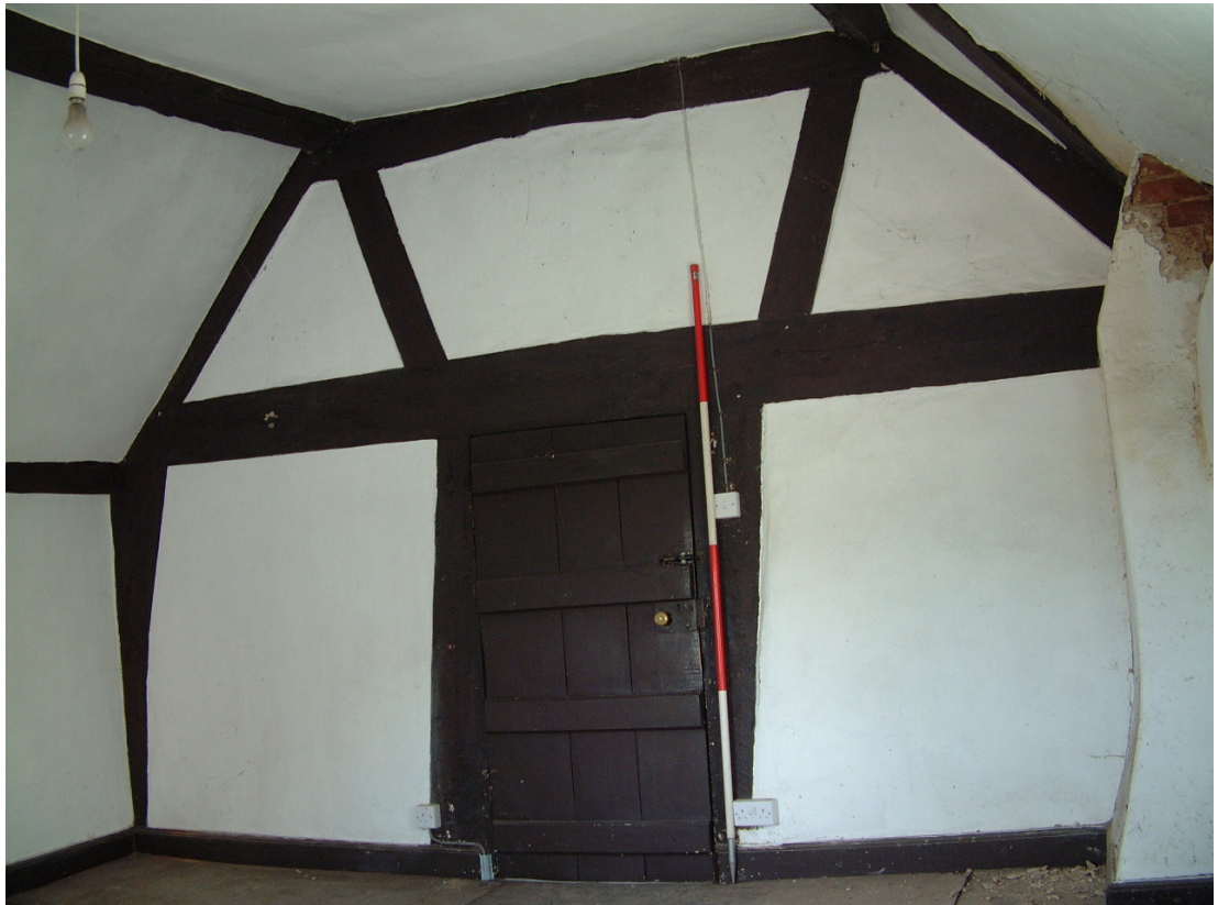
Central truss of southern cross-wing in the western solar room (Scale 2 metres)
