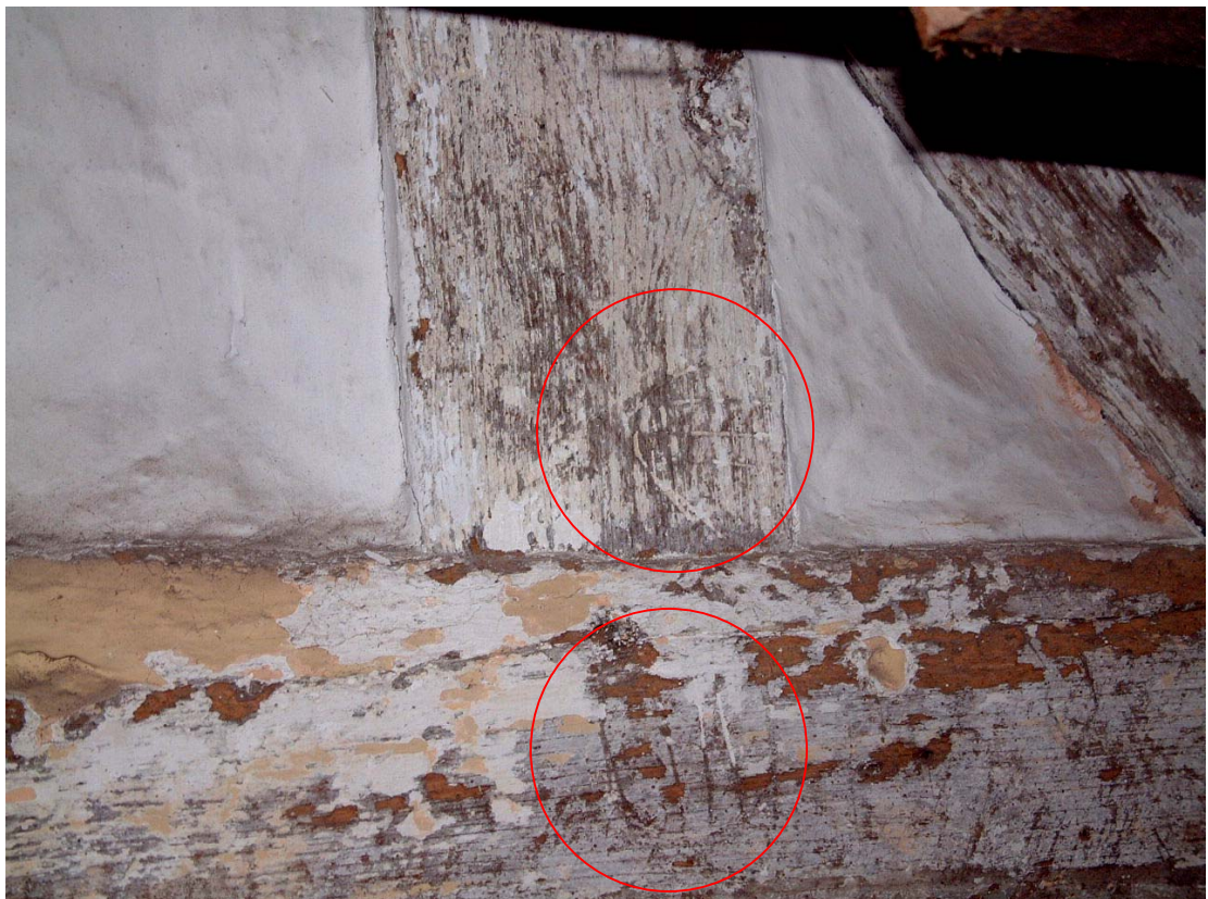
Plate 8: Carpenters assembly marks on the studding and tie-beam of the northern hall frame (northern face)
