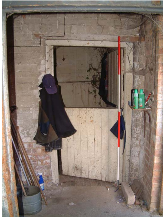
Plate 11: Stable door between the north and south room of the single storey building (scale 2-metres)
