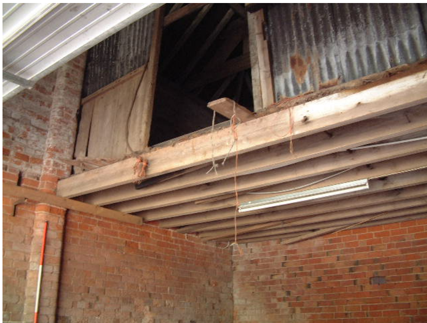
Upper floor (former granary) in Building 1 has been partially removed, note the gap for a joist (left) and sawn off floorboards (sections on scale 0.50 metres)
