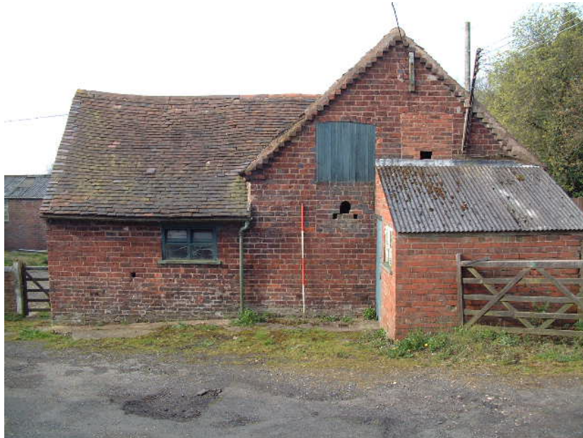
Later addition built against the eastern elevation of Building 1. Note the blocked doorway and window to the obsolete granary and the holes for shafts for portable steam engines (scale 2 metres)
