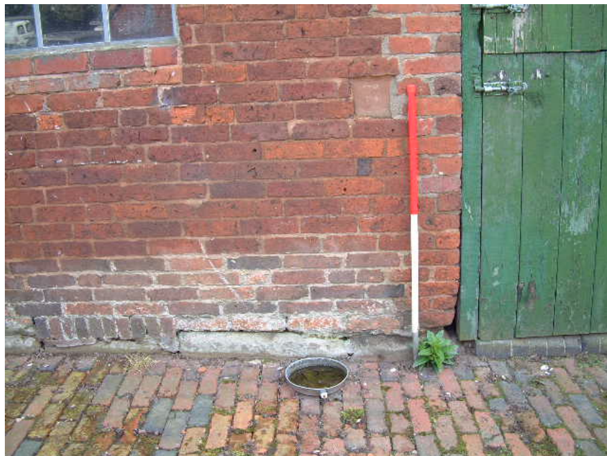
Smaller bricks used at the lower level of Building 3, indicating a possible earlier phase (scale 1 metre)
