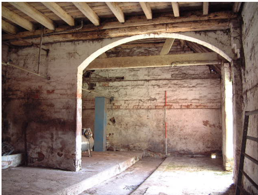
Former cart- door in the eastern elevation of Building 2. The doorway is now obscured by a later phase of building (scale 2 metres)
