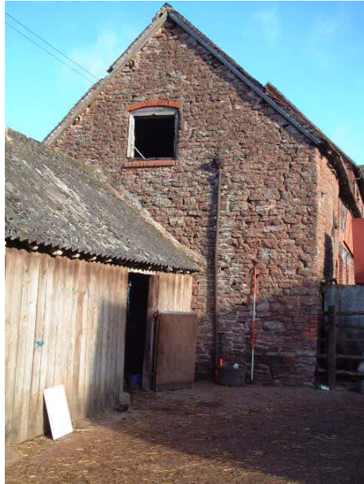
The stone stable block with hayloft above, added to the western end of the range (scale 2 metres)
