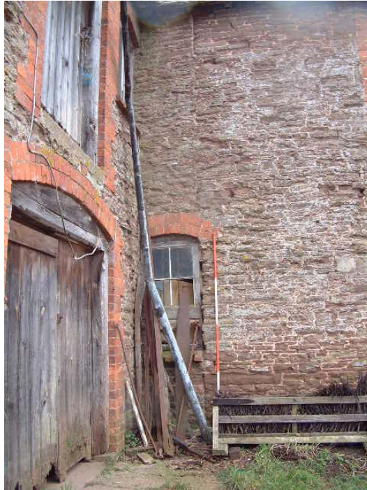
The butt joint between the former farmhouse (right) and Structure A (left) with the return range running to the west (scale 2 metres)
