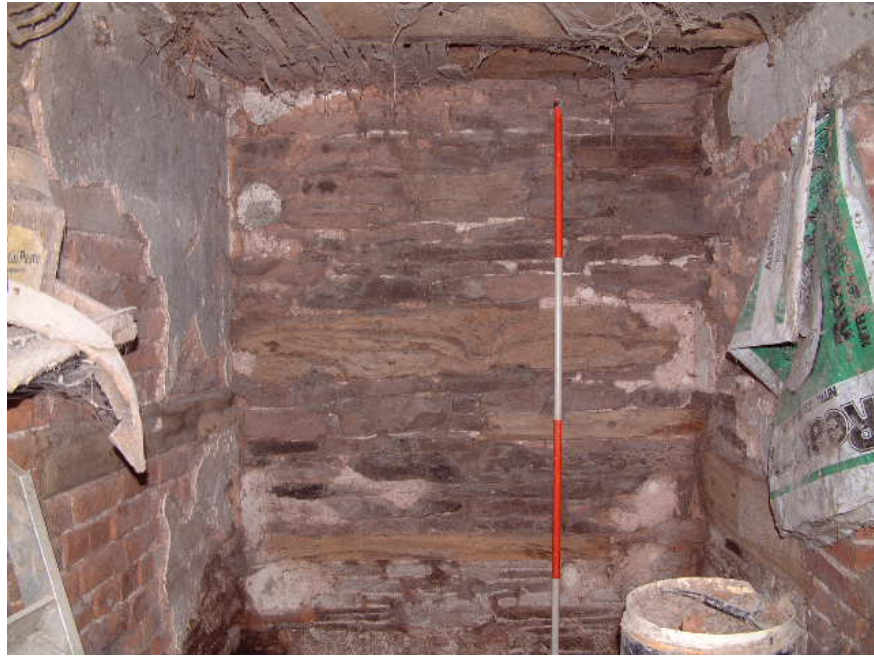
Re-used timbers in the stone wall fabric of the former farmhouse (scale 2 metres)
