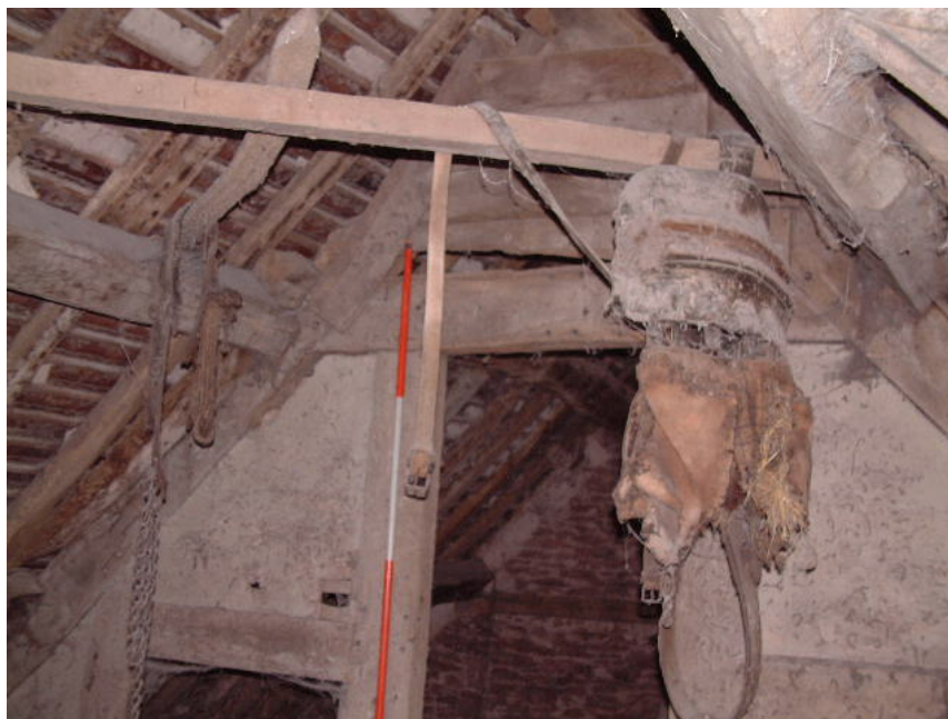
Truss in attic of former farmhouse with central access through, looking north (scale 2 metres)
