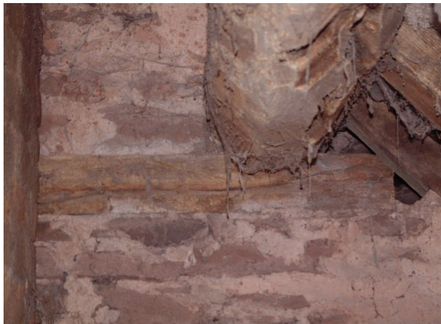
Attic purlin with cut mortises showing the timber is re-used. Also note a re-used rail in the end gable (north) with groove to take the bottoms of staves of a wattle and daub panel
