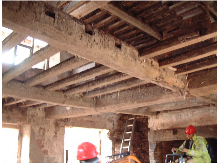
The construction of the first floor in the former farmhouse seen during the watching brief
