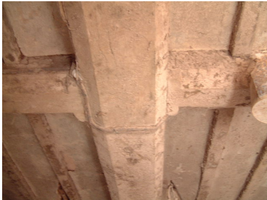
Chamfered axial and bridging beams at first floor level in the former farmhouse
