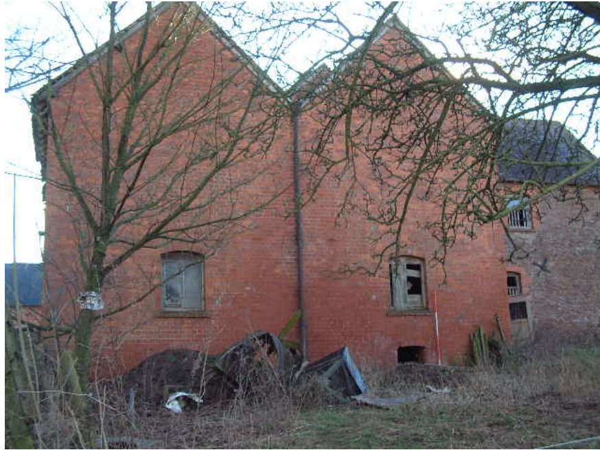
The hop kilns on the northern side of the complex (scale 2 metres)
