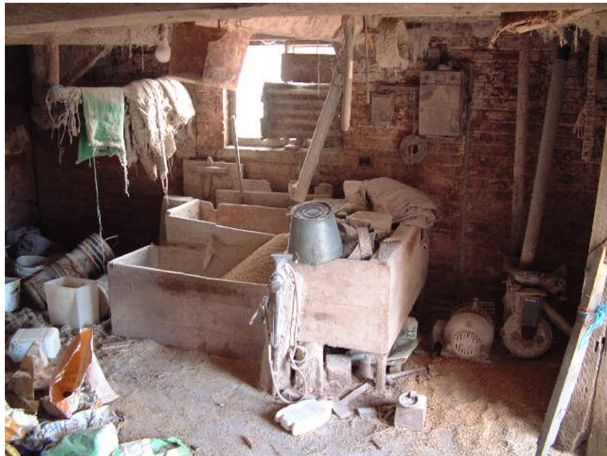
The lower floor of the former farmhouse has lately been used for milling grain
