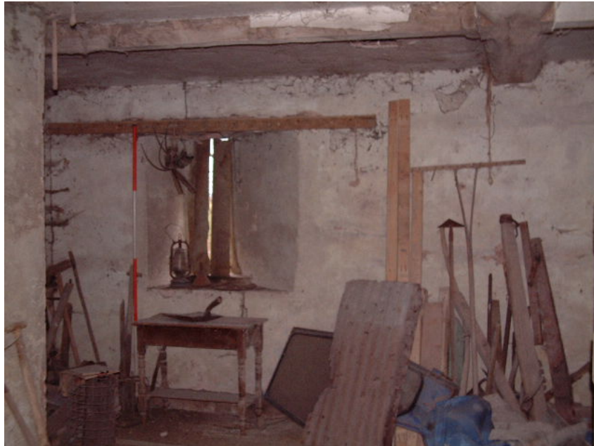
Original splayed window to the upper eastern elevation of the former farmhouse. Note the greater splayed reveal (right) into the room (scale 2 metres)
