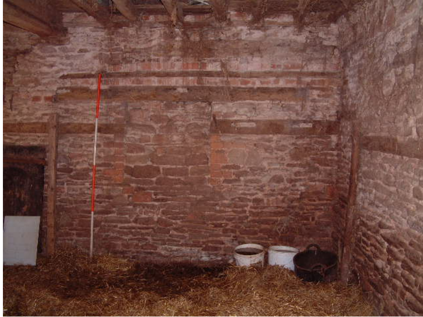
Space B (stables) looking north. Note extensive re-use of carpented timbers in the walls
