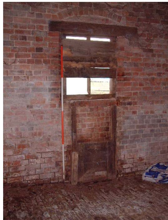
The vent in the northern elevation of one of the hop kilns (scale 2 metres)
