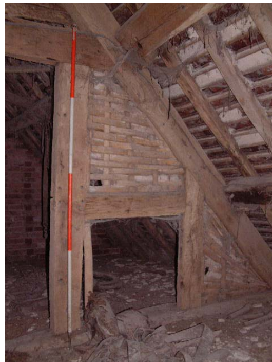
Wattle and daub panelling surviving in the truss (scale 2 metres)
