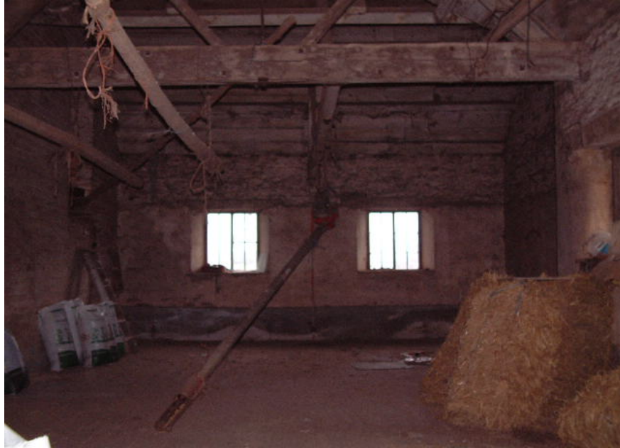
The oasthouse looking east, note the entrance to a kiln drying floor in the wall (top right by step ladder)
