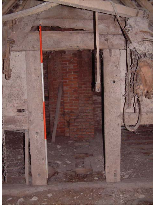
Central access through attic truss in former farmhouse looking north (scale 2 metres)
