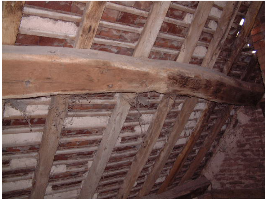
Peg-holes in an attic purlin, showing the rafters are not original to the purlin
