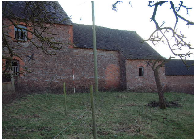
Northern elevation of space A (with windows), space B (with bricked up door) and attached stable at western end. Note the drop in roofline, although the wall is of a single build up to the end section.
