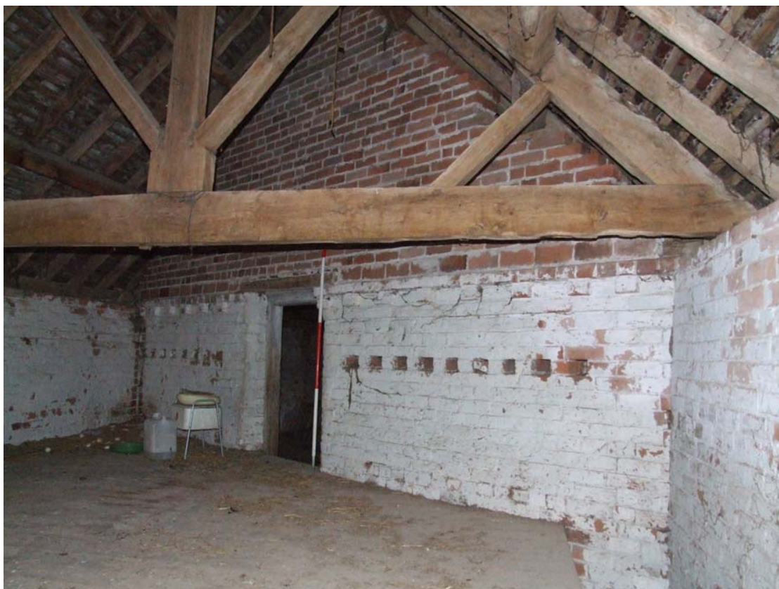
Plate 16: Dentil cornice and pierced vents carried through inside phase 2. View from upper C, looking south-west
