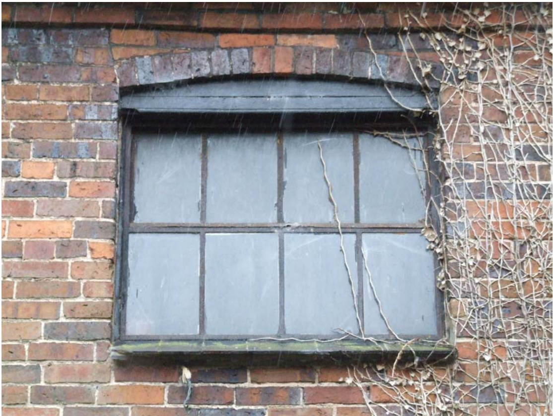
Plate 21a: 8-light iron window unit of upper floor at west end, south elevation
