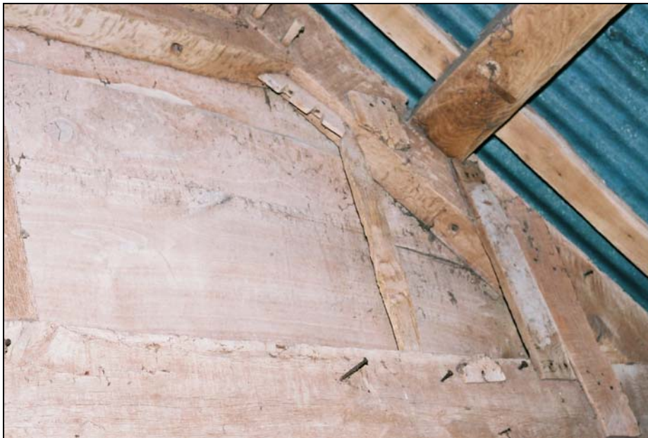
A stave can be seen in-situ between the principal and the tie-beam on Truss T2. Note the empty stave holes to either side
