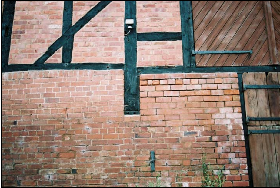
Post of the cart bay standing on the remains of the original sill beam, highlighting the extent of under-building on this side
