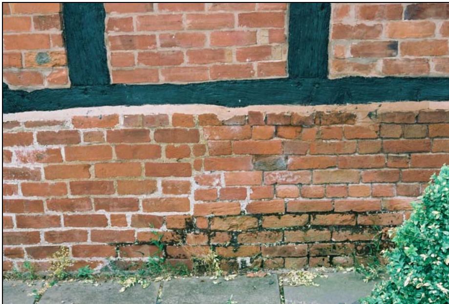
South elevation. The original brick plinth (right) and larger bricks of the plinth rebuild (left). The post of Truss T2 is the one on the right.
