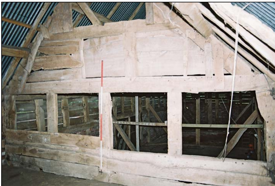
Truss T2 from the hayloft looking through along the barn to the east.
