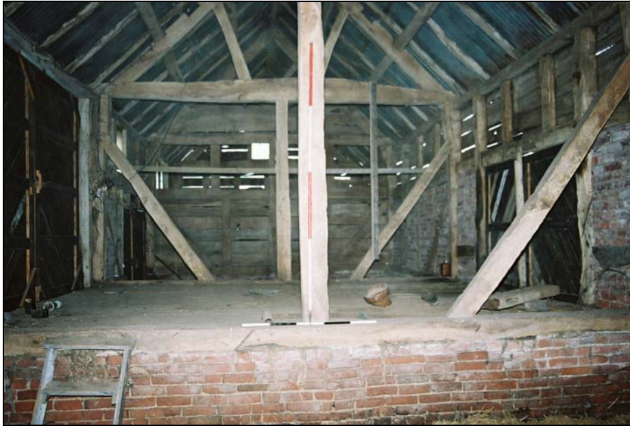
Bay3, originally the threshing bay, but now raised up and a room inserted below on the ground floor (see Plate 10)
