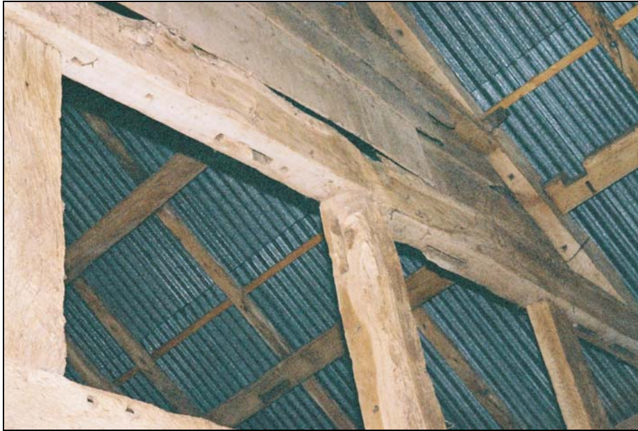
Un-used mortises and stave holes in Truss T2 suggesting this was probably originally the external western end truss
