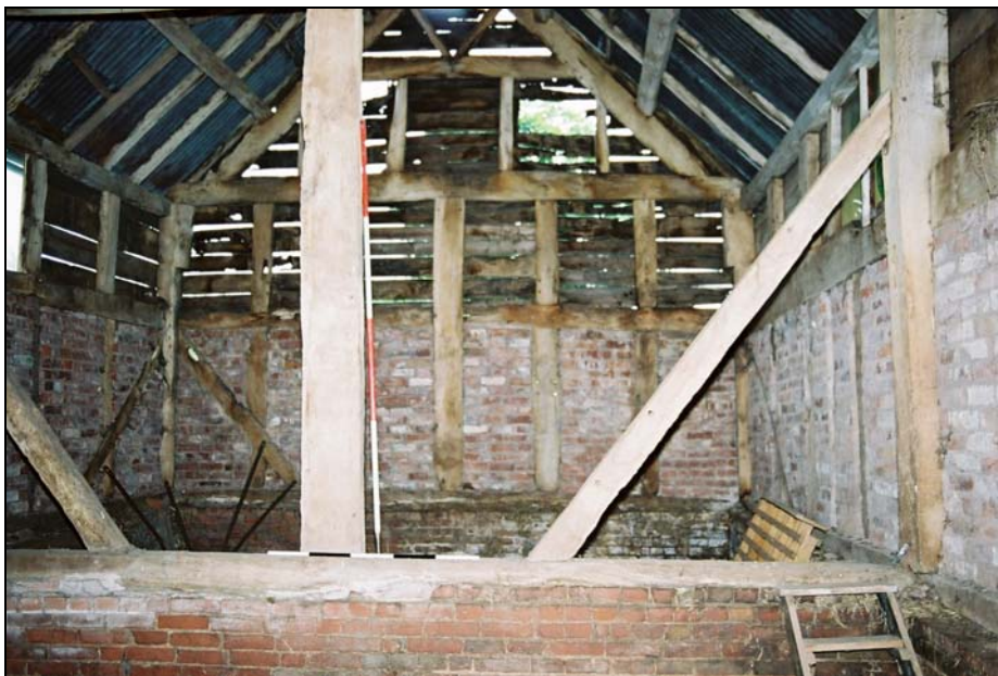
View along the barn to the east showing Truss 5 and Truss T6
