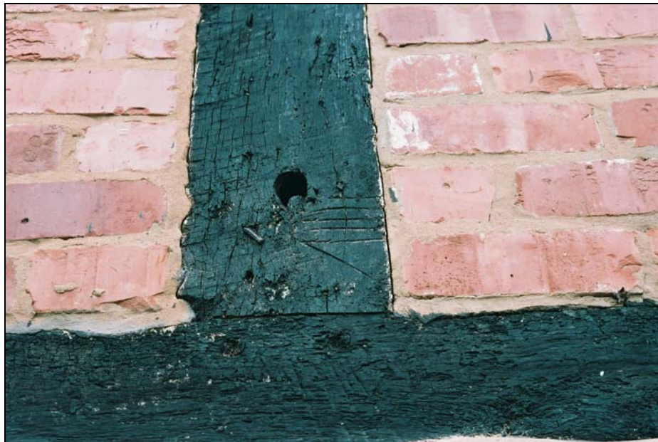
Scribed carpenter's marks on a rail on north elevation of the barn
