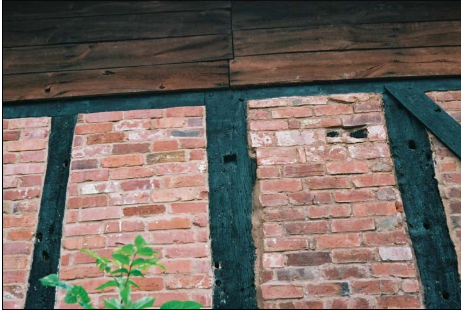
Detail of frame showing a 'scotch' (notch in post for a supporting strut during the construction process). The diagonal strut (right) is clearly false and is nailed onto the frame
