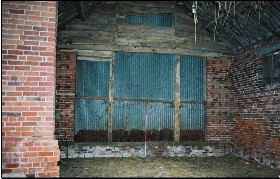
The western gable of Building 8 showing reused brickwork and timber sill beam (scale 2 metres)
