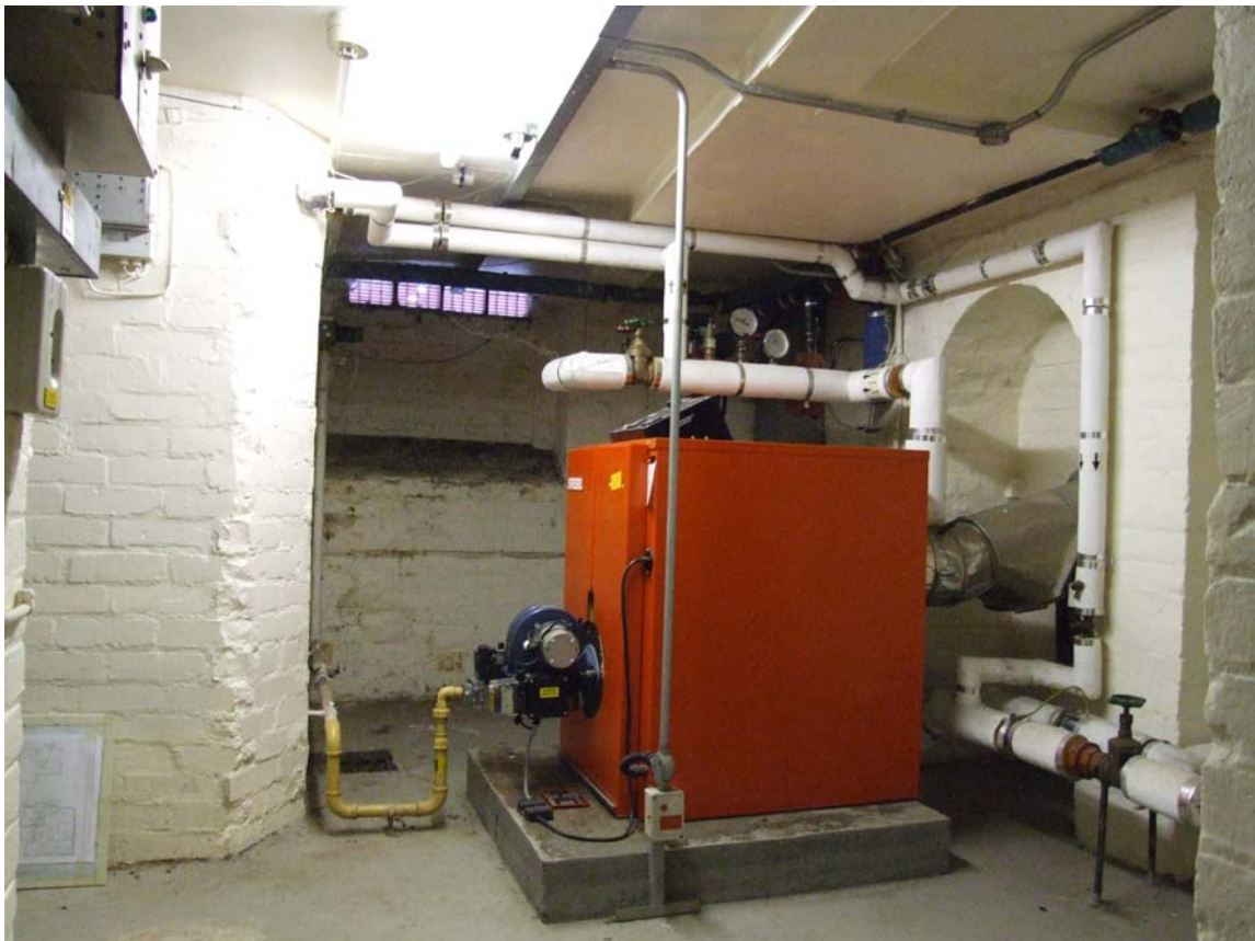
Plate 16: The boiler room in the cellar
