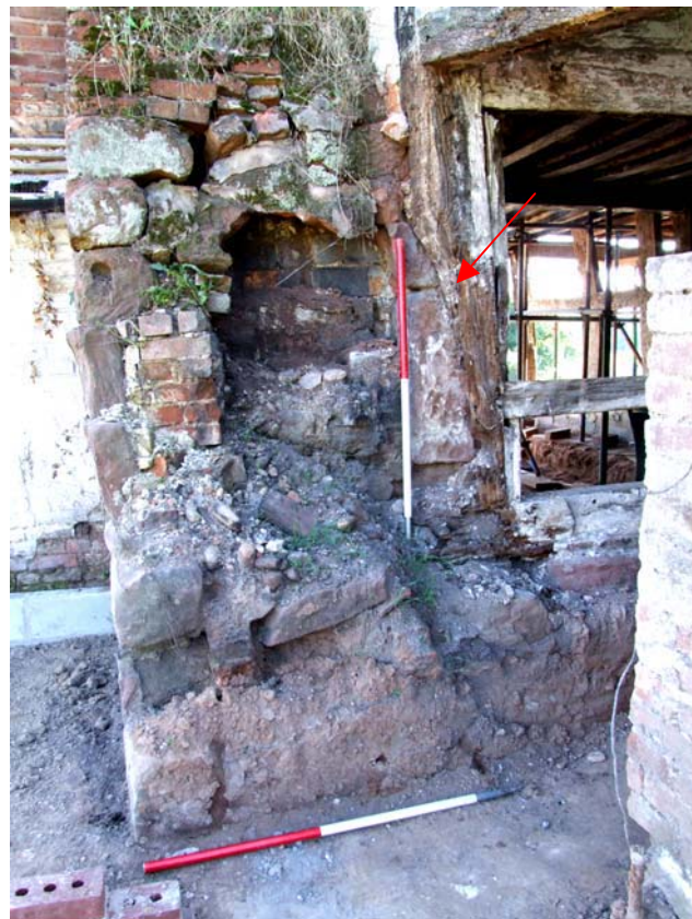
Plate 14: North-east corner post trimmed down to accept bread oven fabric (scales 1-metre)
