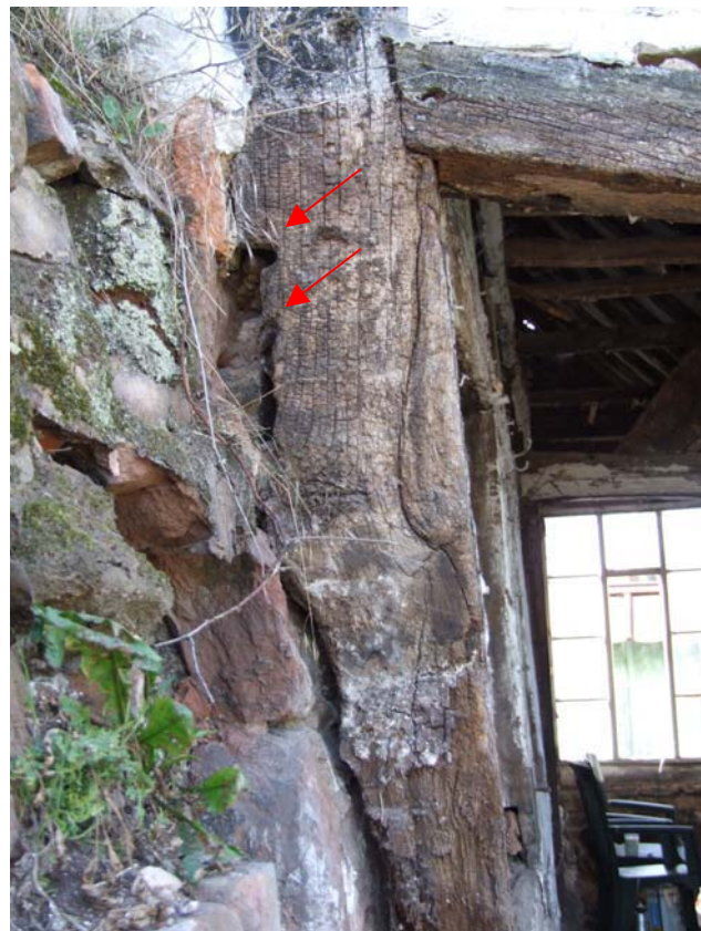
Plate 12: Empty peg-holes in north-east corner post, for rail removed when chimneystack constructed
