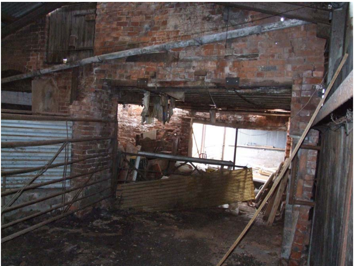
Plate 16: Stub walls of former south range (now demolished) at their juncture with the eastern range
