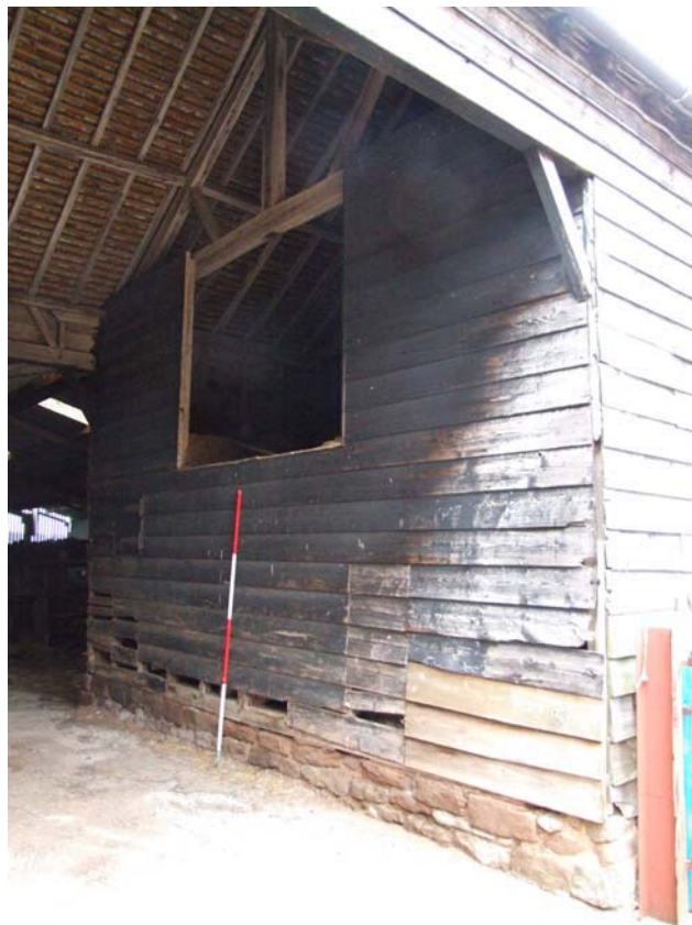
Plate 8: Timber clad extension at the southern end of the western range (scale 2-metres)
