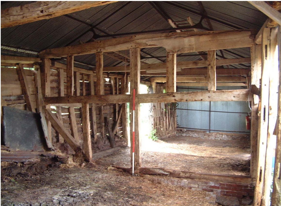
Plate 3: View to the south inside the barn, showing the levelled up bay 2 (centre of photo) and the floor slope to the south-west
