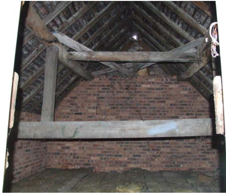
Plate 7: Inserted frame to bay 1 to support purlins. Also note the apex of truss T1 in the gable end
