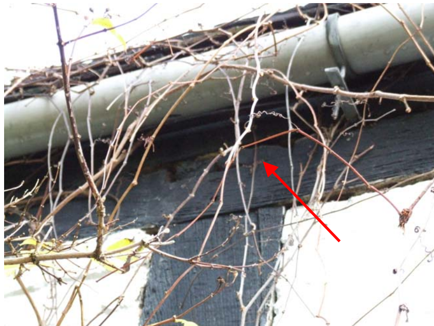
Plate 5: Rebate in wall plate for lap joint to a truss, which has now gone
