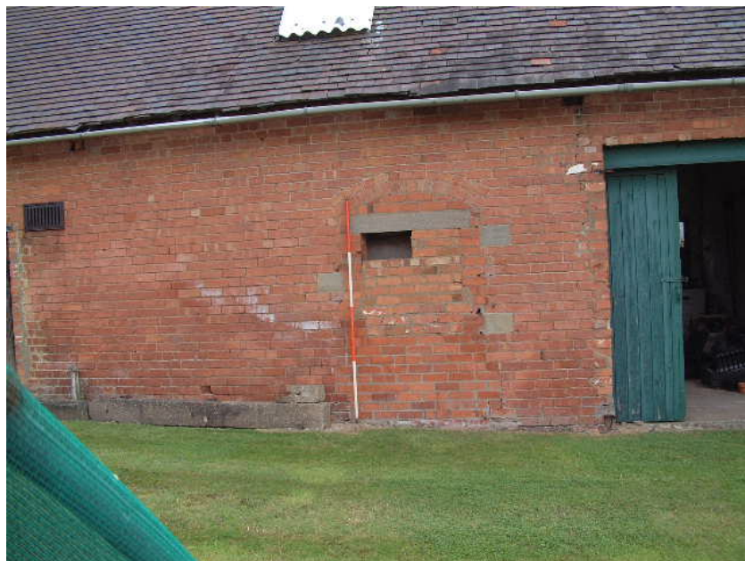
Blocked stable door in Space B of Building 4 (scale 2 metres)
