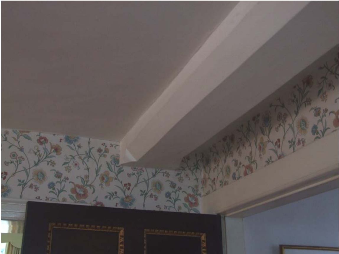
Plate 7: Chamfered and stopped bridging beam in the 17 th century wing, first floor
