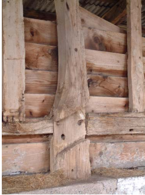
Re-used tie-beam section from a cruck-framed building within the fabric of the barn
