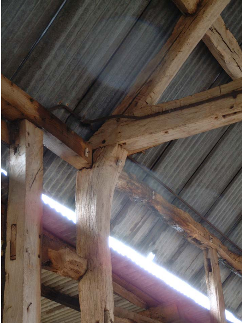
Jowelled post of Frame /Truss T: note the carpenters' marks (III) on the tie beam and principal; the empty mortises on the underside of the tie beam and inner post, indicating removed framing. Note also, the 'newer' framing of bay 1 to the left of the post.
