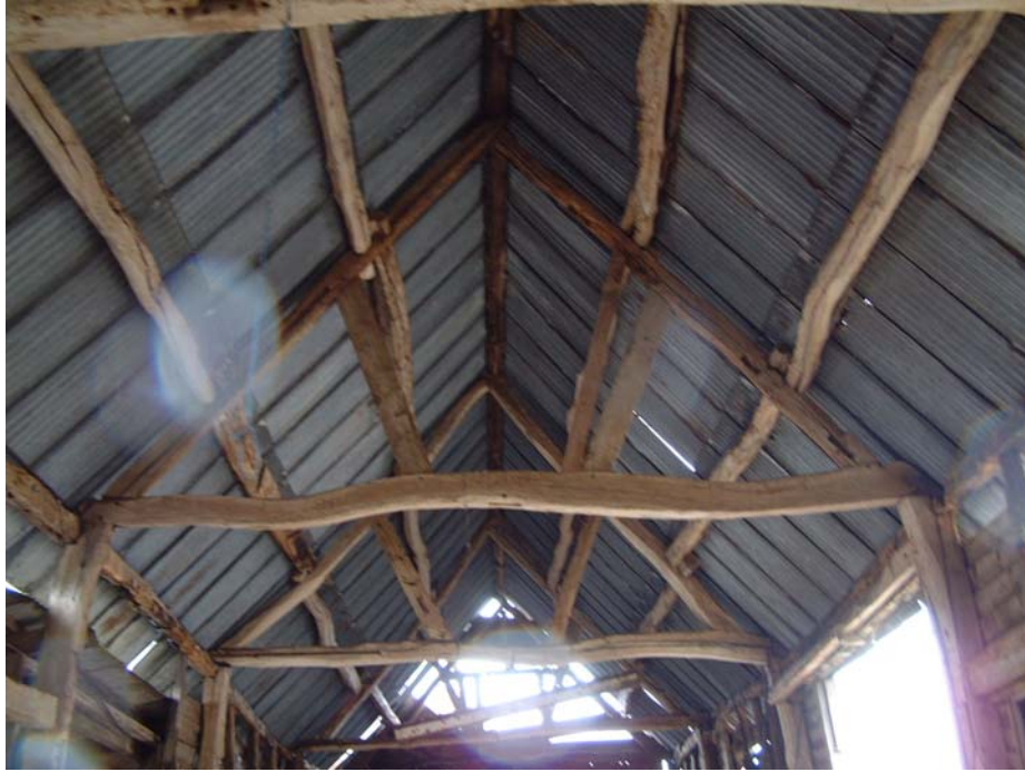
Trusses T3, 4 & 5, note the waney timbers and compare with truss T1 and T2 (plates 4& 5)
