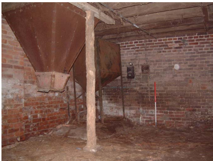
Hoppers on the ground floor of the fodder processing shop (scale 1 metre)
