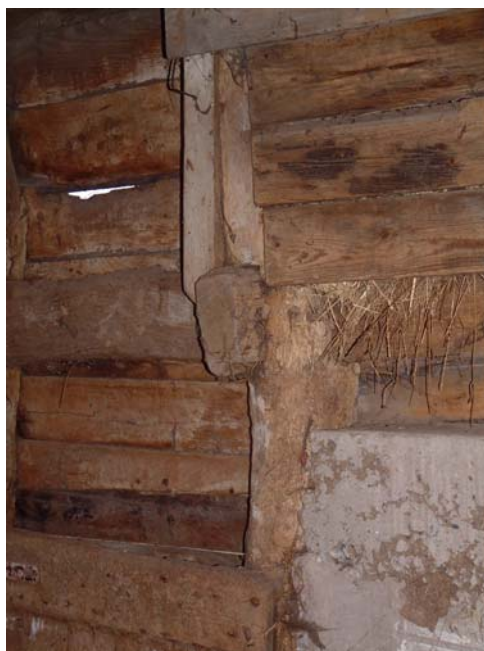
Sawn off rail on the corner post of T5, indicating this was once an external frame
