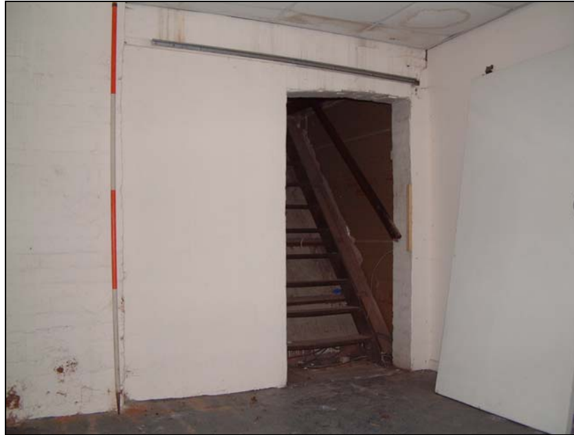
Staircase to first floor of the three-storey mill building. Note the central dividing wall has cut the arched lintel. This was originally an opening from one bay to another (Scale 2 metres)
