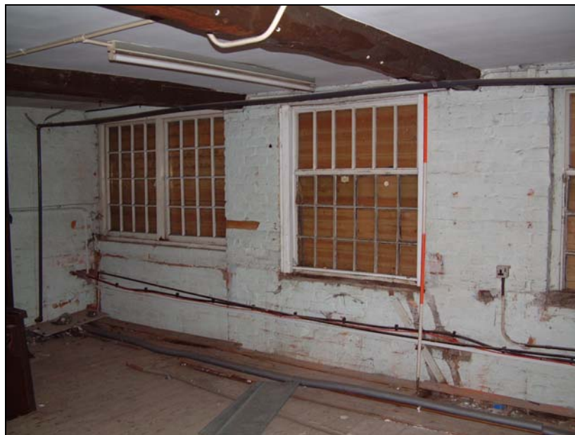
First floor of the three-storey section showing the former location of loading doors on the right, replaced by a later window (Scale 2 metres)
