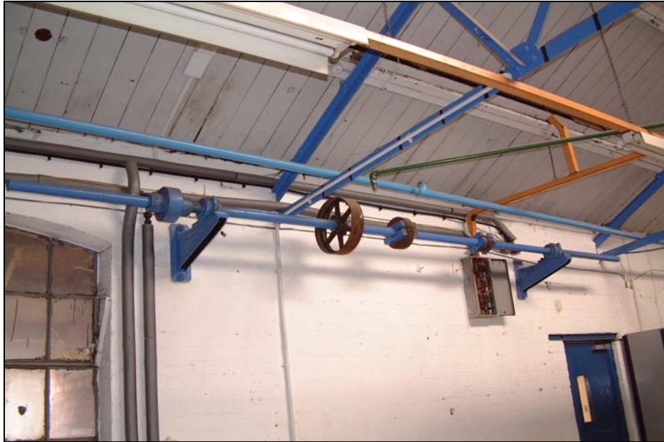
Flywheels and shaft of part of the factory power train in the northern building.
