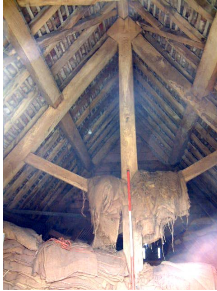
Kingpost truss above storage room at the northern end of the barn (red on scale is 0.50 metres)
