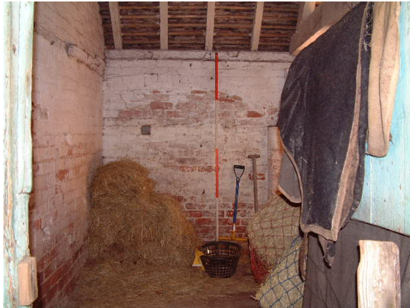
Blocked entrance inside the tack room (Scale 2 metres)
