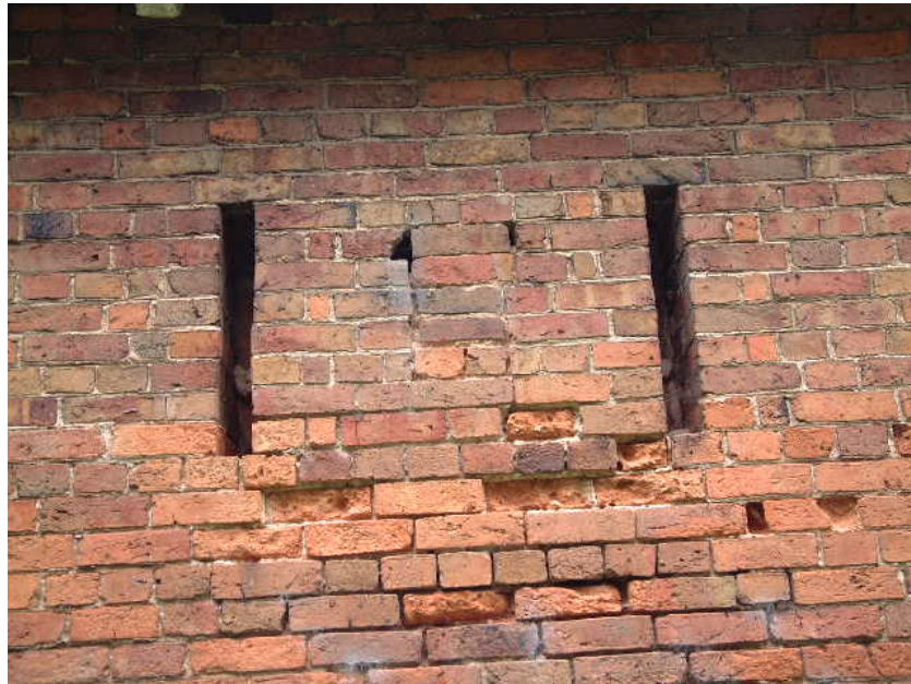
Inserted bricks where the support beam for the new upper floor at the north end has been inserted
