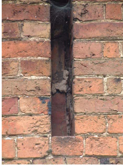
Slit vent blocked when the new floor was inserted at the northern end of the barn
