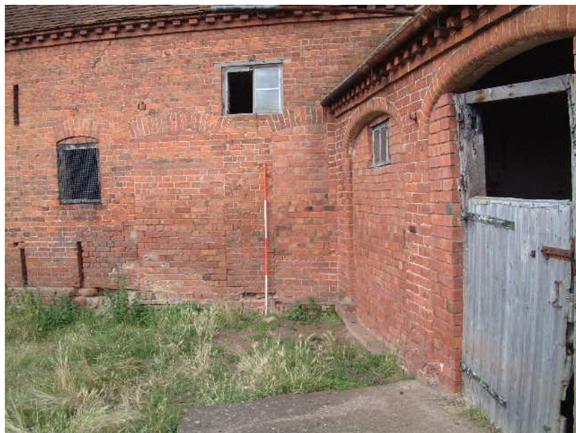
Blocked up doorways in barn eastern elevation showing that the stable block is later (Scale 2 metres)
