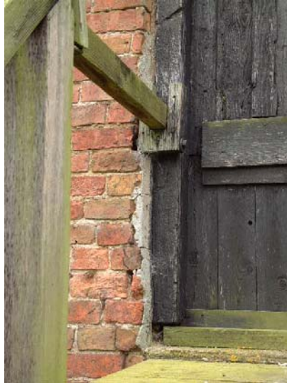
Brickwork cut away at the bottom of former pitching eye, to form new doorway
