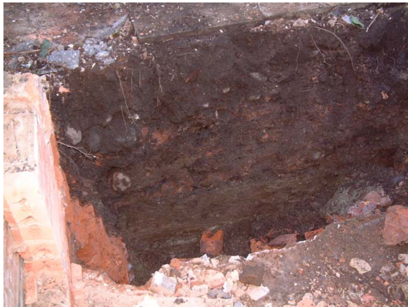
North-west facing section in the foundation trench for the new build (See Figure 5)
